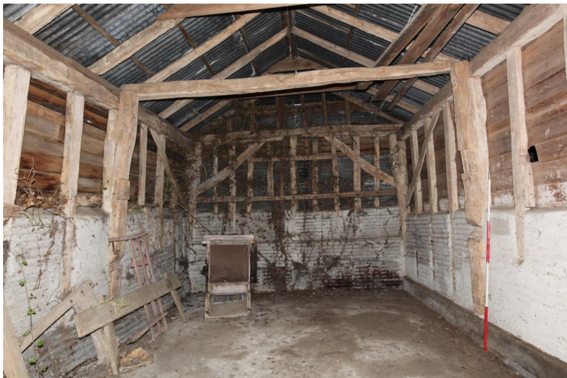
Illus. 8 The open truss of the early-17 th century bays A and B from the south, which originally contained a loft supported by a binding joist spanning the width of the storey posts. The tie-beam is a later replacement but the posts also contain mortises for the down-braces of a partition above the binding joist (presumably with a central door).
