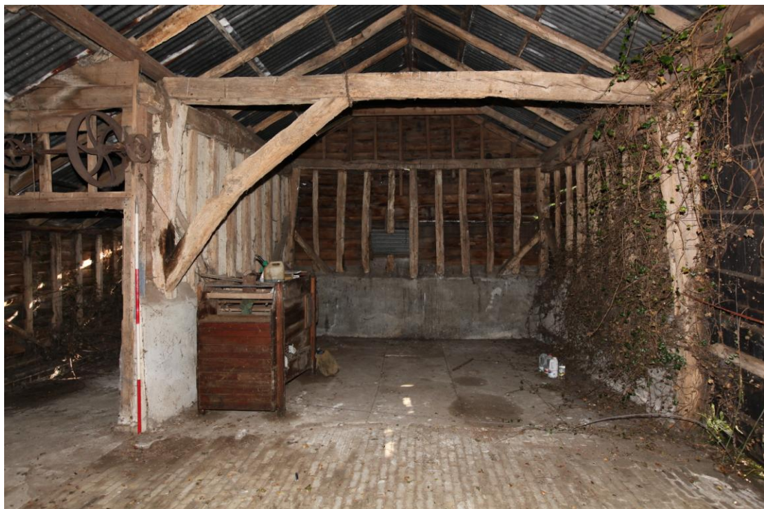
Illus. 6 The open truss to the south of the threshing bay (C) showing the well preserved gault brick threshing floor in the foreground and the 20 th century rear lean-to (E) to the right. This truss is integral to the 18 th or early-19 th century southern bay and consists of re-used timber. The primary diagonal braces of the southern gable, which also consists of re-used timber, are visible in the rear.
