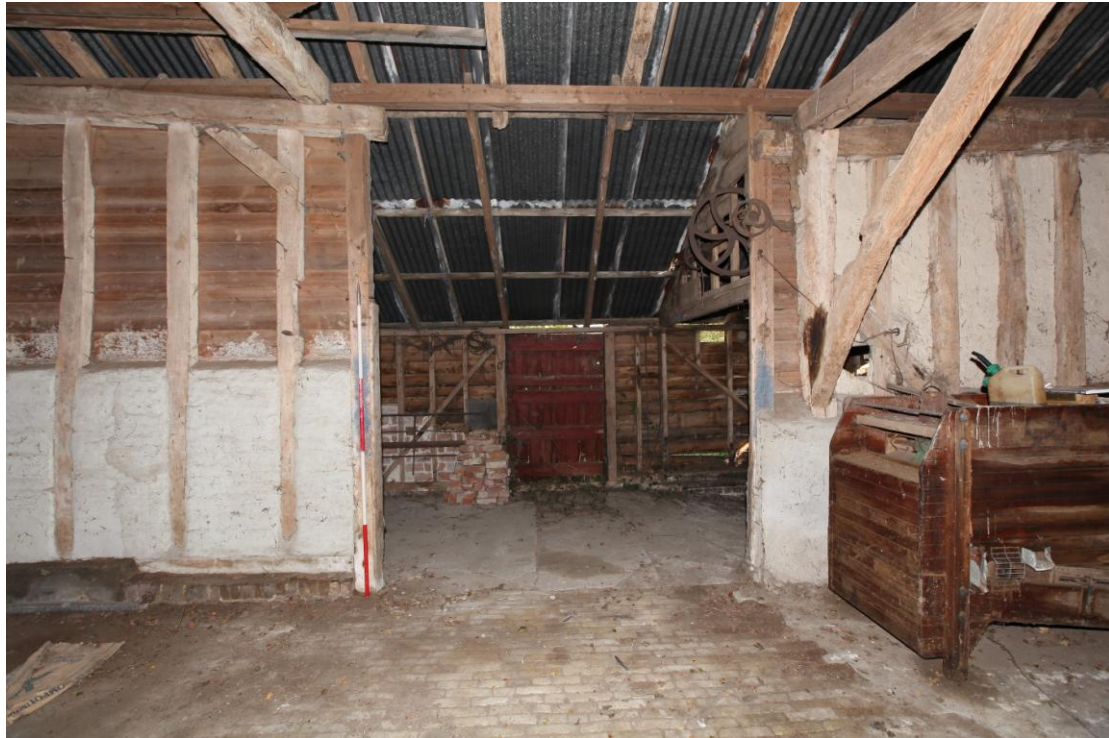
Illus. 7 The eastern interior of the threshing bay (C) showing the access to the rear lean-to (E) and the lack of storey post to the truncated late-16 th or early-17 th century framing of bays A and B to the left.
