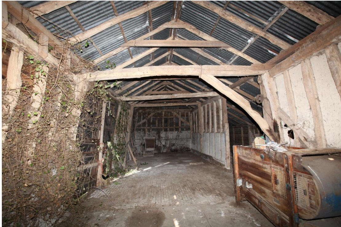
Illus. 5 A general view of the interior from the south showing the intact arch-brace to the tie-beam between bays C and D to the right, with the early-20 th century grain sifter to the extreme right.
