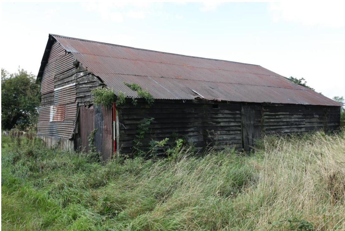
Illus. 2 The exterior from the south-east showing the shallow-pitched 20 th century corrugated iron roof and cladding with the rear doors of the threshing bay (C) in the weatherboarded 20th century lean-to (E) to the right.
