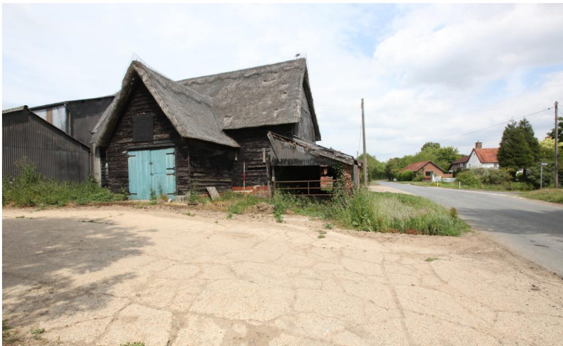
Illus. 2 The exterior of the thatched barn (1) from the west showing its 19 th century gabled porch and southern lean-to shed. The grade II-listed 16 th century farmhouse is visible on the opposite side of the Woodbridge Road to the right.
