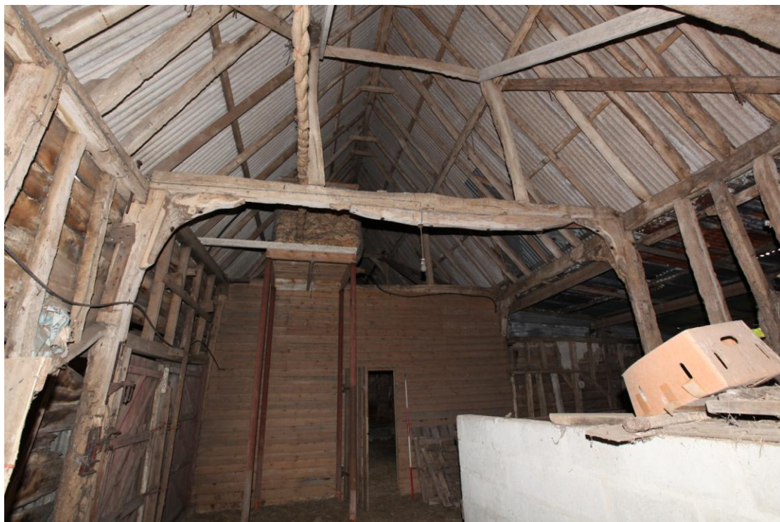
Illus. 8 Middle barn (2). The interior from the east showing the intact queen-post roof structure, which is less visible than that of the thatched barn due to the presence of the 20 th century boarded partition visible here and a wire-mesh hay loft in the two western bays (2A and 2B). The tie-beam in the foreground contains the empty stud mortises of an original partition which divided a three-bay threshing barn to the west from a two-bay stable and loft to the east.
