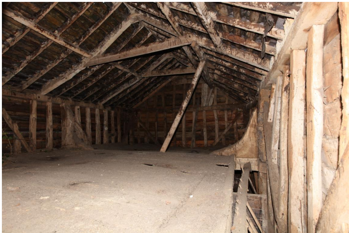
Illus. 14 Stable (4). The interior of the hay loft from the south showing the butt-purlin roof structure with re-used timber and the hay drop above the rack to the right.
