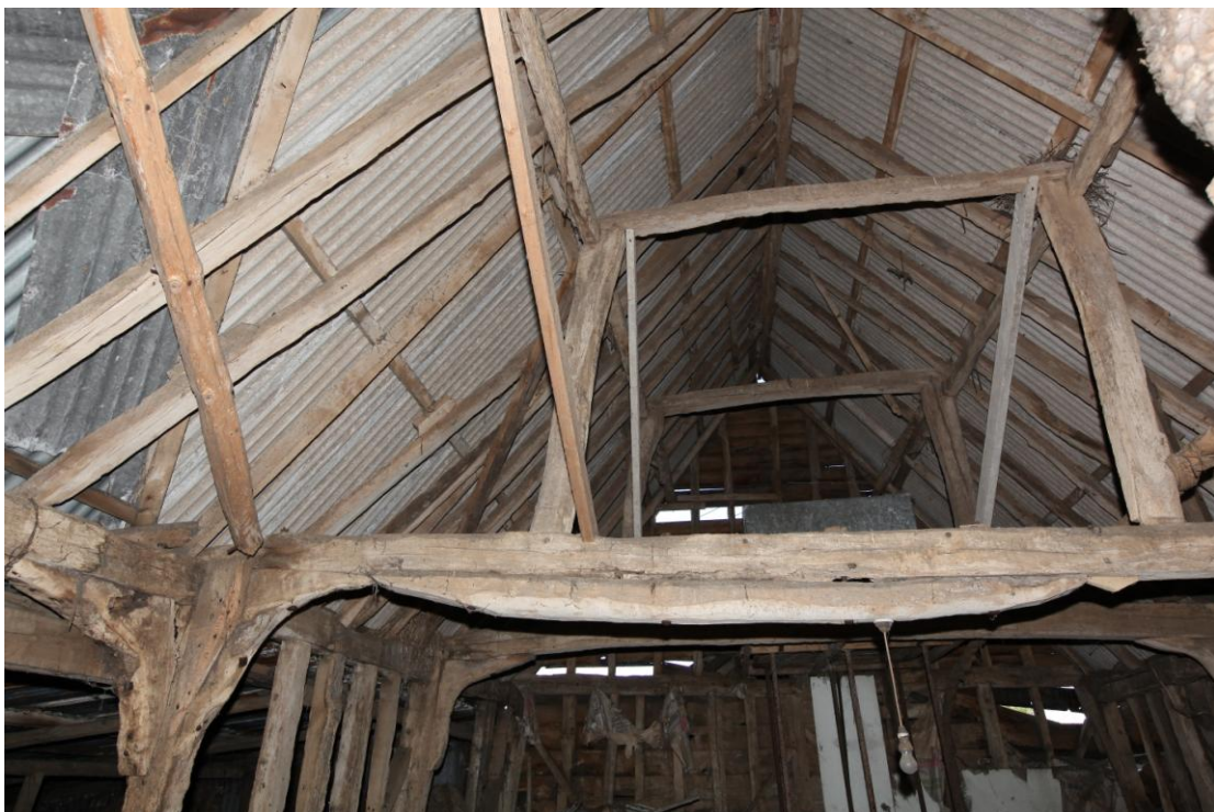
Illus. 10 Middle barn (2). The roof trusses of the eastern bays which lack braces to either the purlins or collars. There is evidence of a half-hip at the eastern gable but (like that of the thatched barn) it was converted into a vertical gable in the 19 th century.
