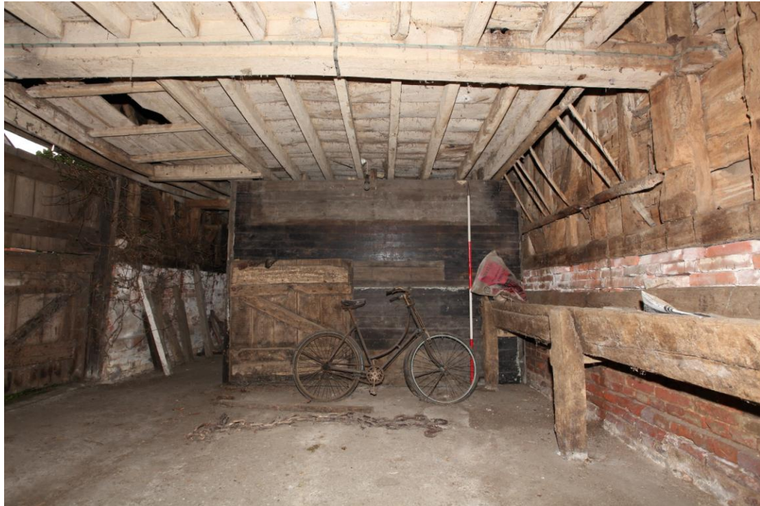
Illus. 13 Stable (4). The southern section of the interior from the southern gable, showing the intact 19 th century boarded manger and hay rack beneath a hay drop in the loft ceiling to the right. The manger continues into the northern section beyond the boarded partition.
