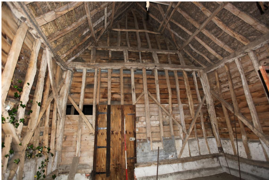
Illus. 6 Thatched barn (1). The interior of the northern gable showing the 19 th century studwork with nailed primary braces. The short studs between the upper tie-beam of the half-hip are original, as are the diagonal hip rafters and purlins. This bay was built as a stable entered by a door against the corner post to the right and evidence is visible here of three diamond-mullion windows to its loft (to the extreme left and right, and in the centre of the tie-beam).
