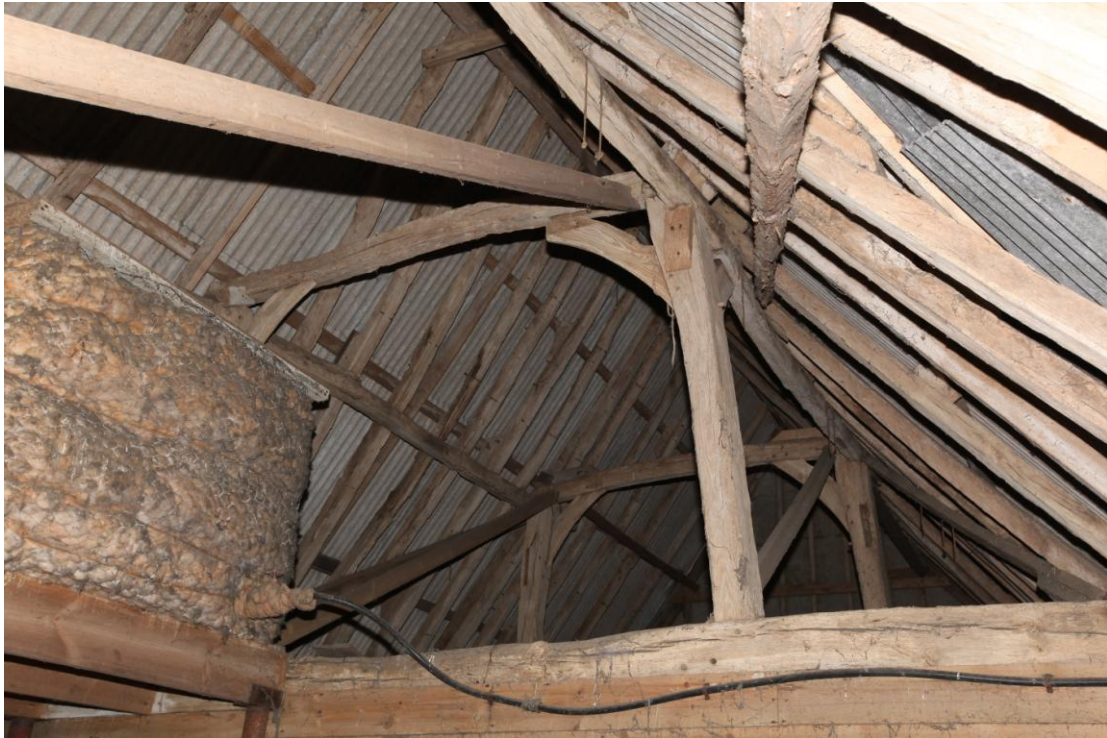
Illus. 9 Middle barn (2). The queen-post roof above the two eastern bays, seen from the east (but hidden from beneath by a wire-mesh loft). Like the thatched barn, only the threshing bay (2B) was provided with braces, of which three have been lost.
