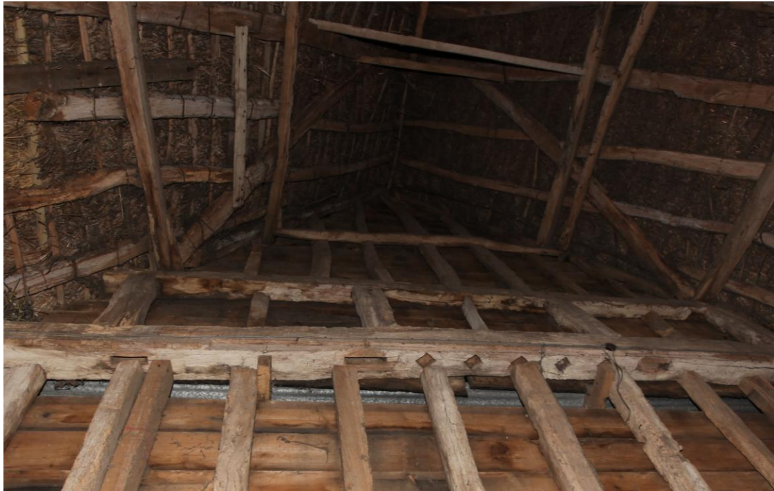
Illus. 7 Thatched barn (1). Detail of the underside of the northern gable tie-beam showing a series of empty mortises for studs and the diamond-mullions of a central six-light window with sliding shutters on both sides. The hip collar at the top of this image contains three peg holes for original rafters.
