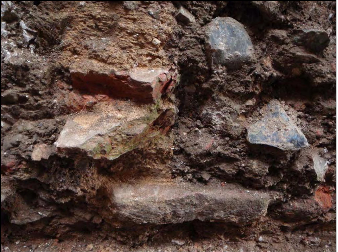
Plate 3. Western half of structure 0007, showing vertical wall stub going down to horizontal base
