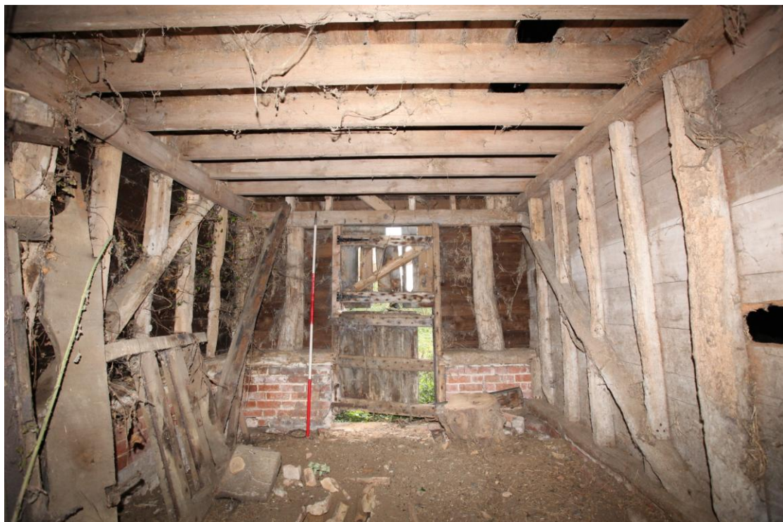
Illus. 12. The southern interior of the stable (1b) showing its ostensibly original entrance doorway respected by a closer brick in the plinth to its right. The joists of the loft are of tall-sectioned softwood and may be secondary but the studwork of the partition adjoining the main barn (1a) to the right is identical to that of the external walls and appears to be original.
