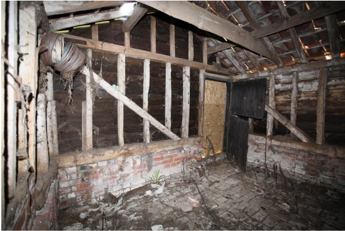
Illus. 7. The southern internal gable of the enclosed yard shed (1e) showing its original gault brick floor and the half-hung entrance door at its western end to the right.
