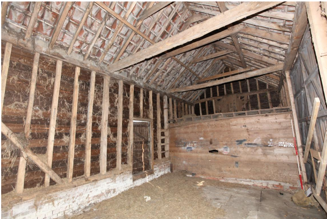
Illus. 8. The interior of the main barn (1a) from the south-west showing its narrow wall studs interrupted by nailed diagonal primary braces incorporating much softwood and re-used timber. The original softwood clasped-purlin roof structure incorporates a ridge board and its collars are nailed to the principal rafters (all typical of the second half of the 19 th century). A nailed loft ladder flanks the small rear door to the left, and the deal boards of the ostensibly original stable partition (with an open loft above) display a variety of unusual graffiti.
