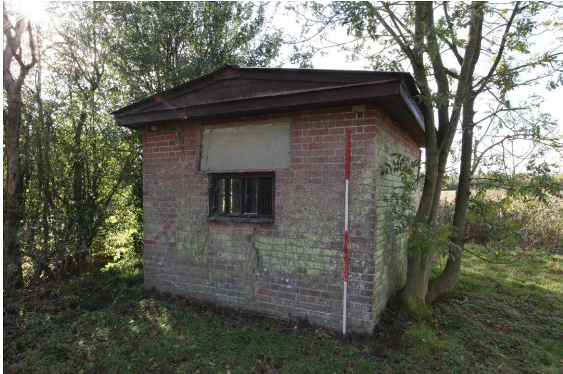
Illus. 13. The eastern external gable of Absalom Feavearyear's mausoleum (4) showing the 16th century style window with pegged roll-moulded mullions and the inscribed stone plaque above. The self-seeded ash tree beneath the foundation to the right is causing severe structural damage and the building is collapsing into the deep enclosure ditch to the left.
