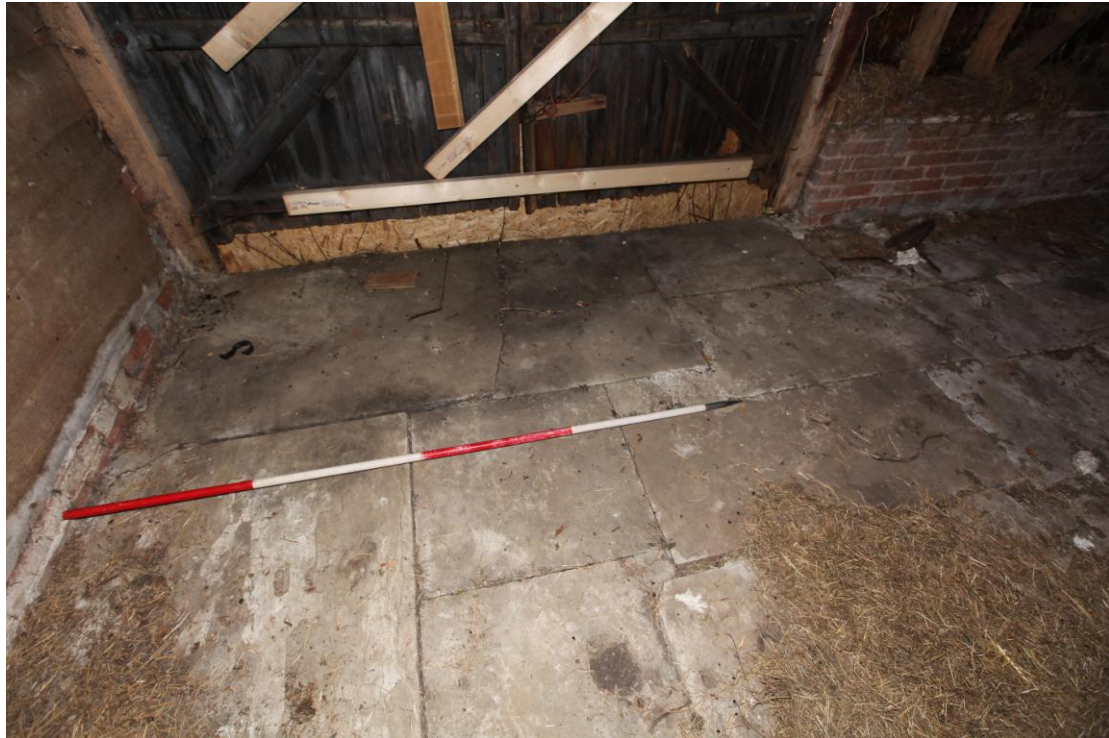
Illus. 9. A detail from the north of the exceptionally large stone flags forming the entire floor of the main barn (1a), showing the southern entrance doors in the rear. The stones may represent the unused stock of the carpenter and stonemason Absalom Feavearyear.
