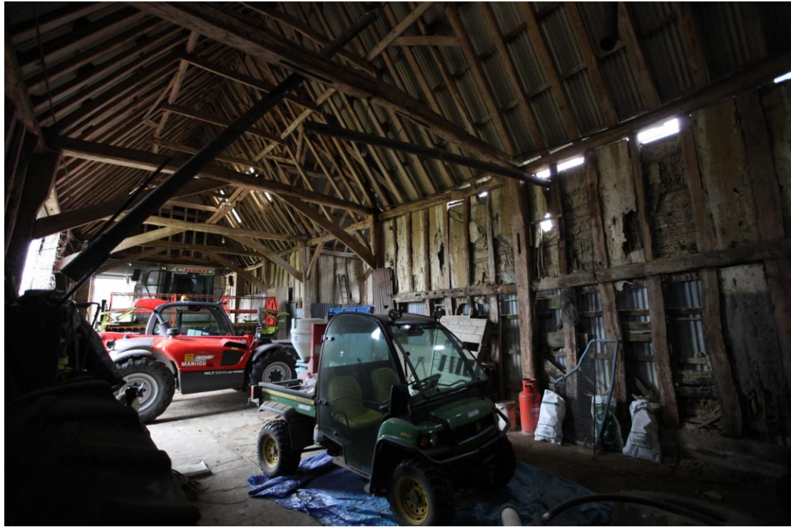
Illus. 5. General internal view of barn from north-western corner (bay A) showing its largely intact timber frame and current use as a garage for farm vehicles.
