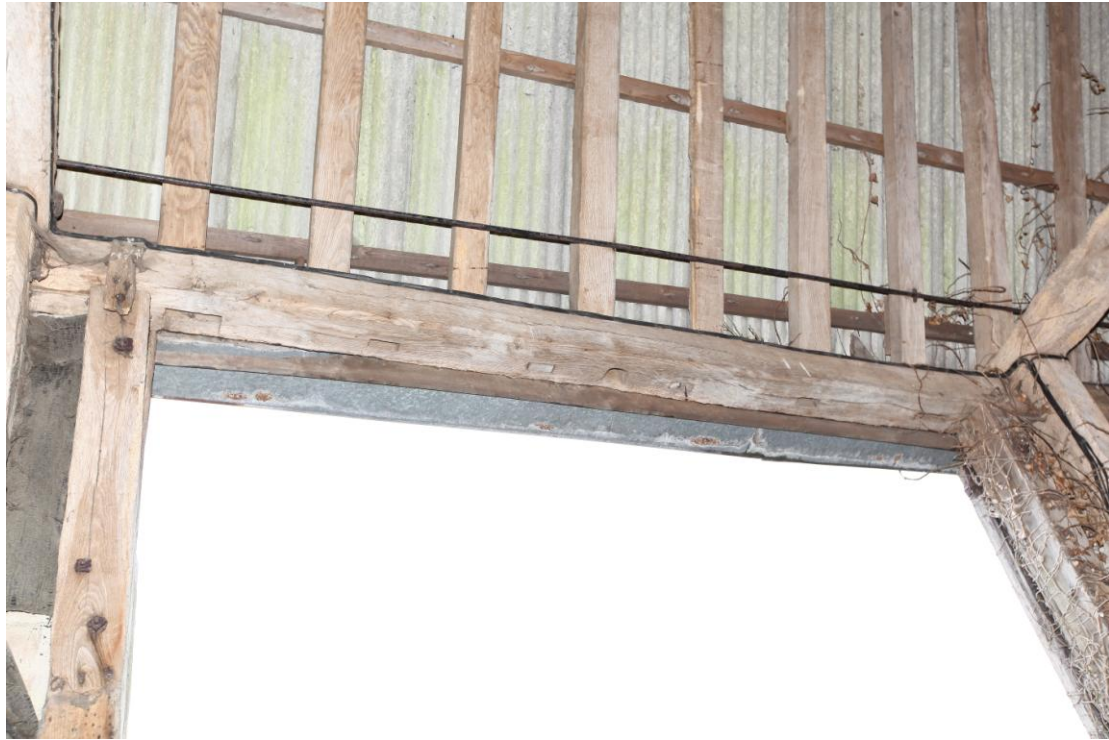
Illus. 7. Detail of the northern roof-plate above the current entrance in bay C showing the unusual arrangement of alternately pegged and unpegged stud mortises with a central housing for a door bar. The large outer mortises inside the present nailed jambs appear to have secured the original door posts.
