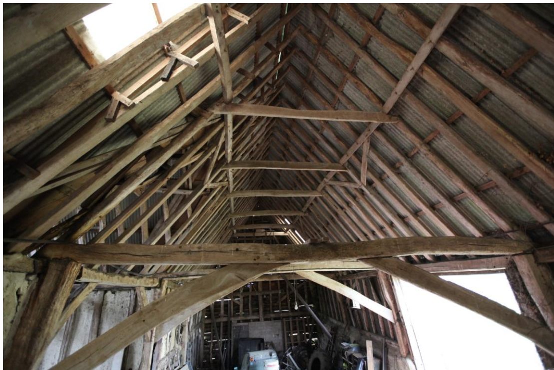
Illus. 12. The clasped-purlin roof structure of the western bays seen from the east, showing its fully intact wind braces and the open truss adjoining the entrance bay (C) in the foreground.
