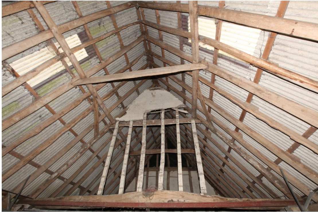
Illus. 11. The roof structure of the eastern bays seen from the west, showing the remains of a later partition which divided the eastern bay (F) from the rest of the interior (probably to form a stable). The pegged mortises of the original arch-braces are visible in the tie-beam.
