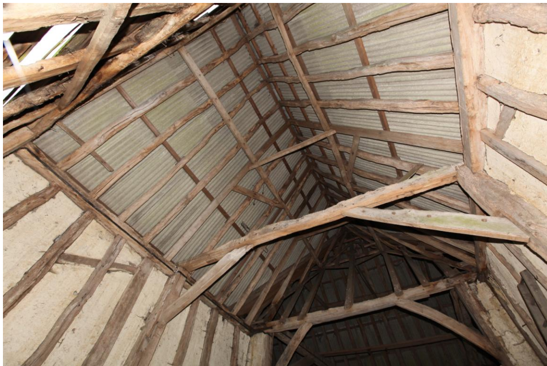
Illus. 8. Roof of porch (1a) from the south, showing its intact wind braces and arch-braced open truss with empty mortises in the underside of its re-used tie-beam. The braces of the southern roof-plate in bay C (visible in the rear) are also original.
