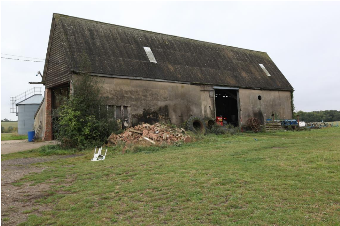
Illus. 2. Exterior from north-east showing corrugated asbestos roof (replacing thatch) and cement render to walls, with 20th century vehicle entrance in eastern gable to left and original entrance in bay C to right.
