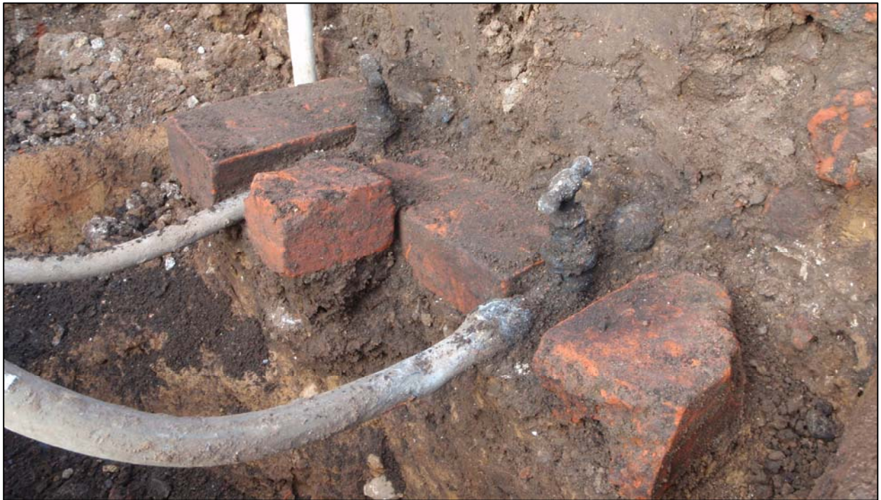
Plate 16 stopcocks (0084) at the front of houses 2 and 3 (ref. HLP 85)
