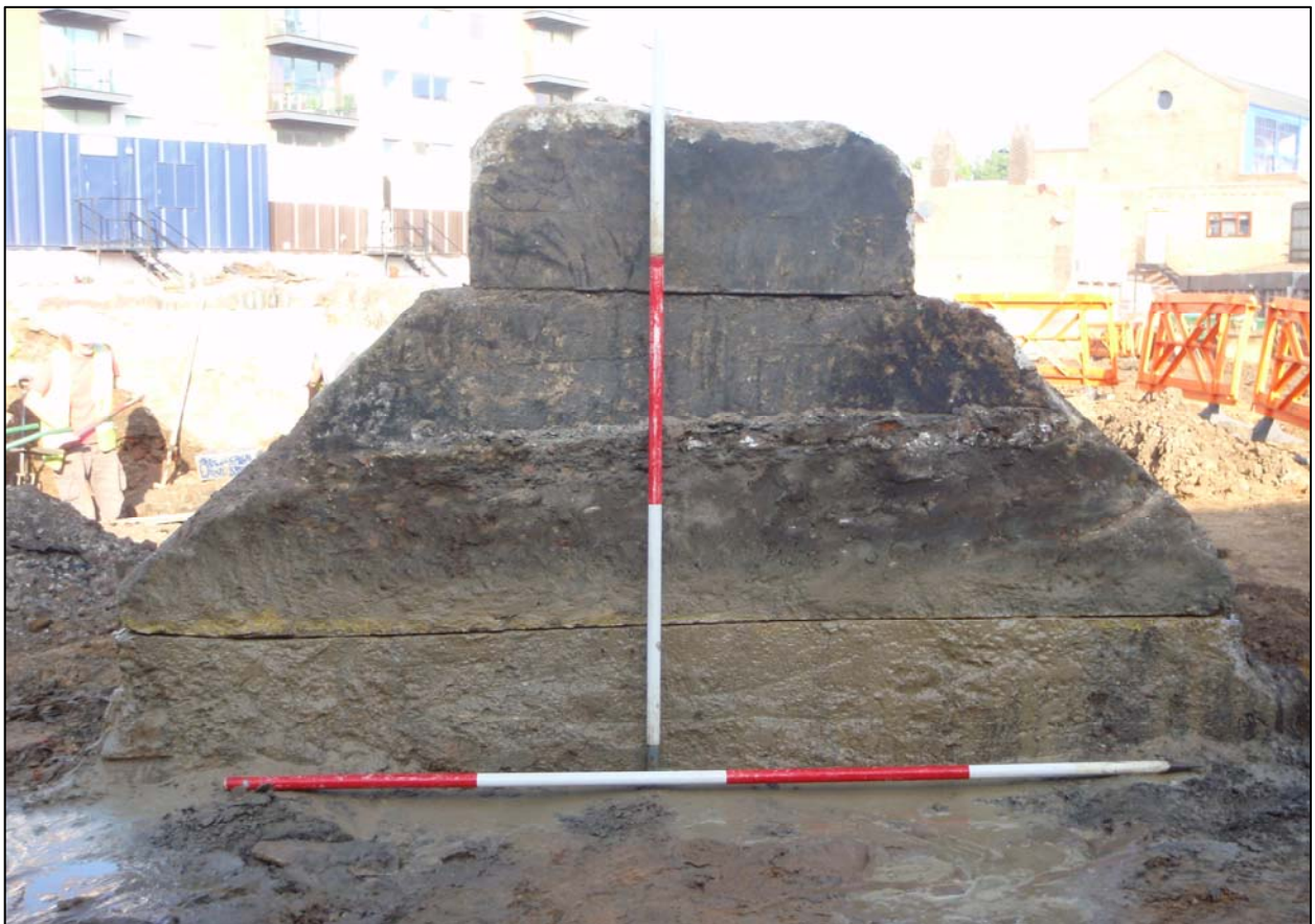
Plate 47 Shelter 6, south-east face with escape hatch shaft (N.B. the concrete has been cut with a disc-cutter in preparation for demolition) (ref. HLR 03)
