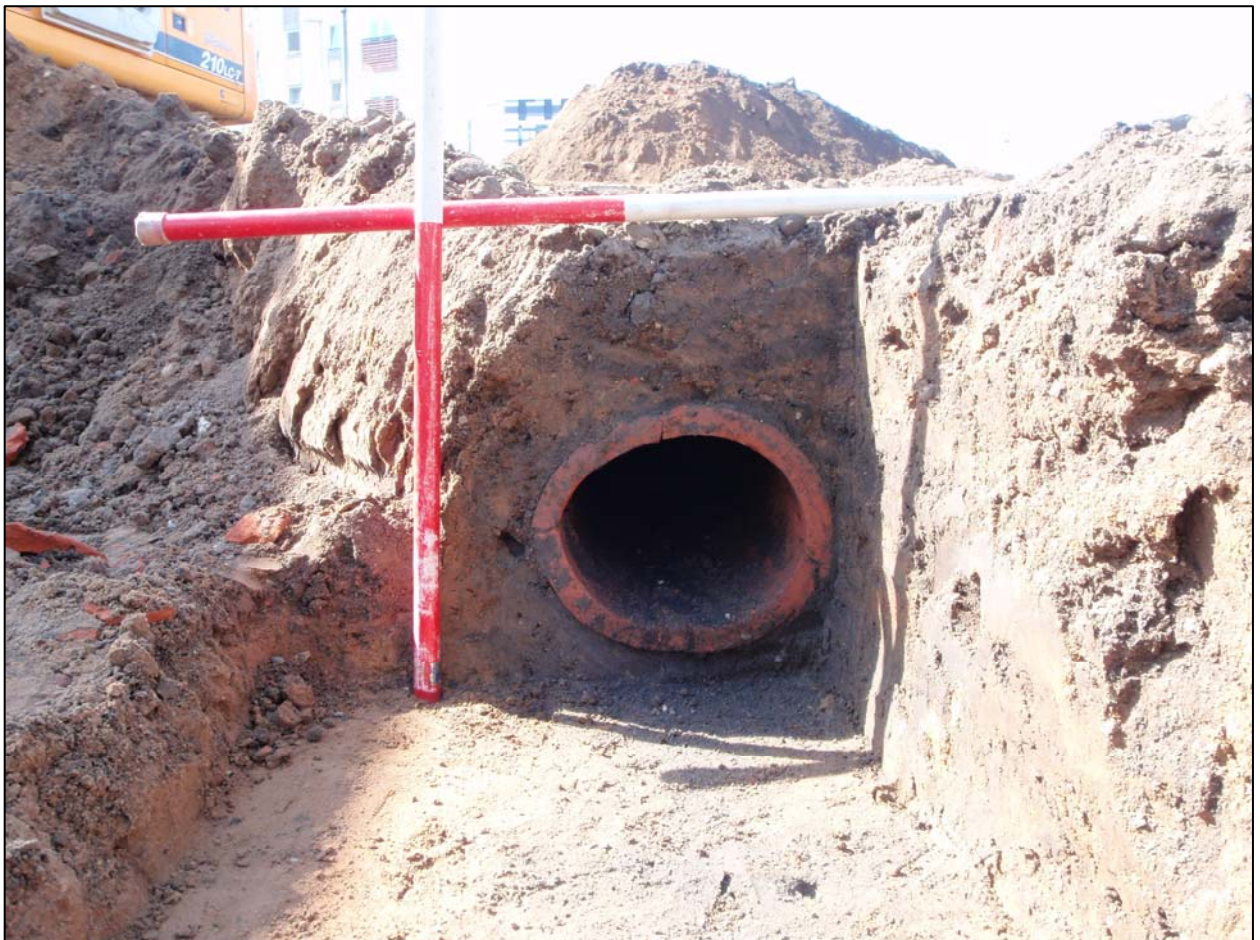
Plate 5 surface water drain running below roadway (ref. HLP 48)
