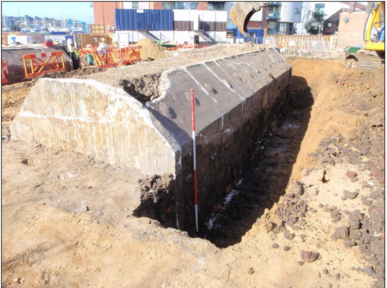
Plate 43 Shelter 5, after exposure of north-east side, just prior to demolition (ref. HLQ 92)
