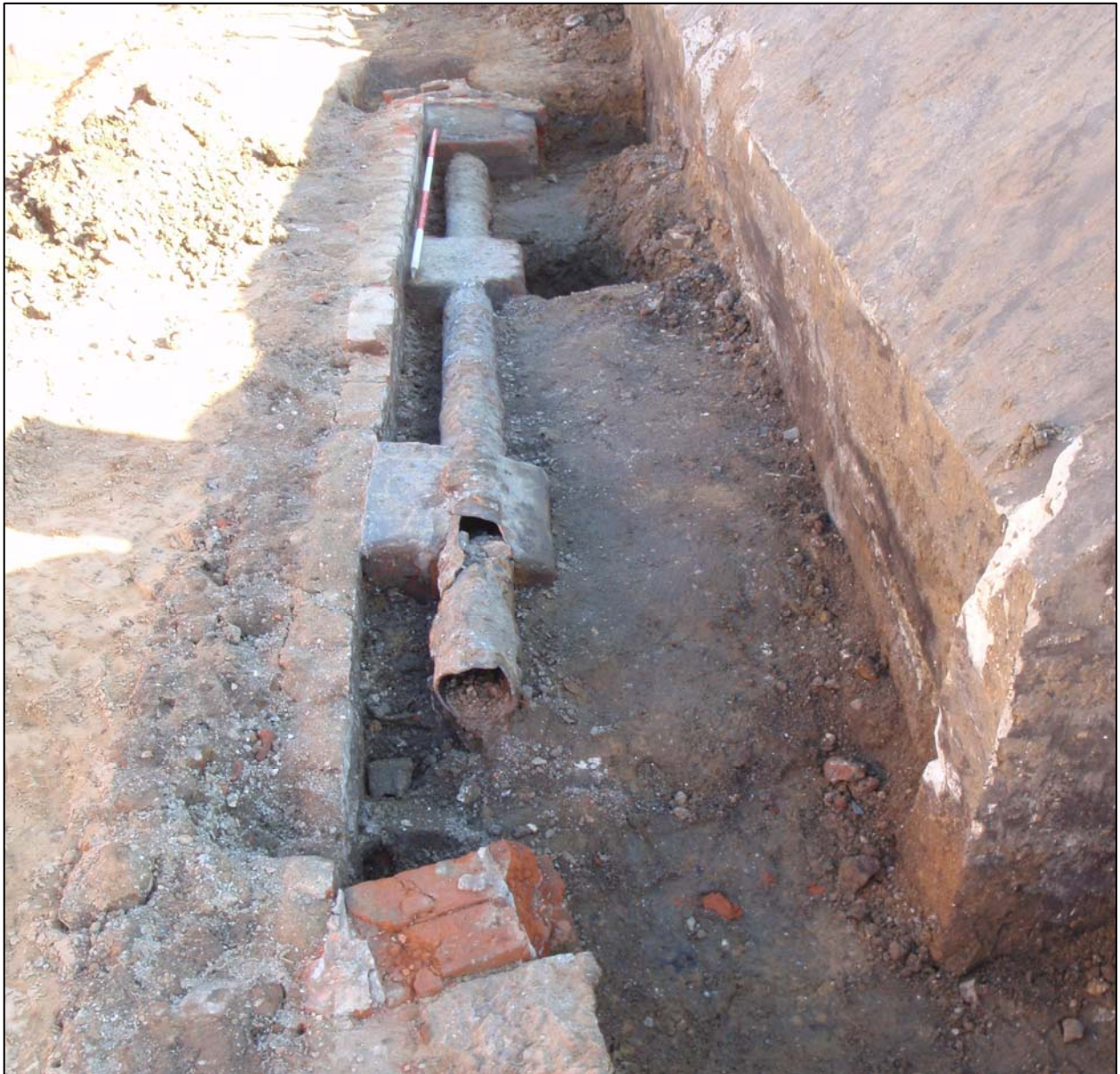
Plate 21 cast iron drain pipe (0096) as seen in house 3 cellar (ref. HLP 93)
