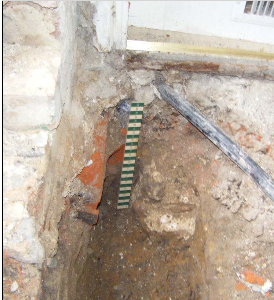
Plate 1. Flint and mortar foundation for a sill beam sitting on natural at the north end of the footing trench.
