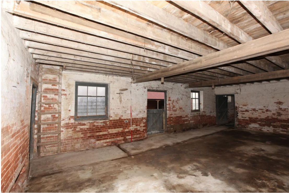
Illus. 9. The southern interior of the eastern stable (D) showing its central yard door flanked by windows with an original vertical loft ladder to the left.
