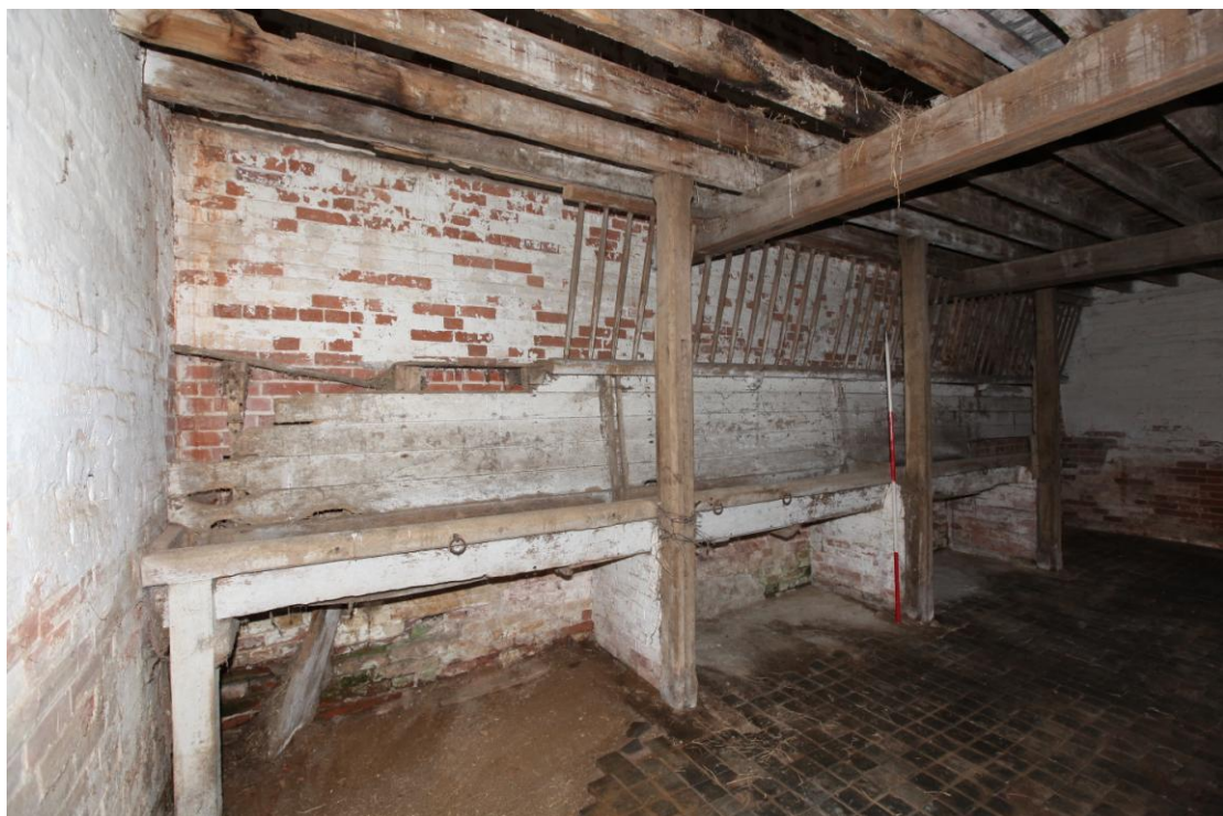
Illus. 12. The manger & hay rack to the rear of the western stable (B) showing three bolted vertical posts with vertical grooves for missing stall partitions.
