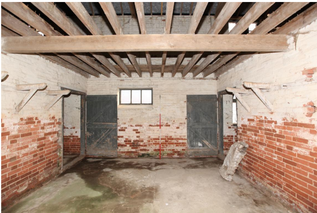
Illus. 10. The southern interior of the central tack room (C) showing the original wooden harness hooks and the doors to the eastern and western stables (D and B) to the left & right respectively.
