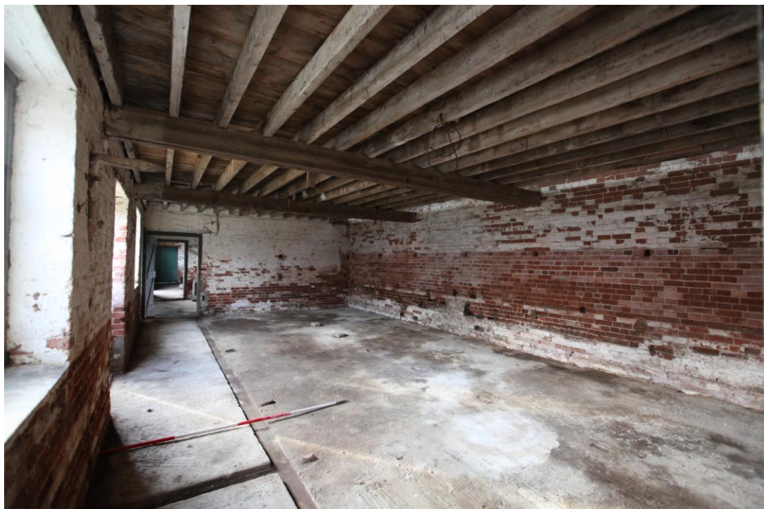
Illus. 8. The interior of the eastern stable (D) from the north-east showing the position of the removed hay rack & manger beneath the hay drop against the rear wall to the right and the axial passage to the left. The concrete floor is a 20 th century replacement.
