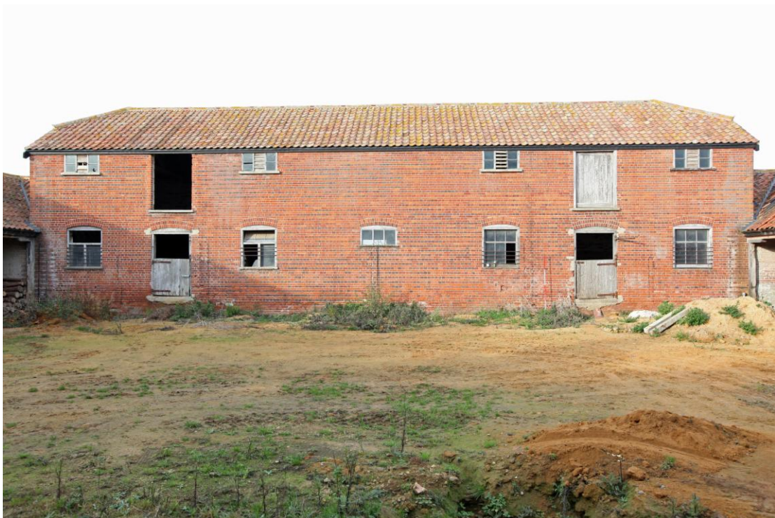
Illus. 4. The southern facade of the stable range from the yard. This elevation is largely original apart from the first-floor loading doors to the hay loft which are secondary insertions interrupting the pattern of brickwork.
