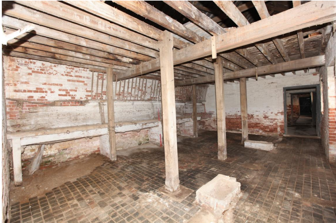
Illus. 11. The interior of the well preserved western stable (B) from the south-west showing the original hay rack and manger to the left with the nailed posts of ostensibly secondary stall divisions (from which the boarded partitions have been removed). The tiled floor appears to be original.
