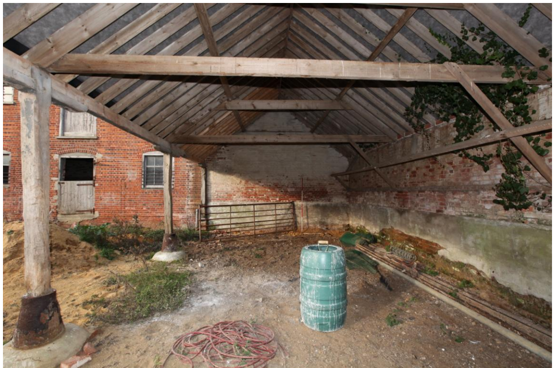
Illus. 6. The interior of the eastern shelter-shed (G) from the south, showing its softwood clapped-purlin roof structure and the remains of a 20th century hay rack to the right. The chamfered arcade posts and lintels to the left retain their original iron conical bases.
