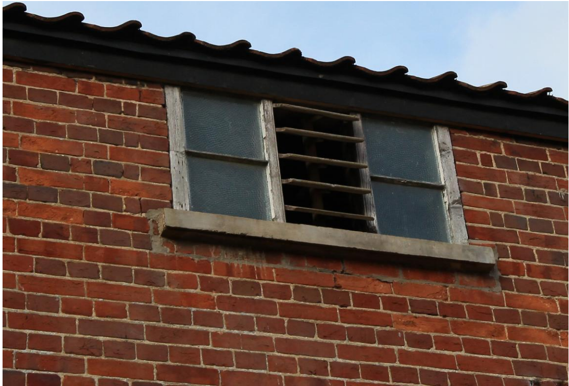
Illus. 5. Detail of one of the unusual loft windows in the southern exterior showing its original central louver operated by a vertical spindle. The sill is a replacement.
