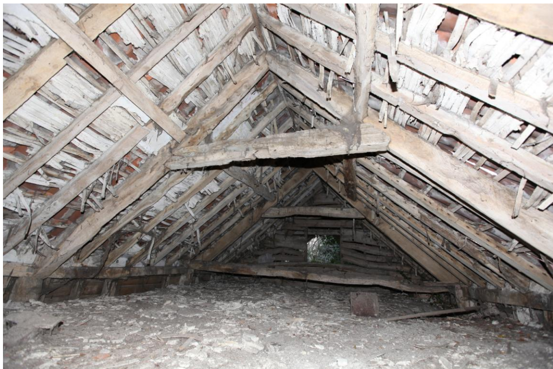
Illus. 12. The butt-purlin roof structure of the hay loft over the stable (1a) seen from the northern gable. The lath-and-plaster beneath the pantiles appears to be original but many timbers show evidence of re-use from older buildings. The hatch in the rear is an internal feature which opens onto the loft of the tack room (1b).
