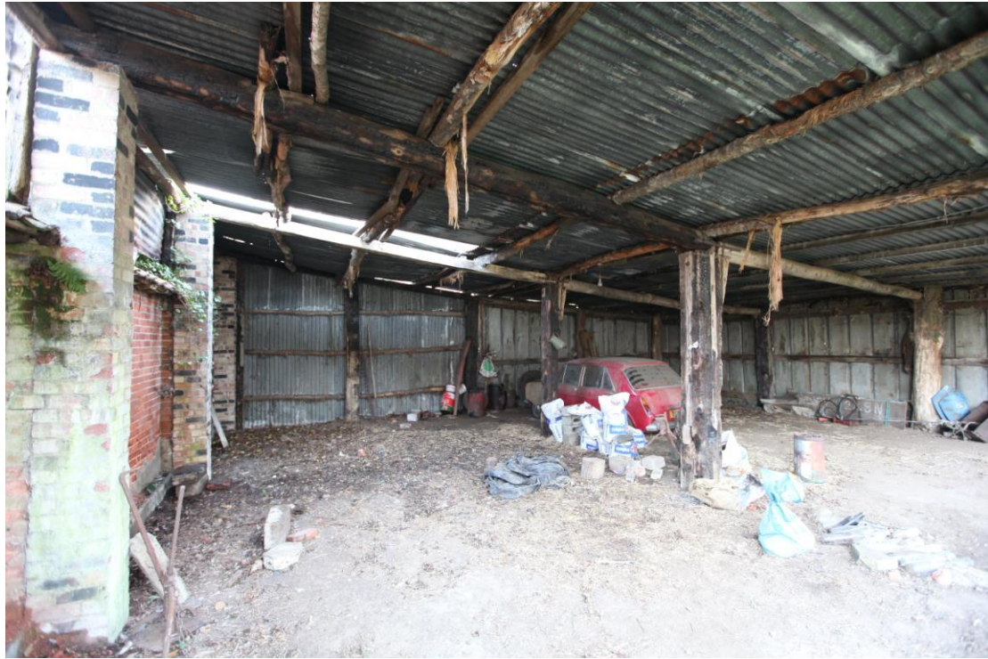
Illus. 5. The interior of the 20th century corrugated iron vehicle shelter (3) from the north showing the western exterior of the 19 th century brick shelter-shed (2) to the left.
