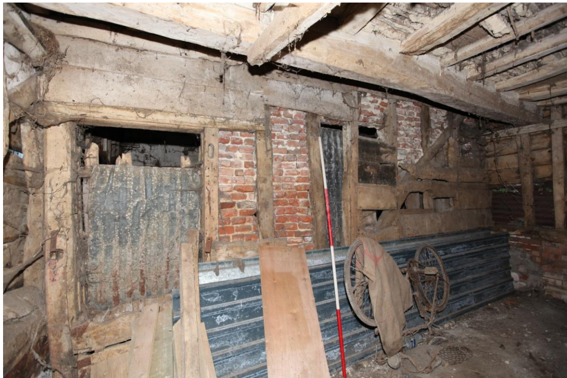
Illus. 10. The brick-nogged southern interior of the stable (1a) showing the door to the tack room (1b) to left and the position of the missing trough and rack beneath the hay drop to the right.
