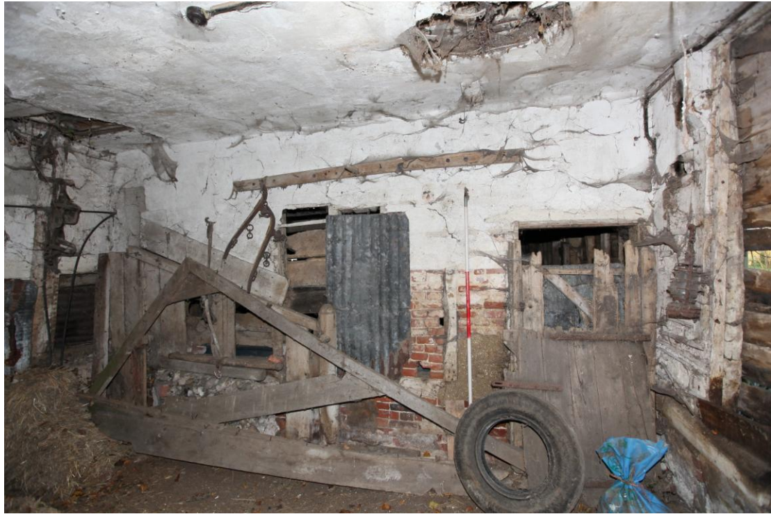
Illus. 13. The northern interior of the tack room (1b) showing the door to the stable (1a) to the right with the original 19 th century ceiling of tall-sectioned joists sandwiched between wattle-and-daub above and thick lime plaster beneath. Note the wooden rail of harness hooks (with harness still attached) and the slope of a stall partition with a carved oak finial to the left.
