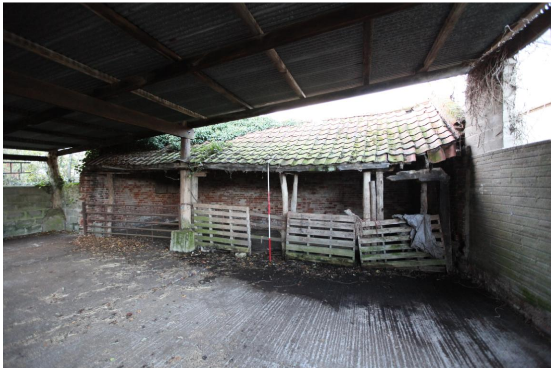
Illus. 6. The open-sided eastern exterior of the 19 th century brick shelter-shed (2) from the 20th century covered yard showing its pantiled roof and renewed arcade posts.
