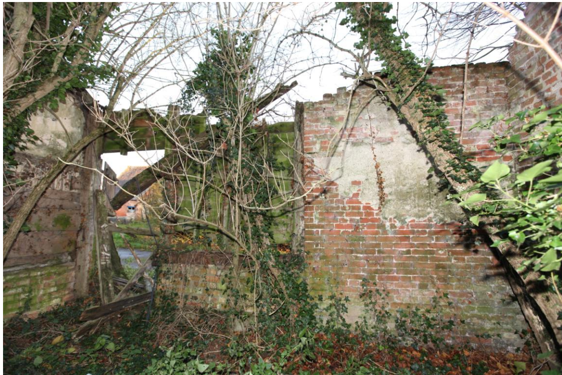
Illus. 14. The eastern interior of the partly collapsed loose-box (1c) showing what appears to be a 19th century brick extension to the earlier timber-framed stable range to the left.
