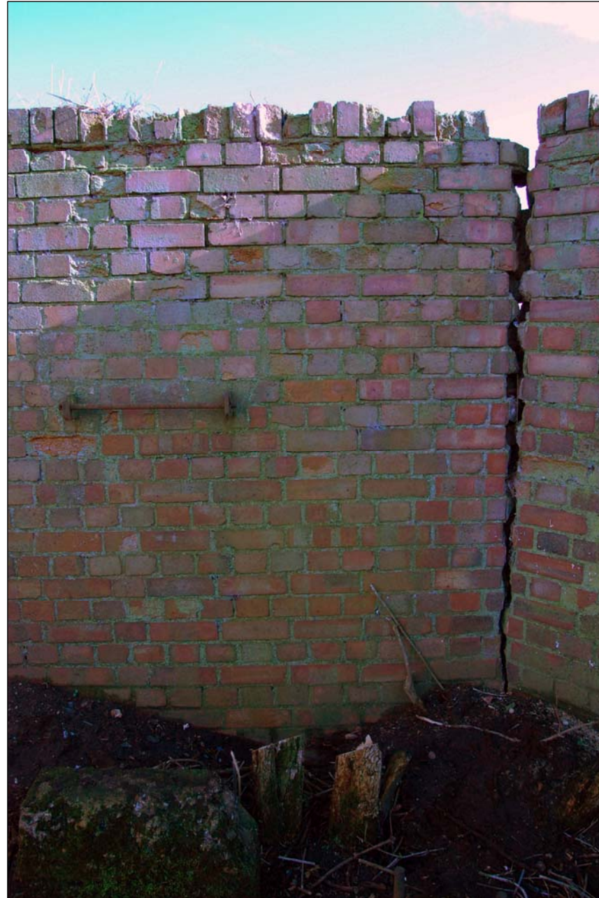
Plate 13. Left – HFDF curtain wall & foundations entrance, with concrete slab and octagonal internal foundation, facing east (photo colours edited to compensate for low light conditions)
