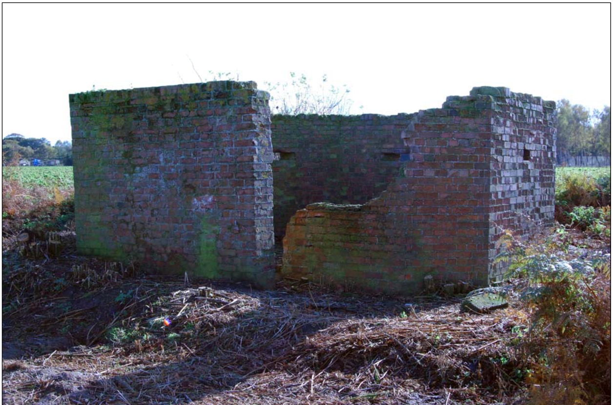
Plate 10. HFDF curtain wall, walls 5, 6a and b/entrance, facing south-east (photo edited to compensate for low light conditions)
