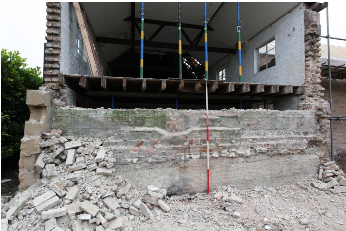
Illus. 2. The northern external gable showing a projecting course of masonry 1.25 m above the internal floor. This appears to relate to a raised floor in the previously demolished structure in the foreground.
