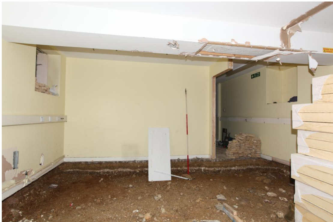
Illus. 10. The southern section of the maltings from the north showing the partition of the surviving 20th century office compartment (1c) and a horizontal layer of beaten clunch in the section of excavated floor beneath. This layer appears to represent the original floor and suggests headroom of no more than 1.75 m to the binding joists before they were raised in the 20 th century.
