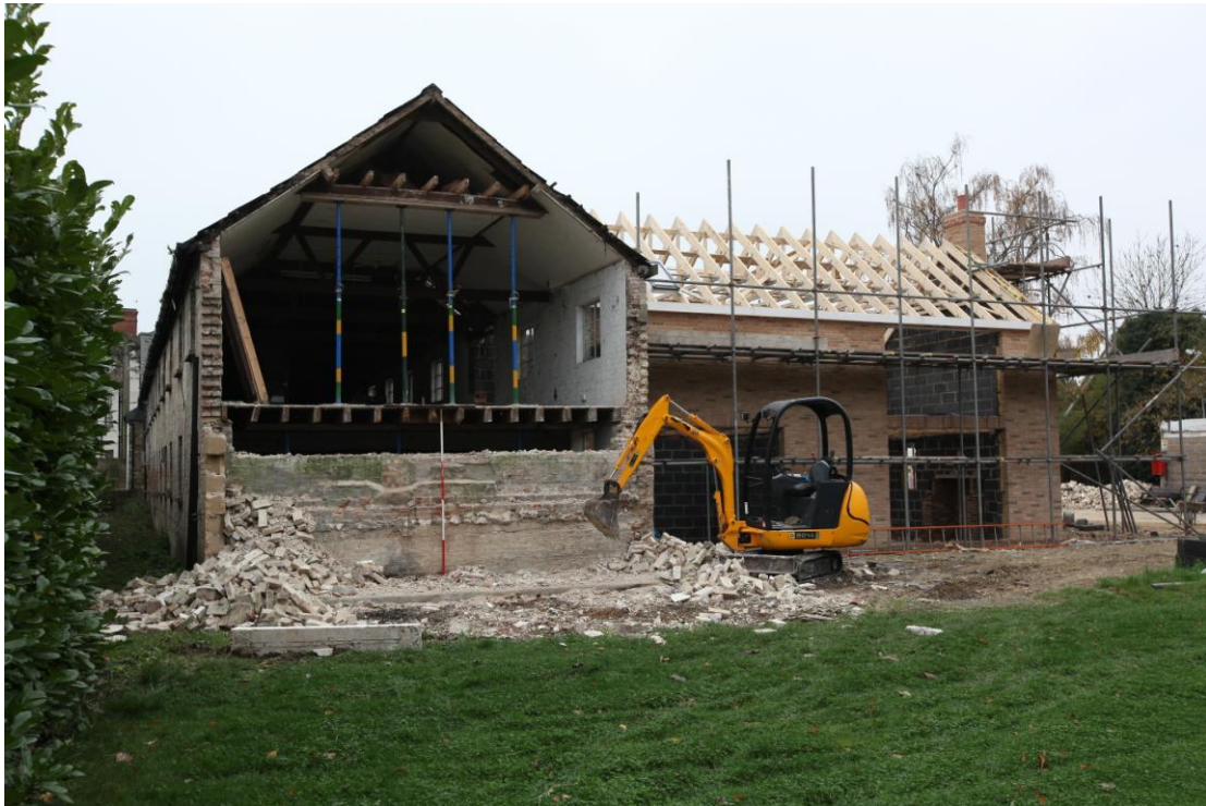
Illus. 1. The exterior of the partly demolished northern gable showing evidence of a raised floor in the previously demolished structure which occupied the foreground.
