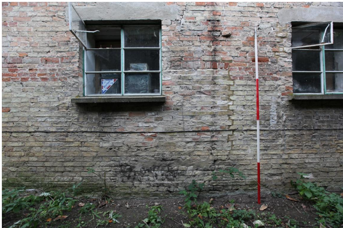
Illus. 4. The eastern exterior showing the lintel and closers (quarter-bricks) defining right-hand edge of a blocked low original window to the right (visible to the left of the scale). The courses of red brick at the same height as the lintel formed a decorative band dividing the original upper and lower storeys.
