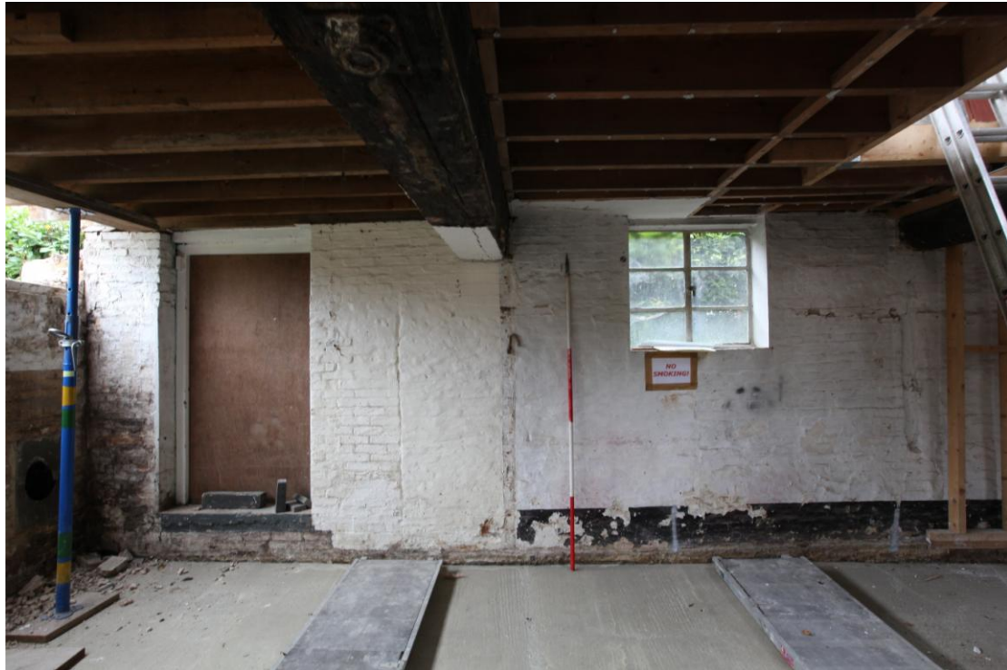
Illus. 7. The northern end of the eastern interior showing the partly demolished northern gable to the left. The scar of a blocked original door is visible to the right of the existing door (with later infill between the two) and patches of secondary brickwork beneath both original binding joists show the extent to which they have been raised. A vertical groove beneath the right-hand joist terminates at the original ceiling height.
