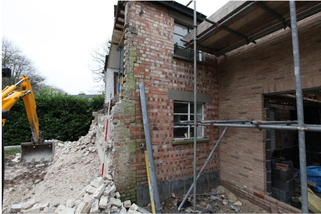
Illus. 3. The north-western corner of the building showing the recent extension to the right. The 20 th century Fletton brickwork in the centre has been intruded into the corner of a previously demolished structure which extended further to the north (left) and contained a raised floor as indicated by the projecting course of clunch in its partly demolished gable.
