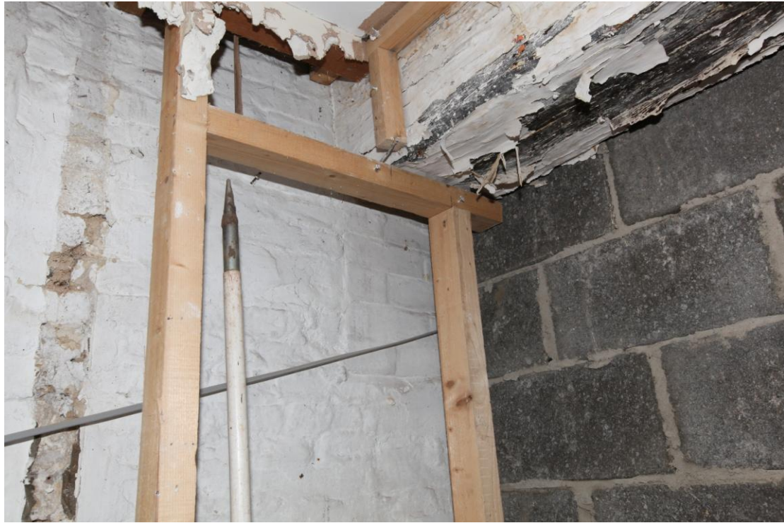
Illus. 9. A detail of the later brick infill beneath the raised binding joist in the western interior of the southern section. The vertical scar to the left relates to a secondary partition which pre-dates the most recent dry-lining.
