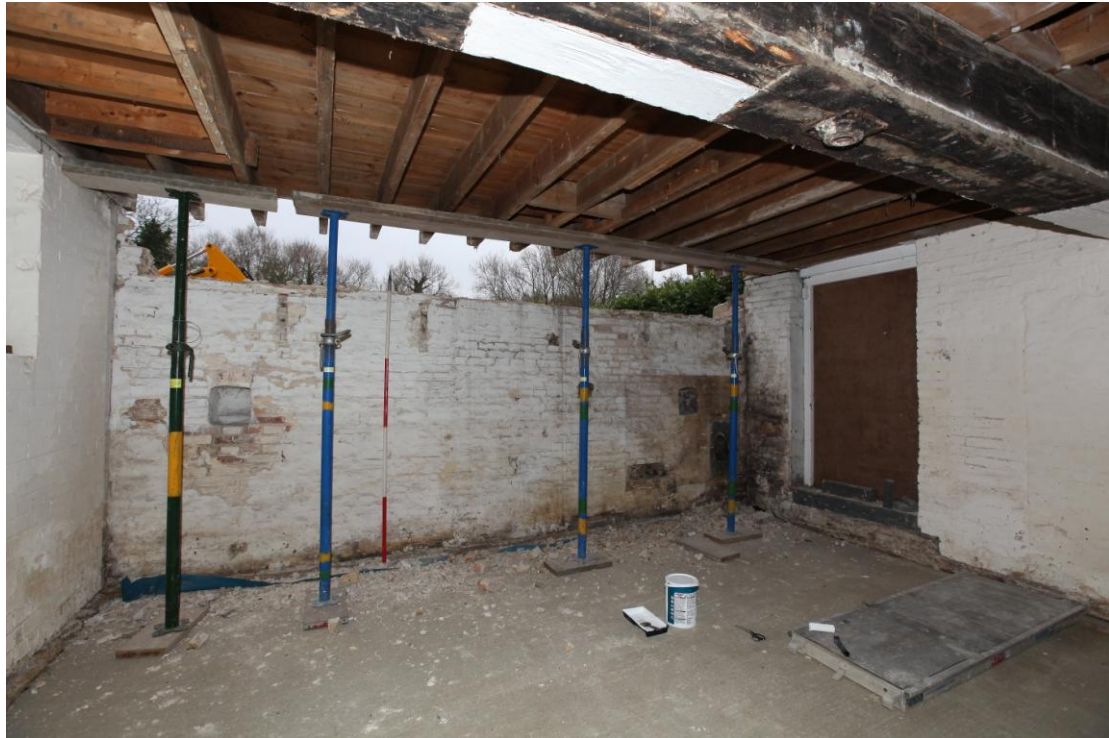
Illus. 5. The interior of the northern gable showing original square niches to left and right together with the 20 th century softwood common joists of the ceiling.
