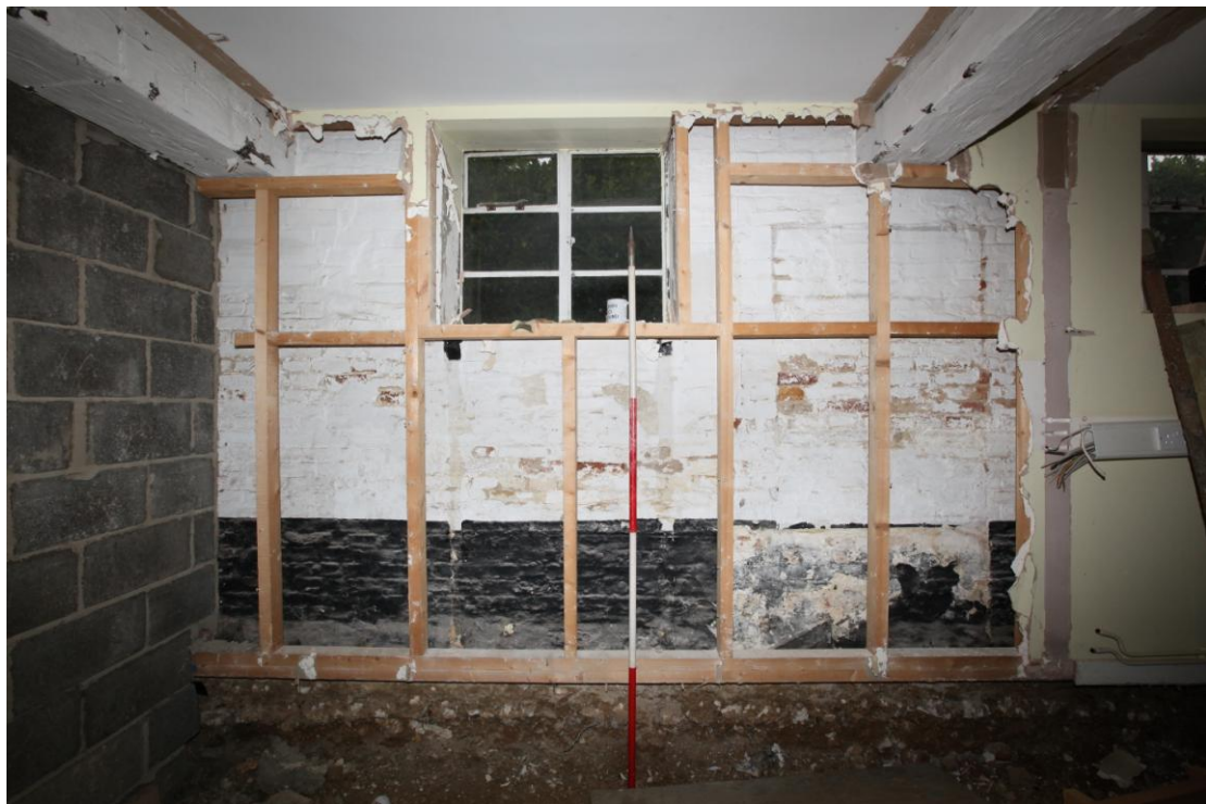
Illus. 8. The eastern interior of the southernmost of the three sections into which the maltings has been divided by block-work partitions, showing the whitewash and painted black skirt beneath the 20th century cladding which still survives to the right (with the vertical scar of the former office partition, 1d).
