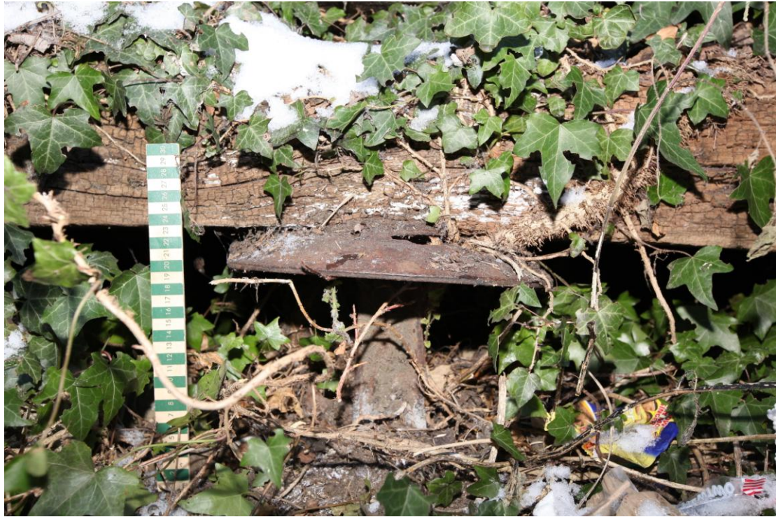
Illus. 11. A detail of the cast-iron mushroom with cross-sectioned base supporting the eastern ground sill immediately beneath the entrance to the detached granary (4).
