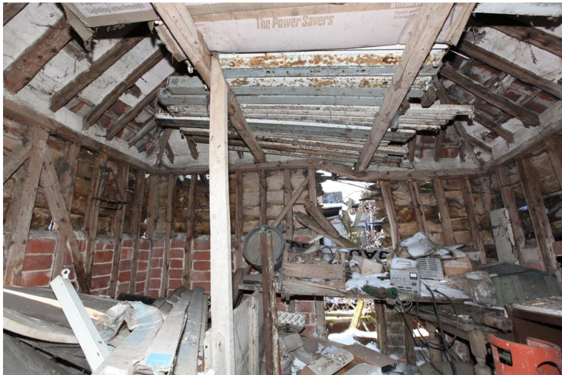
Illus. 12. The interior of the detached granary (3) from its central eastern entrance showing the narrow ostensibly secondary door in its western wall and the plaster beneath the pantiles. The brick infill probably indicates the height of the missing grain bins.
