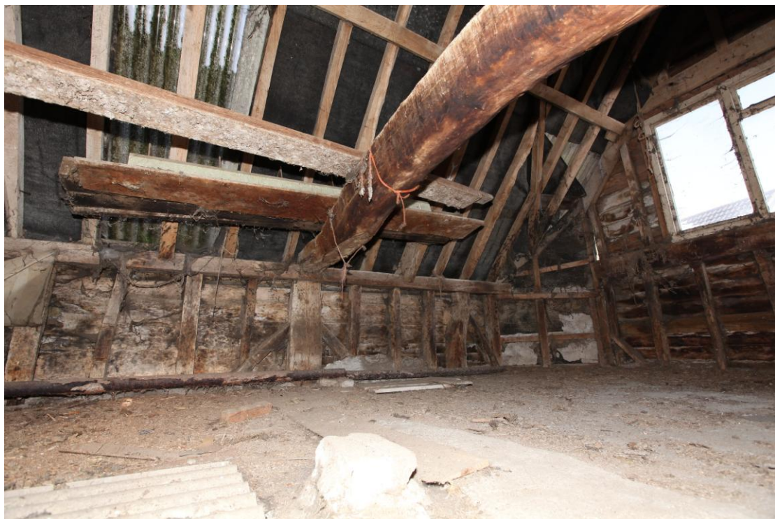
Illus. 8. The northern interior of the loft above the milking parlour (2) showing its timber-framed walls with nailed primary braces and an original tie-beam. The rafters of the butt-purlin roof structure are also interrupted by diagonal braces as in the roof of the barn (1) and both buildings appear to be contemporary.
