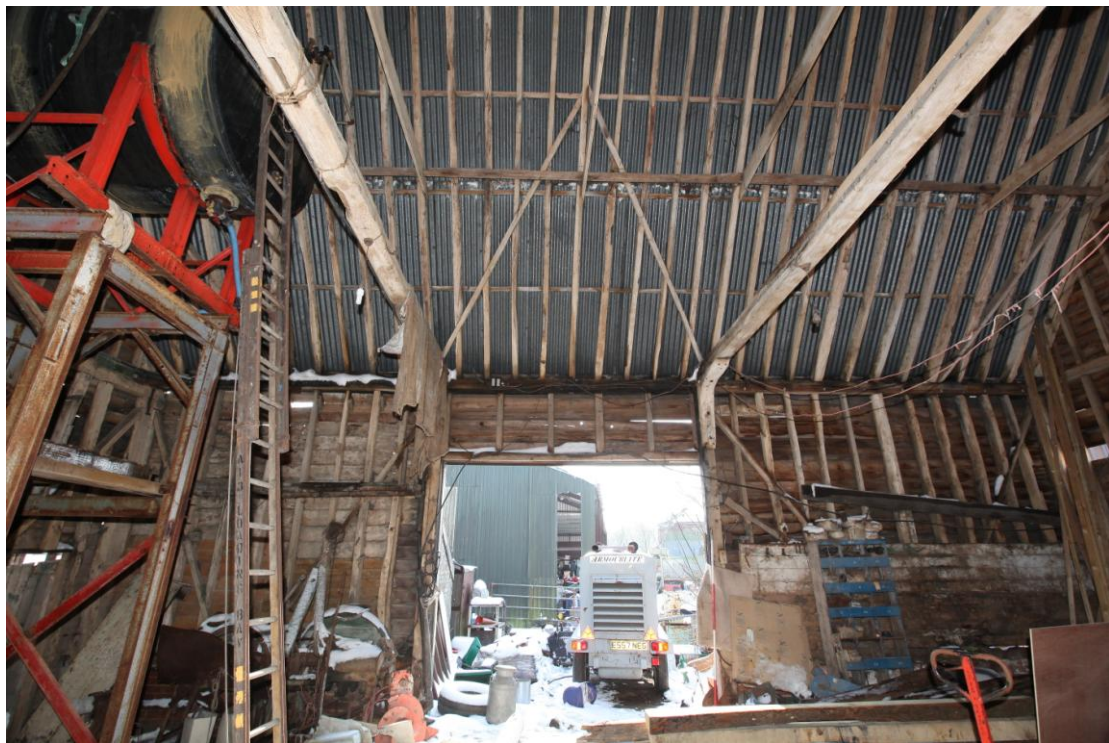
Illus. 4. The southern interior of the barn (1) showing the original entrance in its central bay (now reduced in height and lacking doors). The bolted knee-braces to the tie-beams are original features, and the diagonal primary wall and rafter braces are typical of the mid-19 th century.
