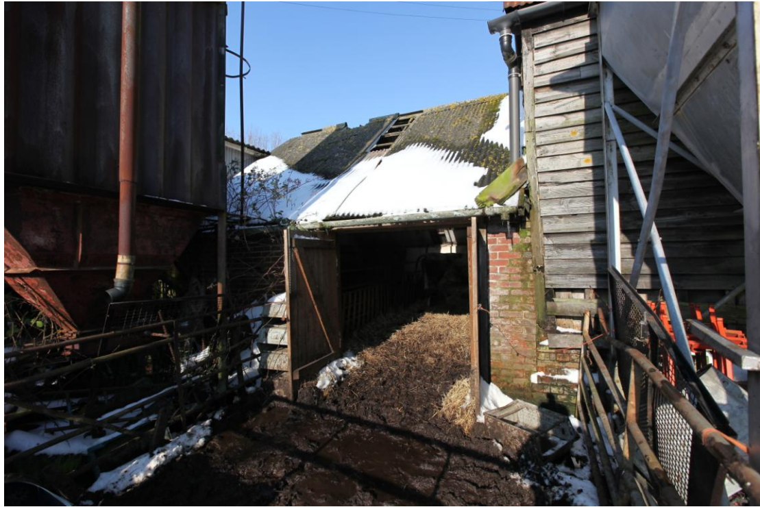
Illus. 9. The southern exterior of the brick loose box (3) showing the modern cattle pen in the foreground and the corner of the barn (1) to the right.
