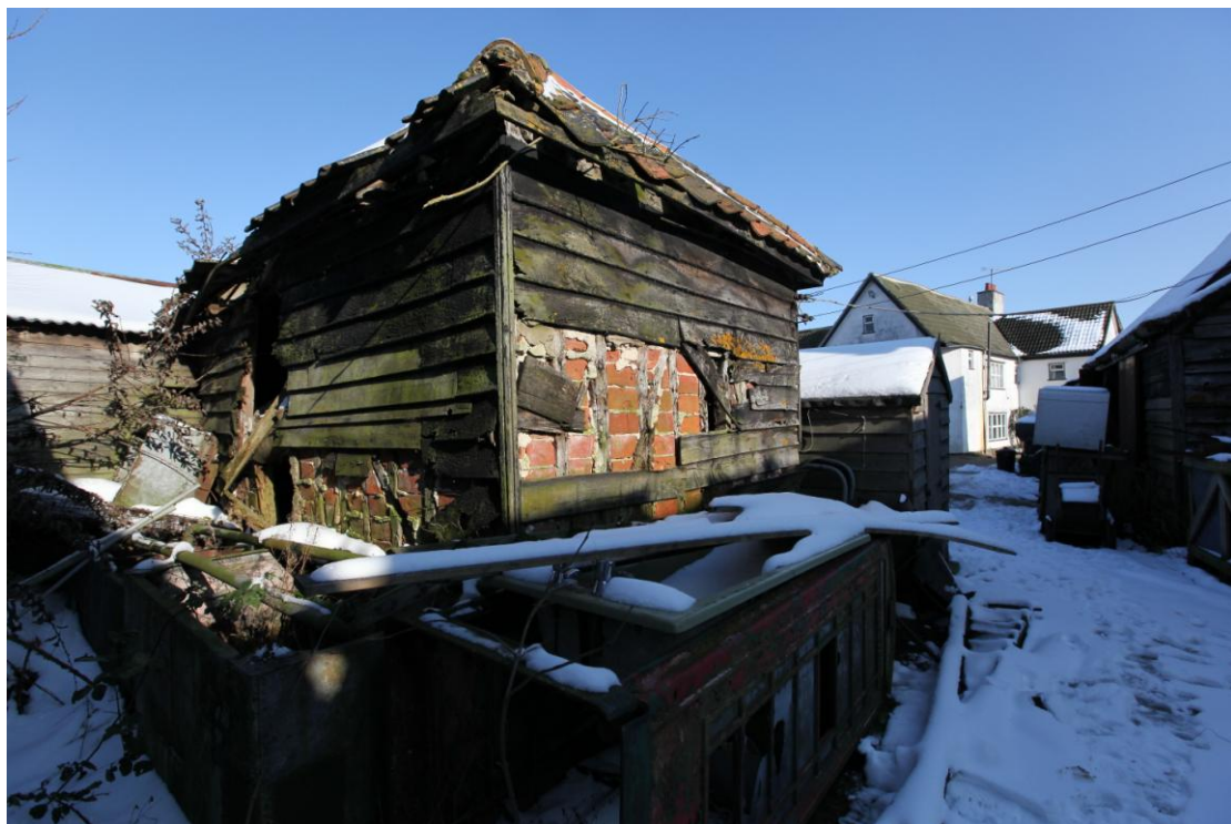
Illus. 10. The detached granary (4) from the south-west showing its hipped pantiled roof and the remains of heavily tarred original weatherboarding. The farmhouse (7) and barn (1) are visible to the right.
