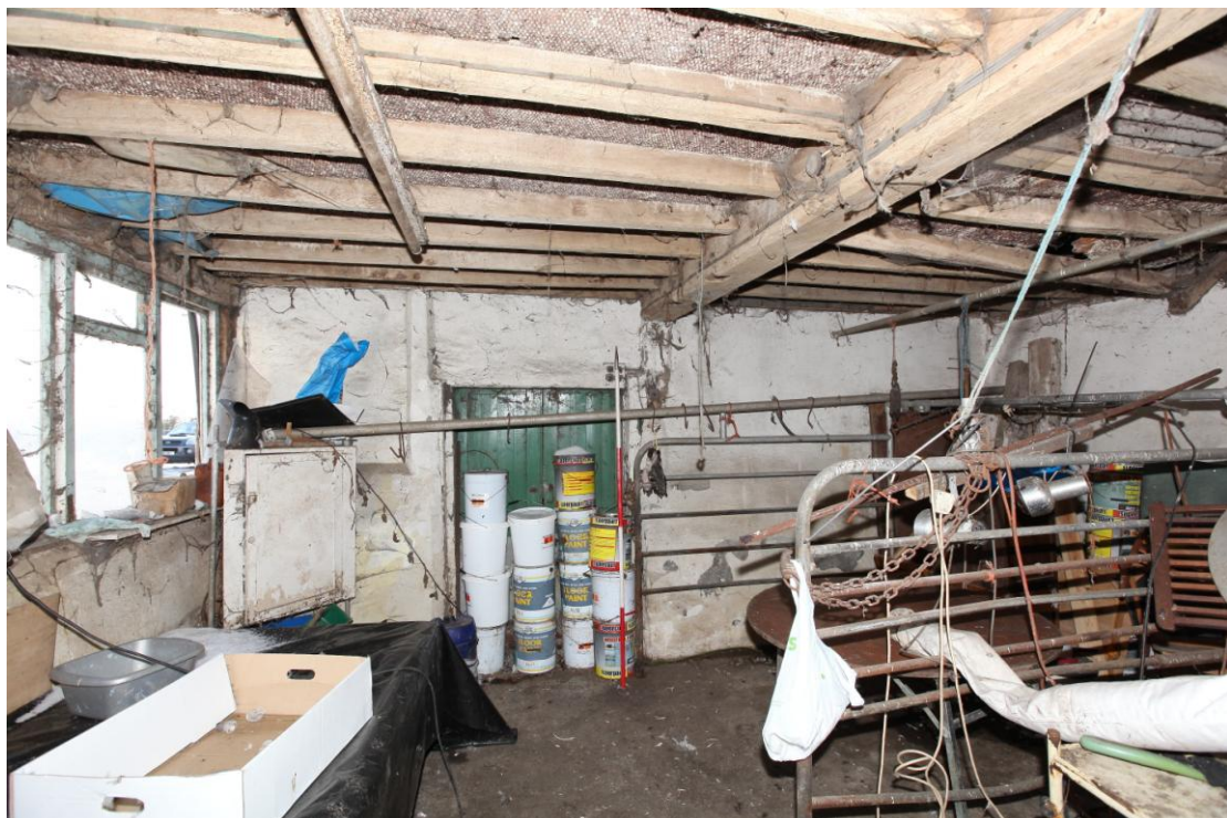
Illus. 6. The rendered and whitewashed southern internal wall of the milking parlour (2) showing its two external doors with the 20th century windows of the eastern gable to the left. Although used most recently as a milking parlour this shed may have been designed as a stable.
