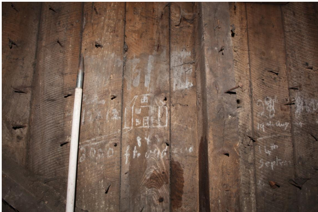
Illus. 12. Detail from west of chalk graffiti to partition between forge (B) and carpenter's shop (A) showing drawing of house and iron nails for hanging tools.
