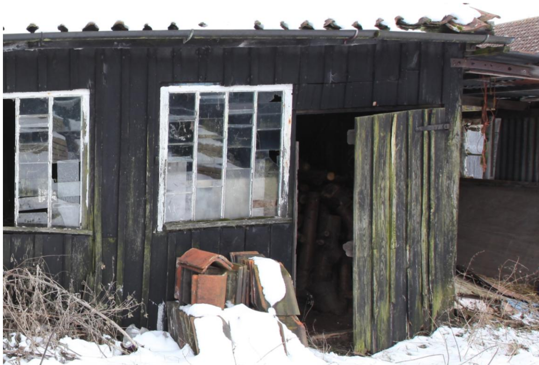
Illus. 4. Western end of northern exterior showing entrance door and windows with overlapping 'waster' panes of forge (B).
