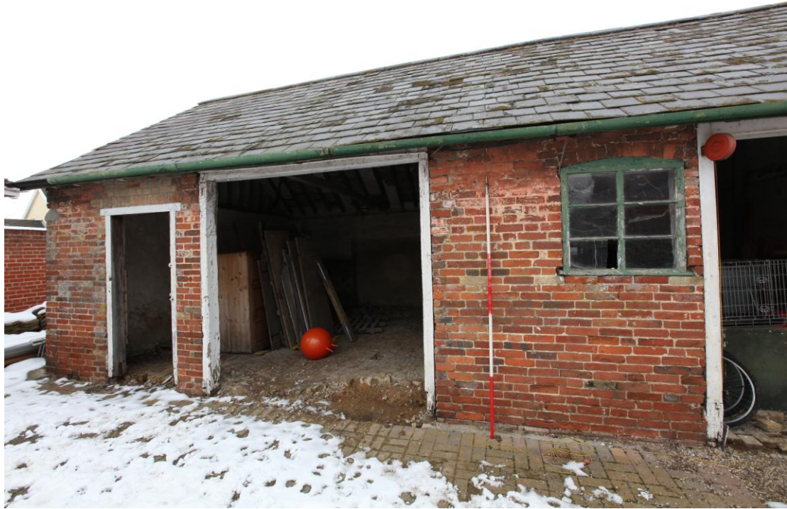
Illus. 5. Southern vehicle door (A) showing edge of original narrow door respected by brickwork to left & cut bricks to right. The smaller left-hand door is surrounded by cement pointing and is entirely secondary. This shed was originally entered by a narrow central door.
