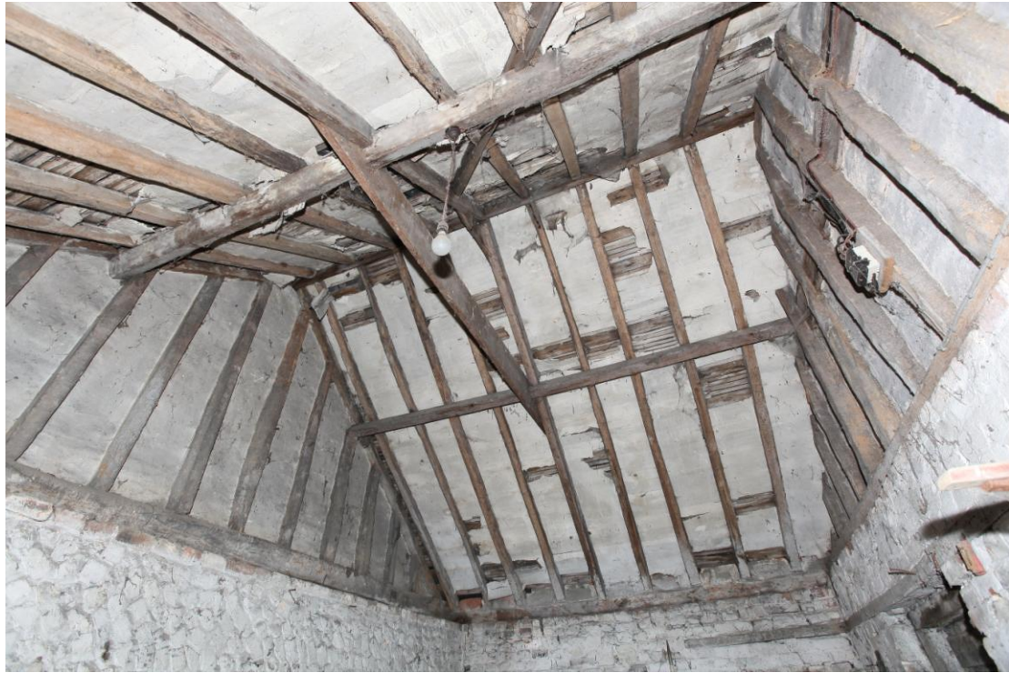
Illus. 11. The clased-purlin roof structure of the northern shed (C) with original lath-and-plaster, seen from the south-east showing the northern gable to the right.
