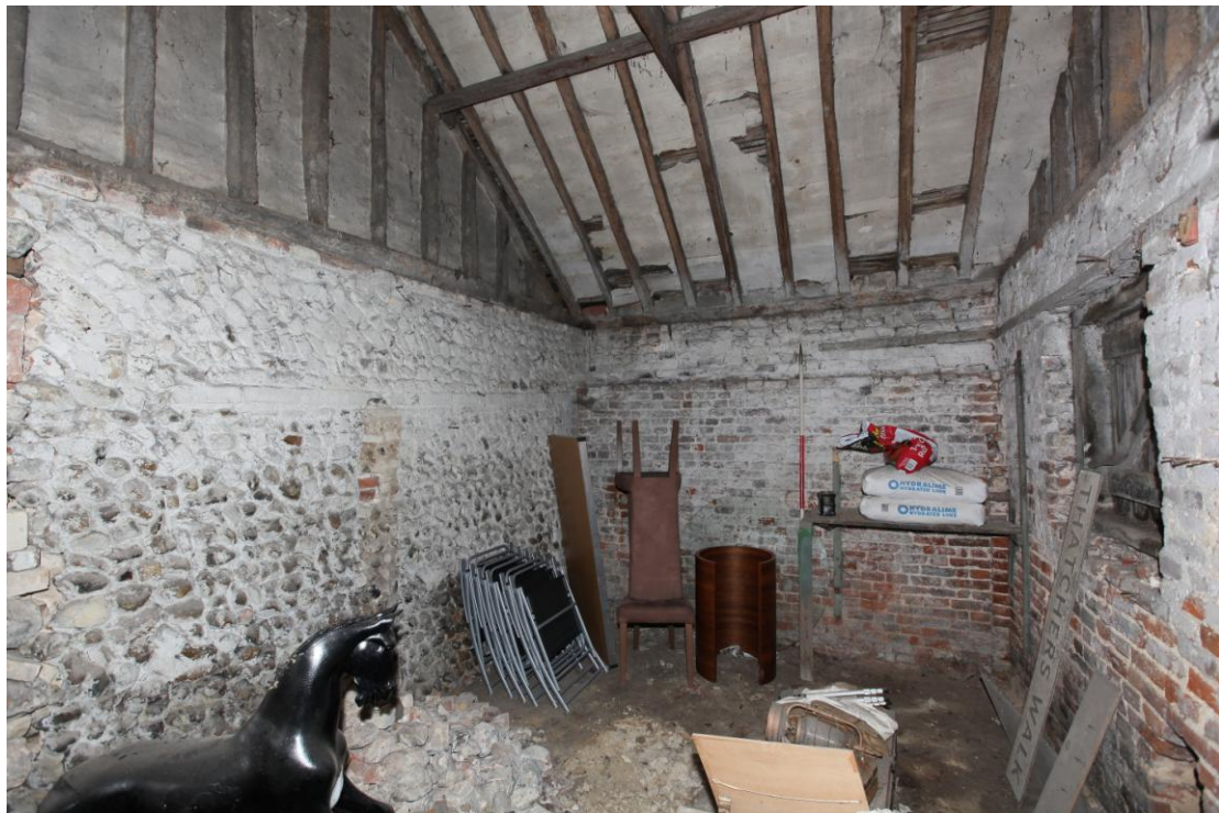
Illus. 10. Interior of northern shed (C) from south-west showing flint-rubble partition to central shed (B) to left. The shelf in the brickwork of the rear wall marks the 19 th century 'lift' and is respected by a line of brick in the left-hand partition – suggesting its lower fabric may also pre-date the building of 1853.
