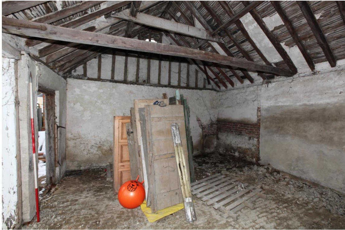
Illus. 7. Internal south-western gable of southern shed (A) showing the dated tie-beam in the foreground and the scar of a secondary partition (since removed) immediately behind.
