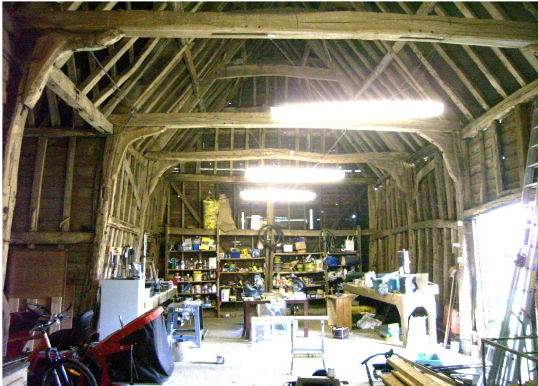
Illus. 5. General view of barn interior from east showing central porch (2) to left and bolted knee-braces replacing the original arch-braces to the tie-beams.
