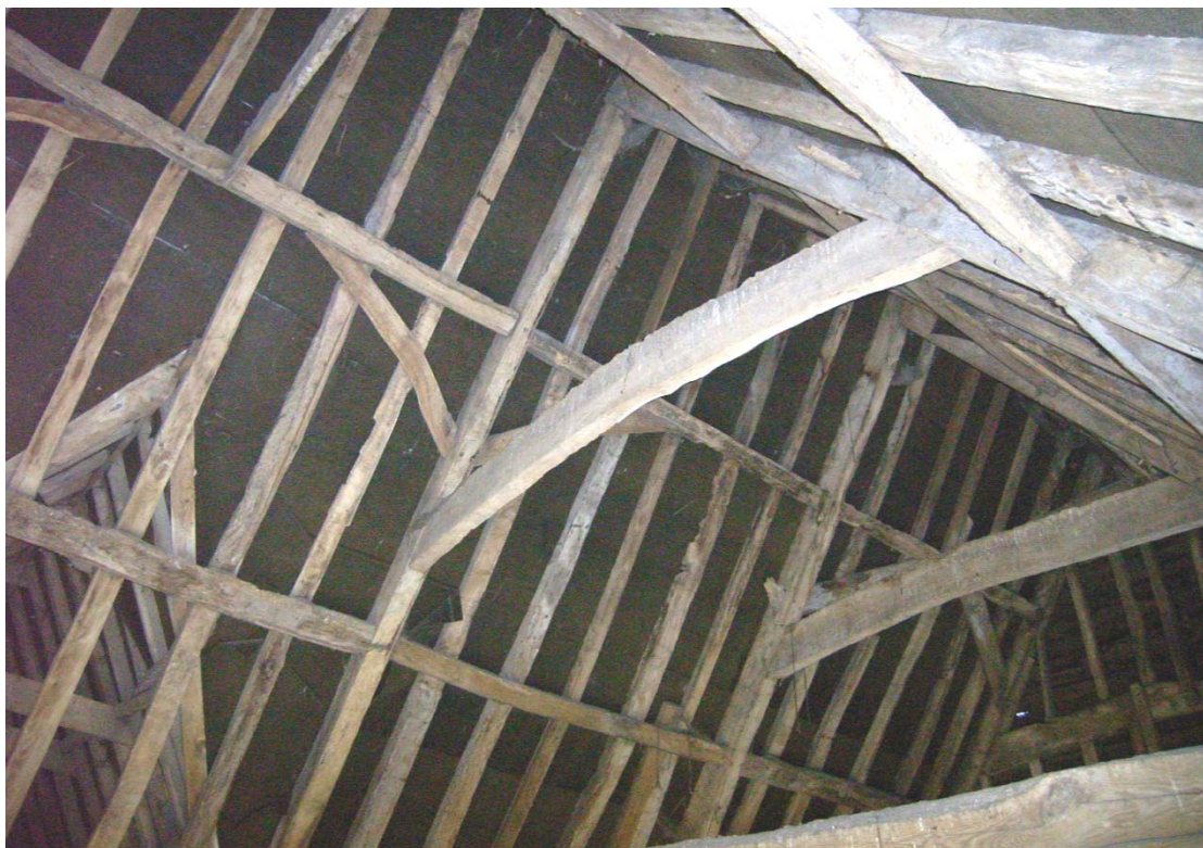
Illus. 6. Detail of roof structure of barn from north showing the two tiers of butt-purlins with intact wind-braces to the upper tier. The clasped-purlin roof of the porch (2) is shown to the left
