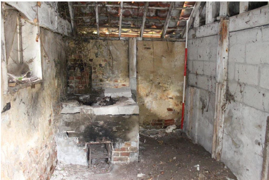
Illus. 6. Interior of southern shed (1b) from east showing copper to left and vertical groove of grain bin in post to right. The internal partition to the right is a 20 th century block-work insertion, and the apotropaic 'M' symbols are incised into the plaster of the southern gable to the left.
