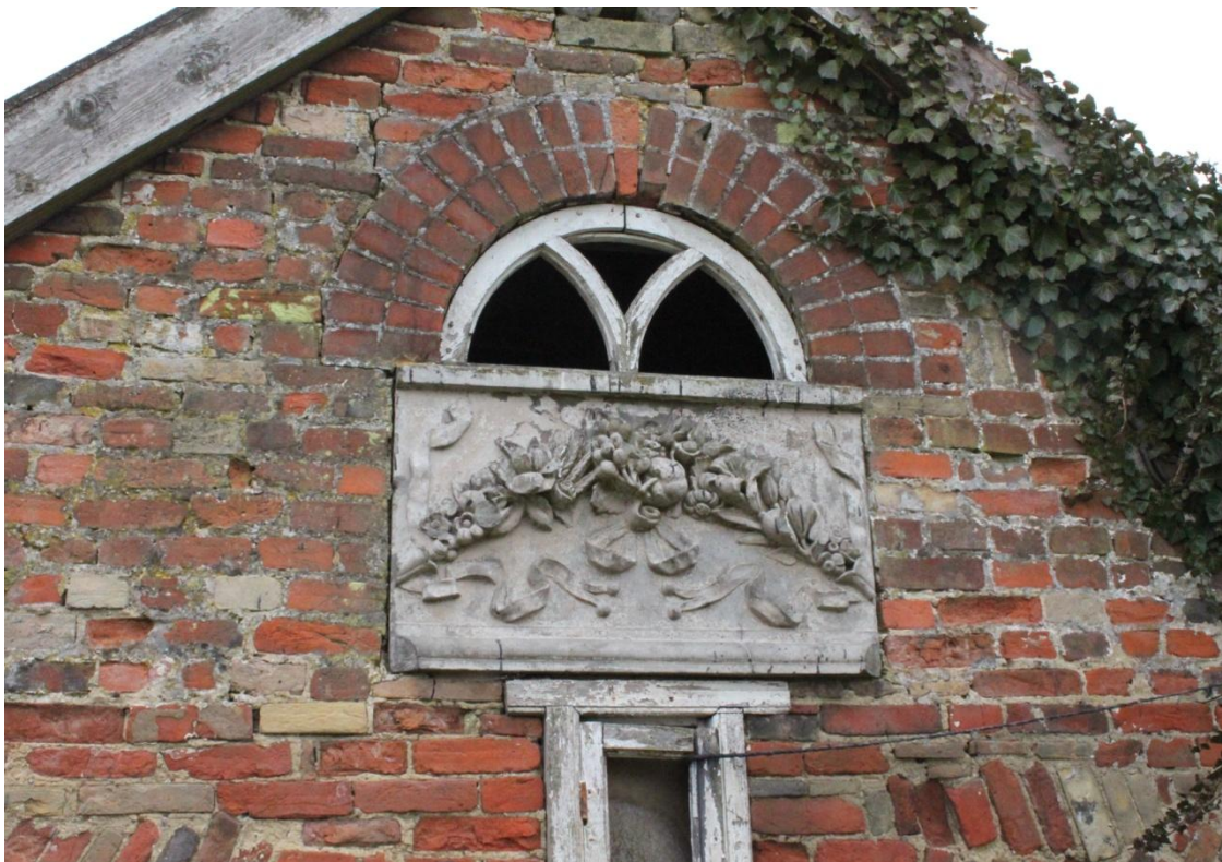
Illus. 4. Detail of re-used stone panel in northern external gable with narrow secondary window below.
