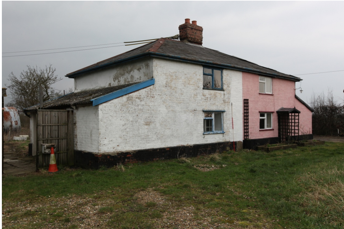
Illus. 3. The exterior from the north-west showing the one remaining area of exposed original fabric of rendered clay above the lean-to of the northern gable. The same area of the southern gable is weatherboarded. The upper part of the chimney consists of 20 th century Fletton brick and was probably rebuilt in the 1960s.
