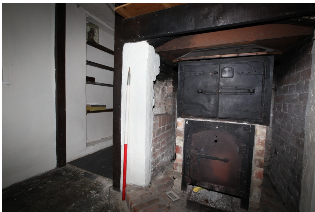
Illus. 12. A detail of the 19th century fireplace in the southern Living Room (1) showing the aperture of a probable bread oven door in its left-hand pier.
