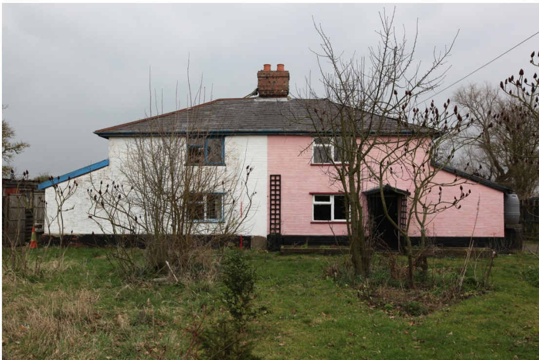
Illus. 2. The symmetrical western facade with contemporary lean-tos adjoining both gables. The present brick facade and slate roof date from a late-19 th century refurbishment and the original building was probably thatched. The original left-hand entrance was blocked when the two cottages were combined and the present windows inserted during the 1960s.
