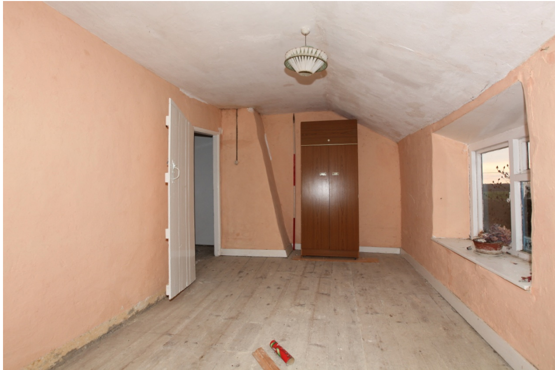
Illus. 7. The Front Bedroom (2B) of the northern cottage from the north, showing the slope of the central chimney and the 0.5 m thickness of the western facade to the right. A 19 th century plank-and-batten door opens onto the rear bedroom (2A) to the left.
