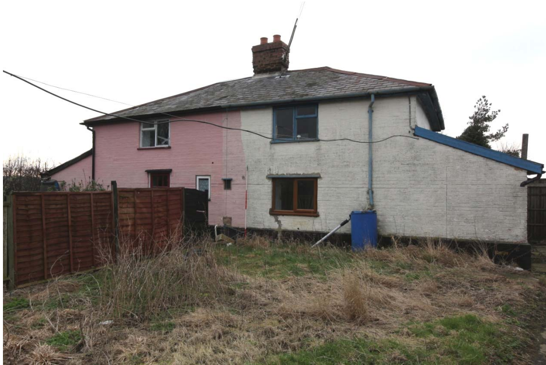
Illus. 5. The rear (eastern) exterior with evidence in the brickwork of two earlier, narrow ground-floor windows but no doors. The position of the southernmost window to the left is now occupied by a secondary door.
