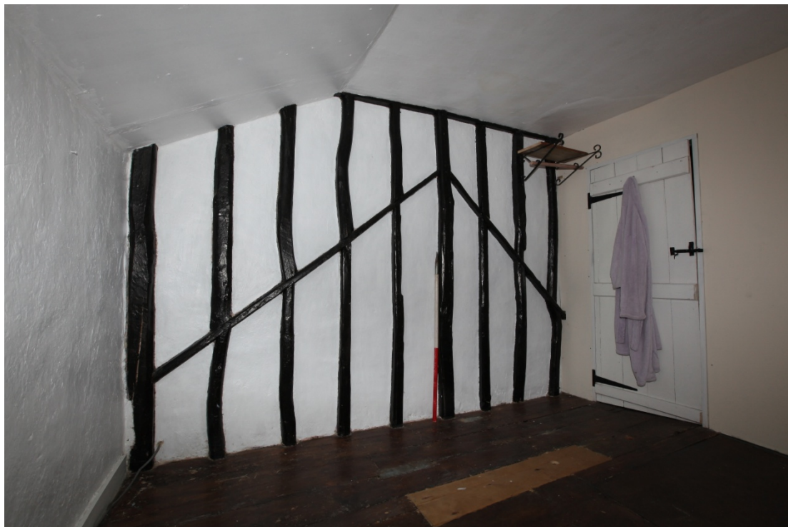
Illus. 11. The rear Bedroom (1A) of the southern cottage seen from the east, showing the hipped southern gable to left and the 19th century studwork partition to the front Bedroom (1B). The plank and batten door to the right opens onto the stair Landing (1).
