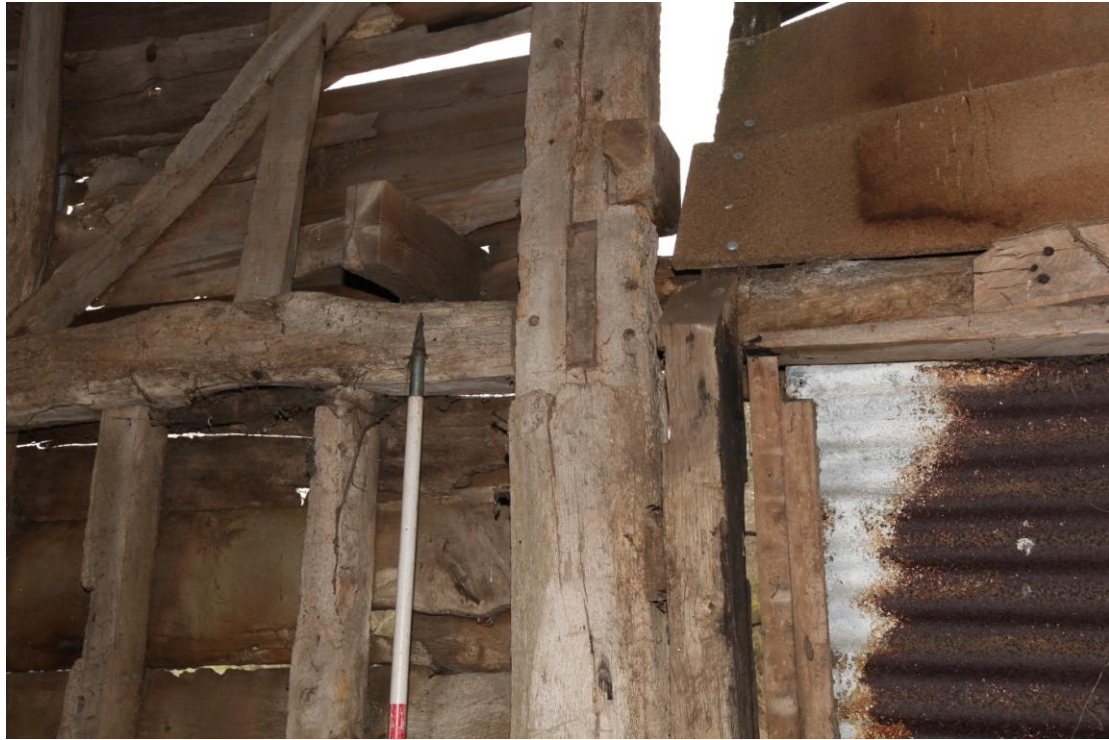
Illus. 7. A detail from the west of the mortise and integral corbel in the central storey post of the two stable bays (E and D) for the binding joist of a missing hay loft. The blocked door in bay D to the right is a secondary insertion and the original stable entrance presumably lay in the rebuilt northern gable or western wall.
