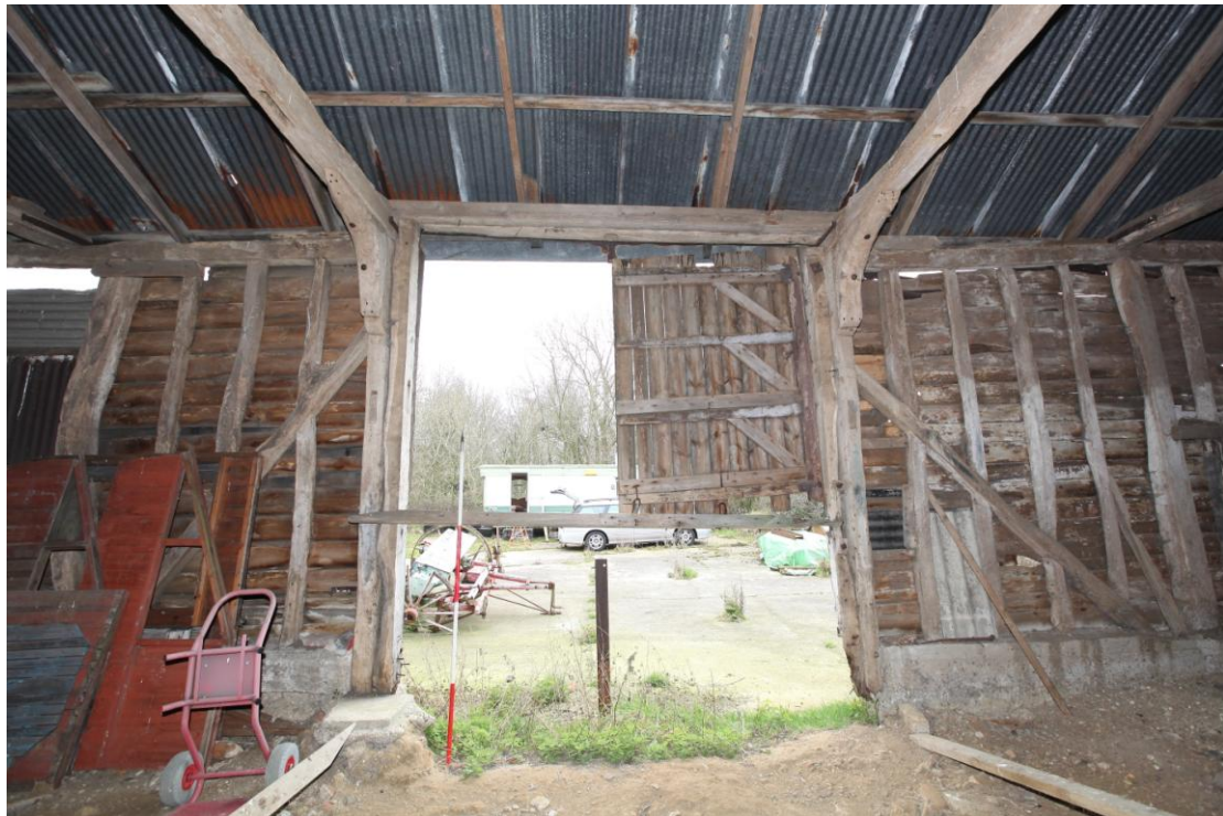
Illus. 9. The eastern interior of the original entrance bay B showing its raised secondary roof-plate and the bolted knee-braces which replaced the original arch-braces to the tie-beams.
