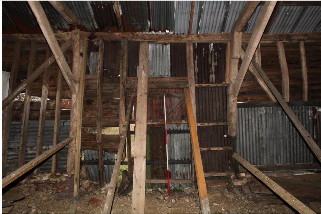
Illus. 11. The western interior of the entrance bay B showing the 20th century narrow door in the centre. The jowled storey posts on each side contain mortises for the lintel of the original low rear door of the threshing floor as seen in illus. 12 below. The roof-plate contains a series of empty mortises for the missing studwork above this lintel, proving the barn always faced east towards the farmhouse.
