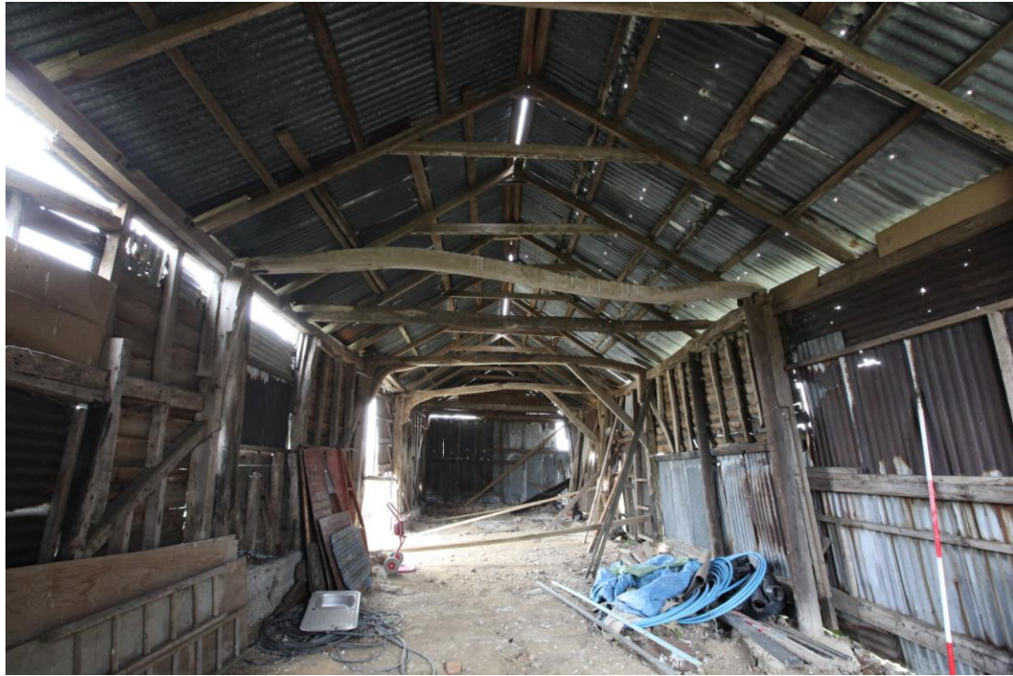
Illus. 5. A general view of the interior from the north showing the late-18 th or early-19 th century timber frame with substantial areas of 20th reconstruction and a replaced through-purlin roof of softwood with nailed collars and some re-used timber.
