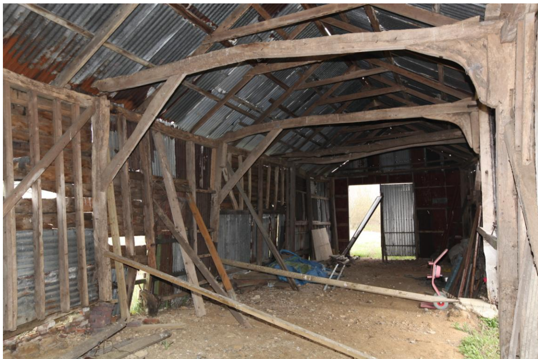
Illus. 10. The two original arch-braces to the tie-beams flanking the western interior of the entrance bay B, as seen from the south-east. The matching braces to the right were replaced by bolted knees in the 19 th century. Note the 20 th century vehicle doors in the northern gable and the loose earth floor throughout the barn.
