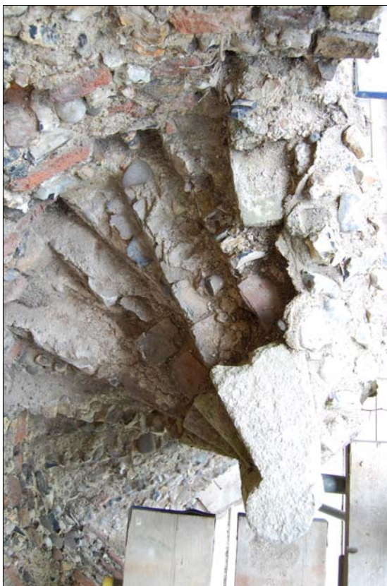
Plate 11. Spiral stairs in the SW corner tower (T5). The stone centre post with the stub of winders are reused from a previous building.
