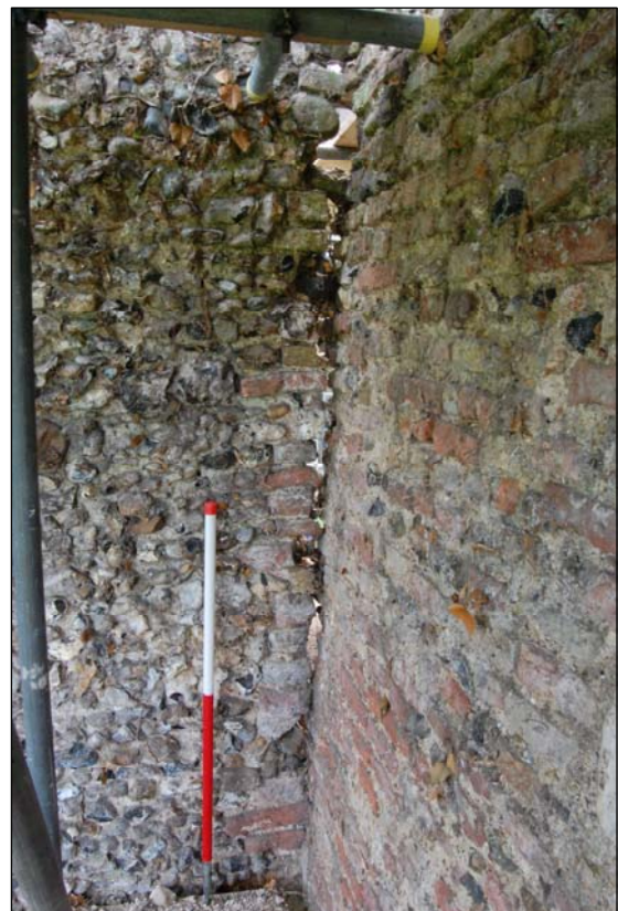
Plate 21. Butted joint between the first phase flint work of the north curtain wall and the later brick-built NW corner gate tower. 1 x 1m scale
