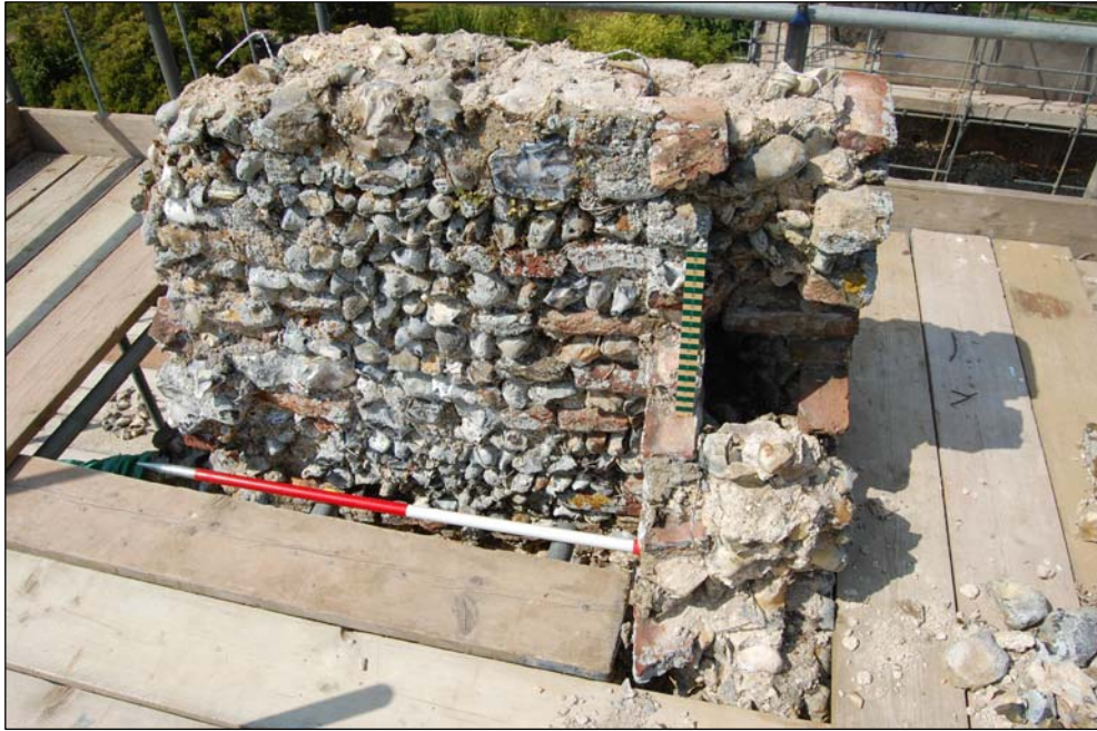
Plate 13. Remains of the stair turret above the roof-line of the SW corner tower (T5) with socketed timber setting built into the thickness of the wall (to the right of the 30mm scale). The shape suggests that it supported a vertical post but there is also a putlog for a horizontal timber to exit through the east (right) face. 1 x 1m scale, 1 x 0.3m scale
