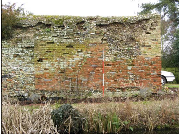
Plate 24. South curtain wall brick infill on the south face and truncated east end. 1 x 2m scale
