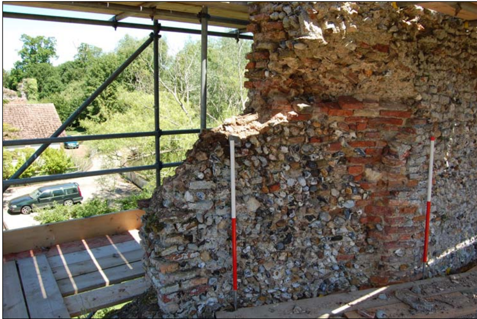
Plate 19. The raised section of parapet (62) at the east end of the north curtain wall shielding the entrance (D11) to the second floor of the NW corner tower. The top of the only surviving merlin of the crenulations that once topped the parapet can just be seen between the scaffold floor boards to the left of the picture. 2 x 1m scale
