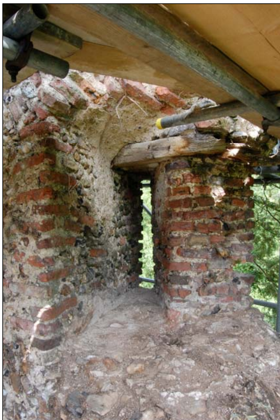
Plate 20. Angled double slit window in the east wall of the NE tower (first floor), the window reveal angled to view the NE approaches to the keep.
