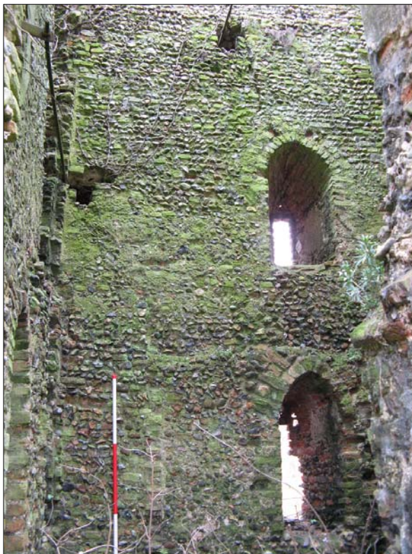
Plate 8. Interior of mid tower (T4) showing stepped ledge at first floor level. The scale is within the remains of enclosed shaft in the SE corner. 1 x 1.5m scale
