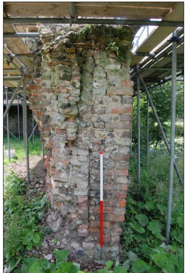
Plate 15. Brick quoin at the north end of the west curtain wall, the jamb of a now missing door (D1), with raised brick stop to the left of the scale. 1 x 1m scale
