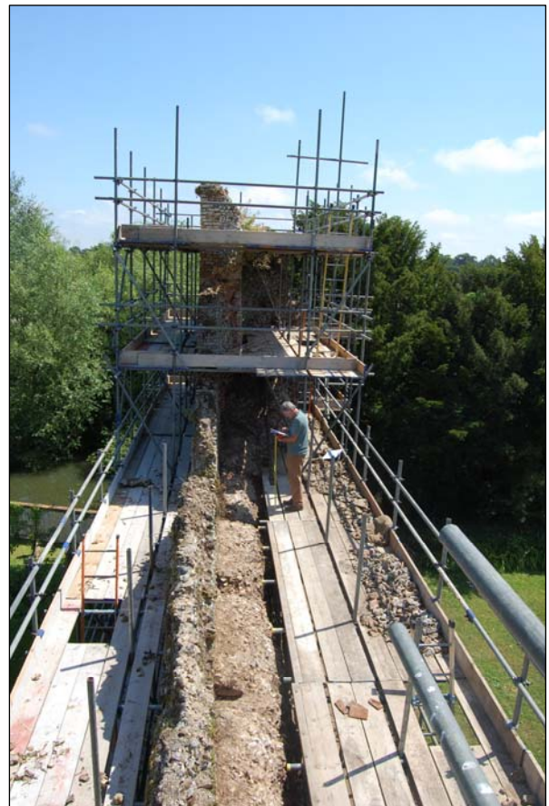
Plate 18. North curtain wall-walk seen from the gate tower (T1). The parapet wall has been truncated and the crenulations lost from its top.
