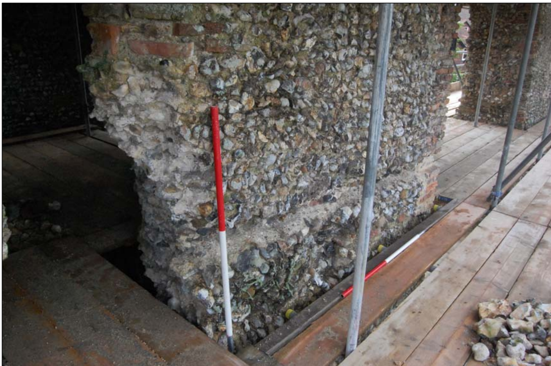
Plate 23. Horizontal scar across the north face of the mid-tower (T4) where the roof of the timber-framed hall was attached to the tower at its eaves. The section of the wall between the first floor door and second floor window, to the left of the scale has been removed prior to repairs. 2 x 1m scale
