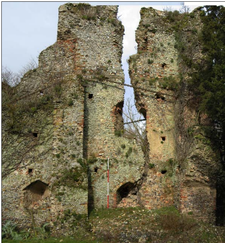
Plate 5. NE corner tower (Tower 2) interior viewed from the south showing east side of the tower detached from the west and anchored by a large chain, with rubble banked up at the base.
