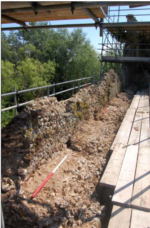
Plate 17. The wall-walk across the top of the north curtain wall. Slots to retain the joist of a boarded deck were regularly spaced along its length and can be seen between the scales. 2 x 1m scale
