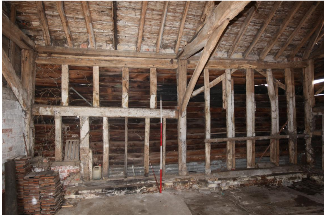
Illus. 7. The rear (western) interior of the two northern bays (B & C), showing the largely original timber framing with externally trenched wall braces. The horizontal mid-rail of the central bay (B) to the left is secondary, but the storey posts contain mortises for a lower predecessor that would have formed the lintel of a small rear door. The low height of these mortises (1.2 m or 4 ft above the present concrete floor) indicates the ground level has risen by as much as 0.6 m – or the walls have been reduced to the same extent.
