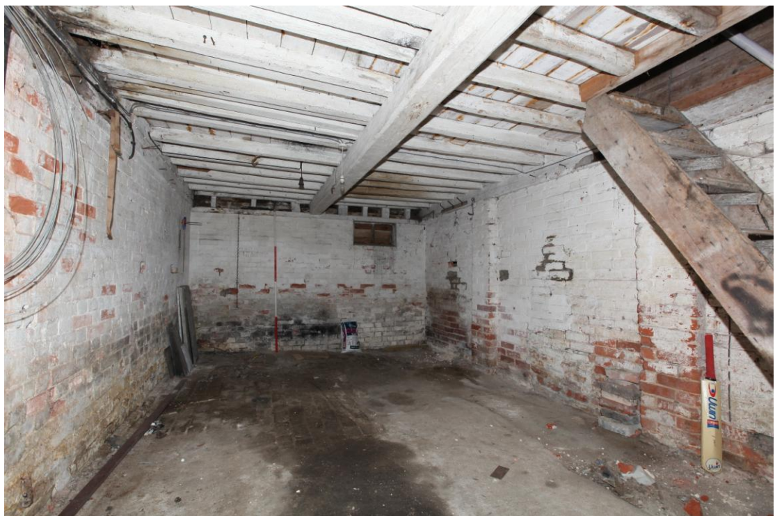
Illus. 12. The interior from the east of the southern bay (A) showing its 19 th century brick walls and ceiling with a 20 th century loft stair to the right. The feet of the original studs are visible above the brickwork in the rear (western) wall. This area was initially open to the rest of the barn but has a 19 th century brick floor and was probably converted into a vehicle or storage shed with a granary above.
