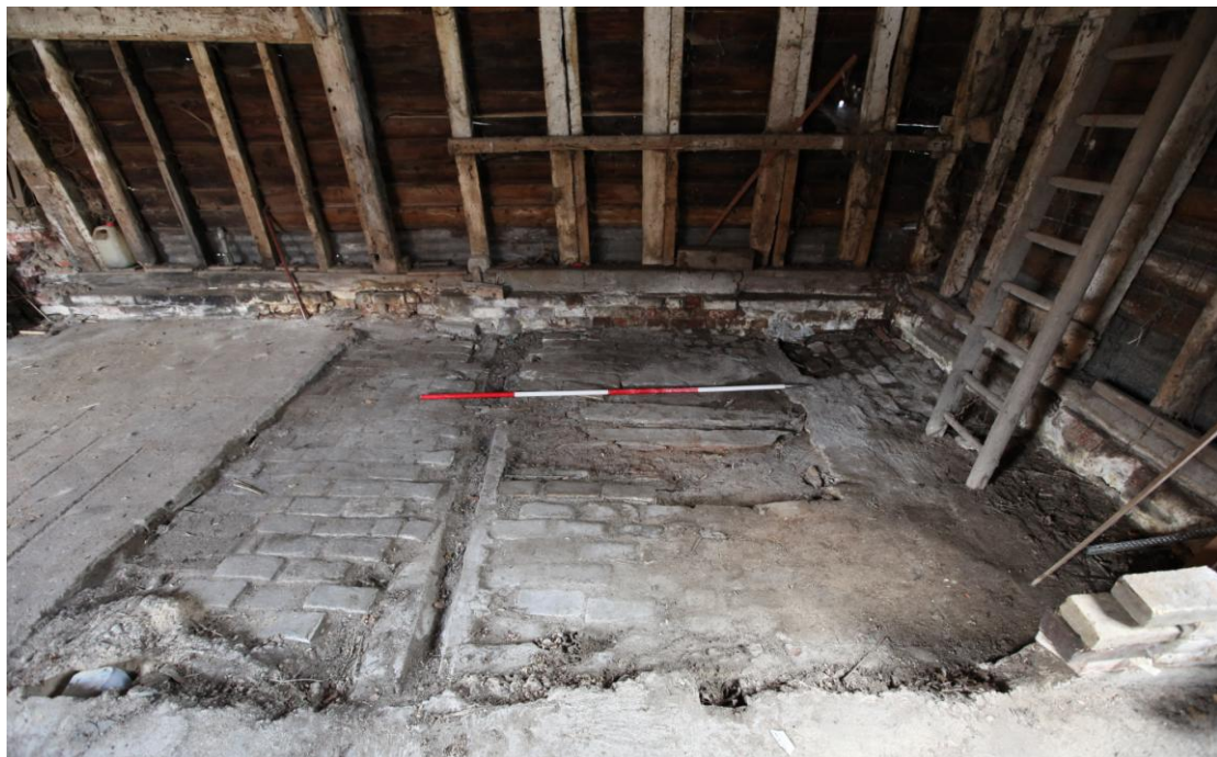
Illus. 8. A section of 19th century brick flooring with a lateral drain exposed beneath the 20 th century concrete floor in the north-western corner of the barn (i.e. in bay C, viewed from the east). This end of the barn have been used as a stable at some point.
