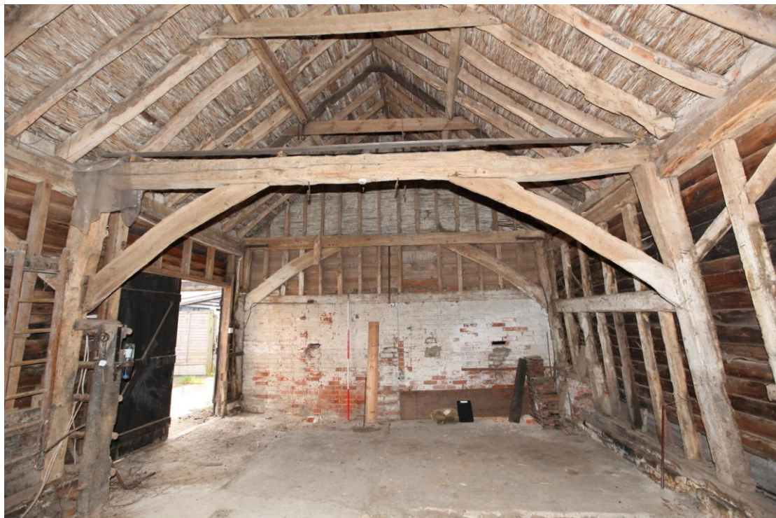
Illus. 6. The two intact arch-braced open trusses seen from the northern gable, with the 19 th century brick and studwork partition of the southern bay (A) in the rear. The 19 th century roof retains its original reed fleaking beneath the tiles.
