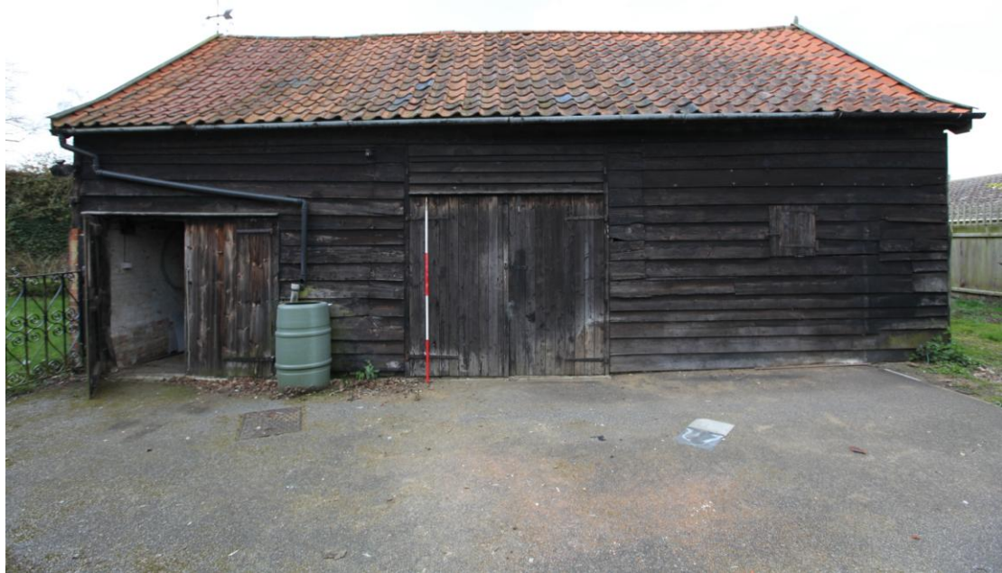
Illus. 5. The eastern facade of the barn showing the 20 th century doors in the position of the original central entrance (bay B) with evidence of taller 19 th century doors in the same position. The southern bay (A) to the left was converted into a separate shed with a first-floor granary in the 19 th century but its present doors also date only from the 20 th century. The pantiles are an alteration of the 19 th century and probably replaced a steeply-pitched thatched roof. Sections of heavily tarred weatherboarding survive from the 19 th century but most has been renewed.
