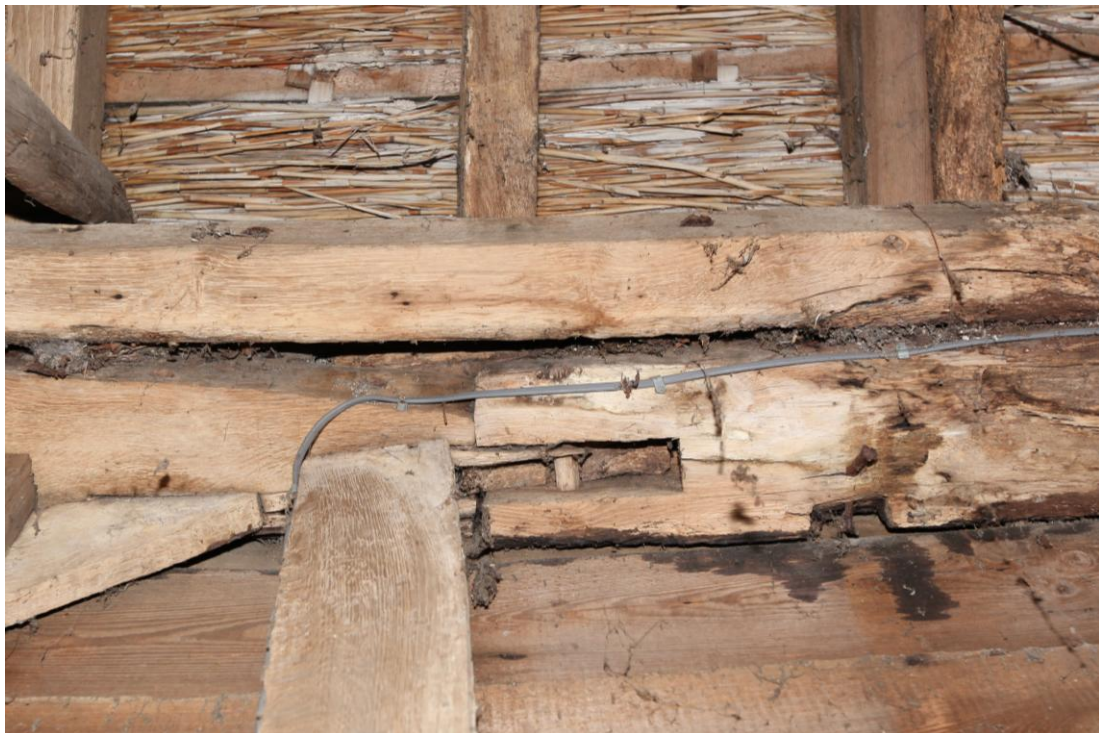
Illus. 10. A detail of the soffit (underside) of the eastern roof-plate in the northern bay (C) showing the tenon of a 16th century type edge-halved and bridled scarf joint. The halving is short at approximately 13 cm (5 ins) in length and the joint was secured by a bolted internal plate in the 19 th century.
