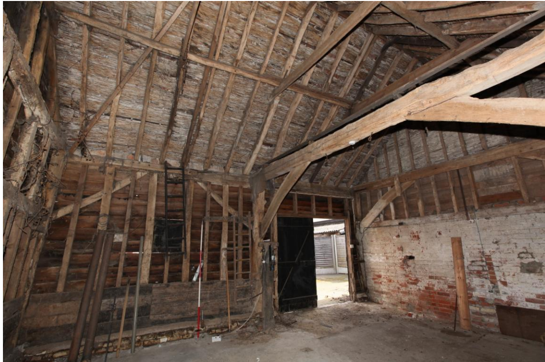
Illus. 9. The eastern interior of the two northern bays (C & B) showing the position of the original entrance to the right and the intact studwork of bay C to the left (with narrow secondary studs nailed in between).
