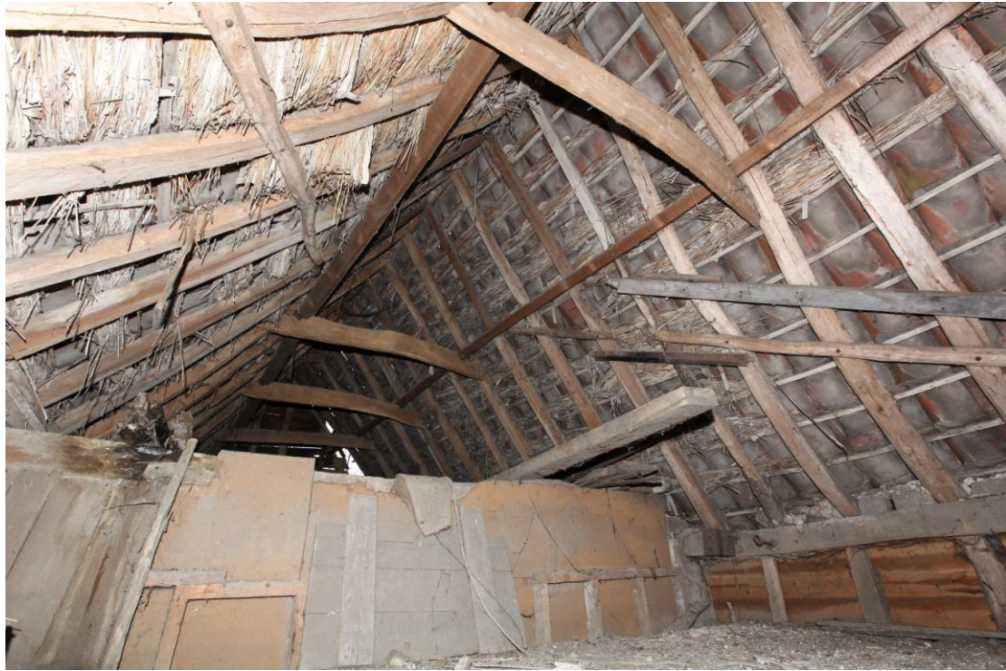
Illus. 11. The intact original roof structure with reed fleaking beneath the secondary pantiles and renewed softwood purlins (looking south from the northern loft, C). The remains of a 19 th century studwork partition are visible against the modern fibre-board which divides the loft from the central bay (B). The steep pitch of the roof suggests it was designed for thatch.
