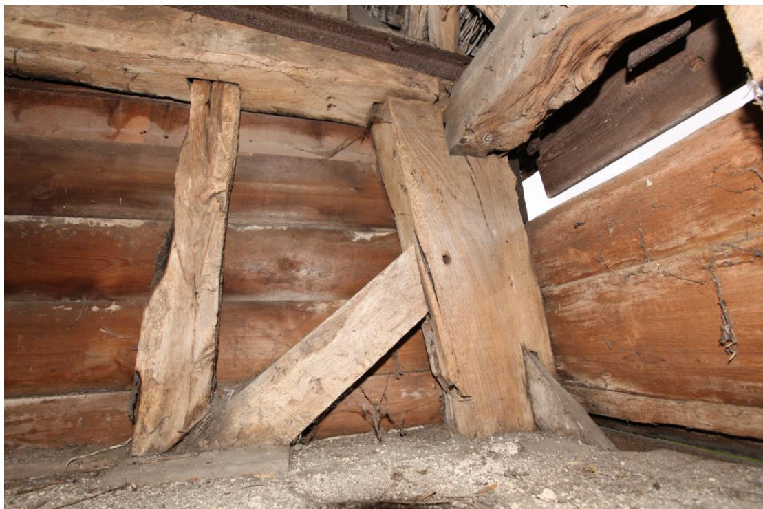
Illus. 12. A detail of the well-hewn jowl of the north-eastern corner post showing the high quality of the oak frame with fully pegged and tenoned primary wall braces interrupting the studs. The common studs are tenoned but not pegged to the tie-beam (left) and roof-plates.
