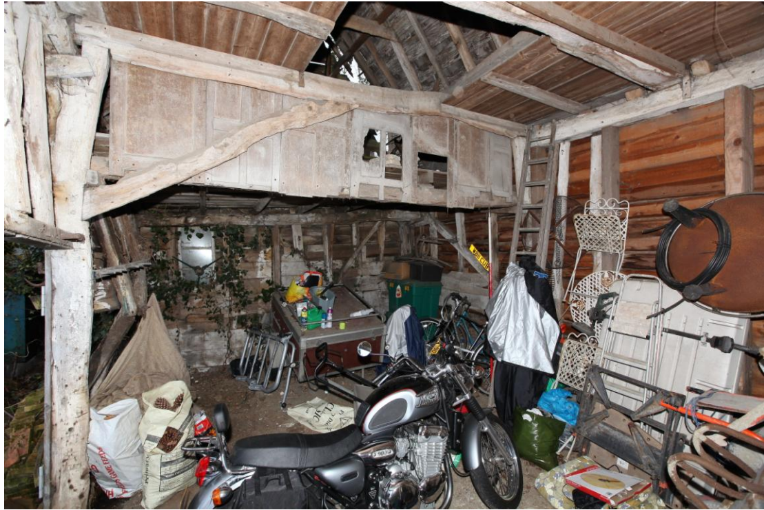
Illus. 7. The interior from the north showing the open truss to south of central bay (B) with an intact arch-brace to the left the empty mortises of its missing counterpart to the right. The partition of the secondary loft consists of re-used 17 th century panelling.
