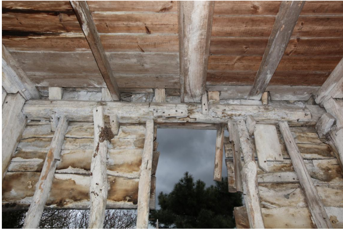
Illus. 9. The eastern roof-plate of the central bay (B) showing a face-halved scarf joint to the right and an unusual single pegged mortise beneath the central flying tie-beam. The present studs are nailed insertions, as are the rafter stubs of the demolished external lean-to. A housing for a central door bar (replacing the original post) has been formed by nailing a fillet of timber to the left of the pegged mortise. The loft is a 20 th century insertion.
