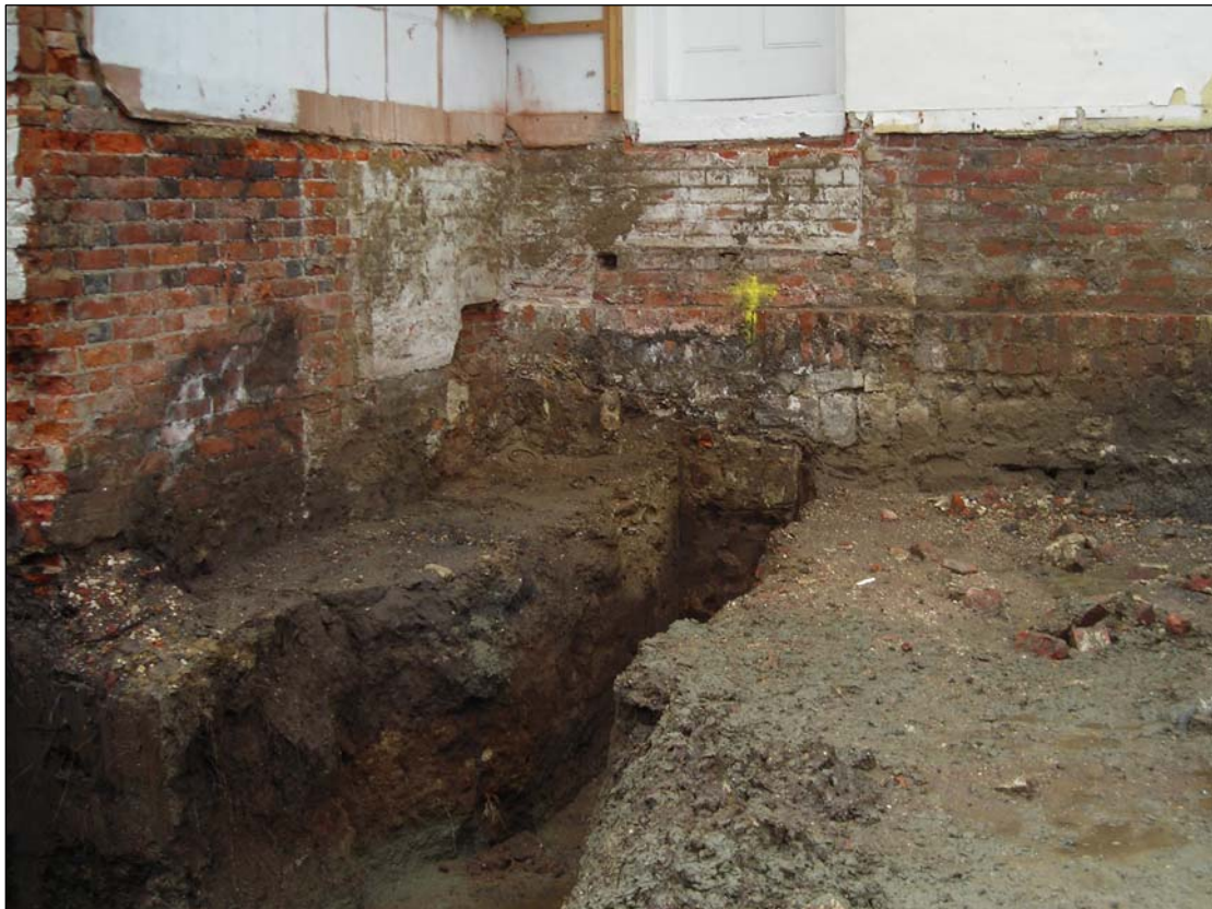
Plate 1. General view showing the eastern excavated footing, and the footings of the existing building
