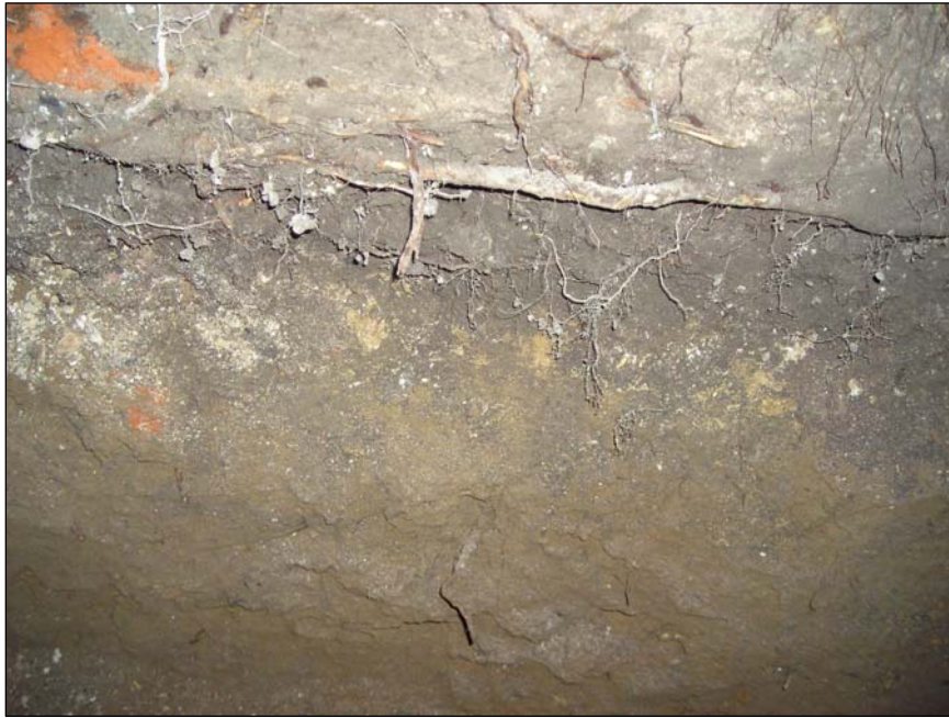
Plate 2. N-S section through the western footings, showing the chalk/mortar layer in the barn interior.
