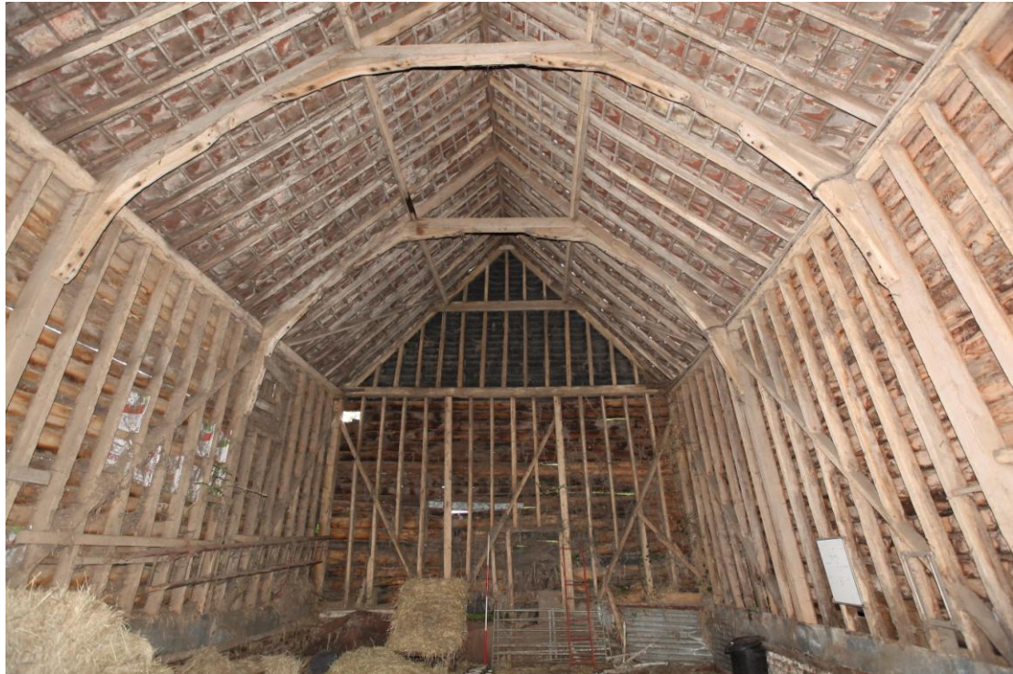
Illus. 9. The eastern bays of the barn (1) showing the remarkably complete original framing with bolted knee-braces linking the principal rafters to both the pegged roof collars and the wall posts (removing the need for horizontal tie-beams and so increasing headroom). The loading hatch in the easternmost bay to the left is an original feature.
