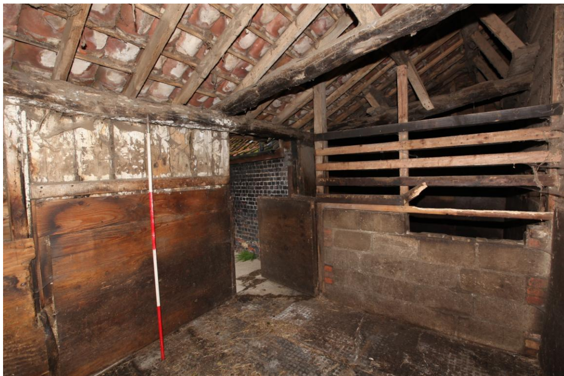
Illus. 6. The interior of the lean-to loose box (4a) adjoining the barn's southern elevation seen from the east (with the weatherboarded wall of the barn to the right). The partitions appear to be secondary but the original roof-plate and tie-beams are charred and may have been re-used after the fire of June 8 th 1822.
