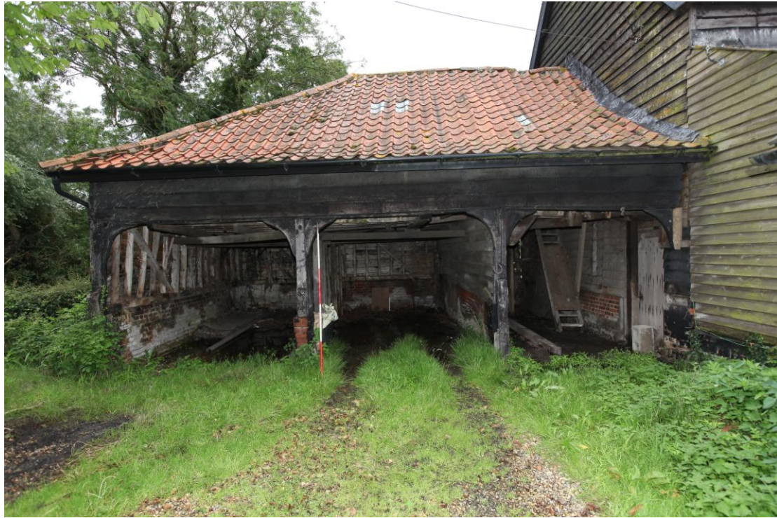
Illus. 3. The open arcade of the well preserved cart lodge (2) from the south showing the heavily tarred weatherboarding of its first-floor granary with the divided eastern bay (2a) containing the stair to the right.
