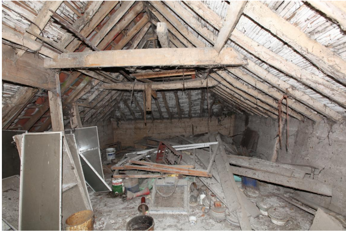
Illus. 5. The interior of the granary above the cart lodge (2) from the east, showing its clasped-purlin roof structure with nailed collars and the boarded internal walls which preserve evidence of removed grain bins.
