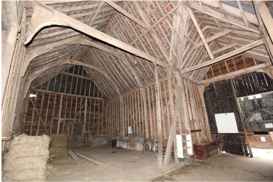
Illus. 7. A general view of the interior of the barn (1) looking south-east from its central threshing floor showing the eastern gable to the left and the integral porch to the right. There is evidence of original full-height doors to both the north and south of the threshing floor.
