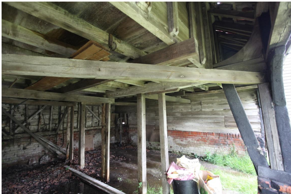
Illus. 4. The interior of the cart lodge (2b) from the west showing the lodged joists and boarded walls of the granary with a reversed knee-brace to the binding joist and various secondary reinforcing timbers.
