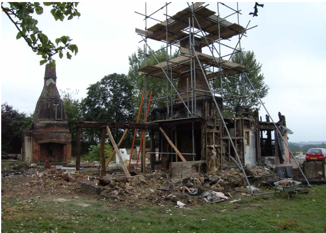
A2.12 General view of site from south-east showing demolition nearing completion (chimneys to remain in situ ).
