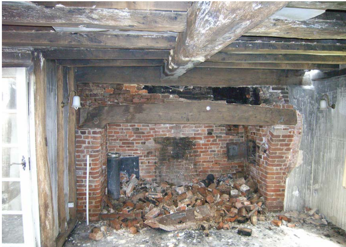
A2.3 Internal view of truss J-I from south, showing partly collapsed fireplace and largely original 17 th century ceiling in room G-J-H-I.
