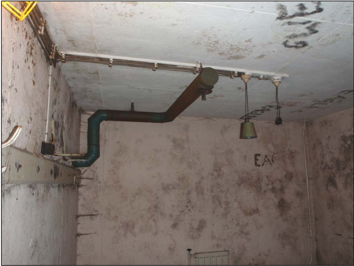
Plate 56. Room B4, air supply pipe and vent (ref. HLY 39)
