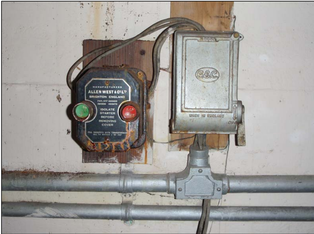
Plate 58. Room B6, air supply pump switches (ref. HLY 19)
