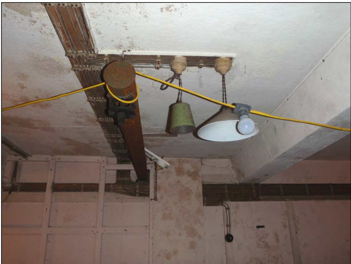
Plate 63. Room B2, multiple light fittings, air supply pipe and vent (ref. HLX 81)
