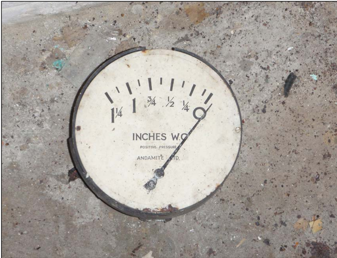
Plate 60. Room B6, air supply pressure gauge (ref. HLY 32)
