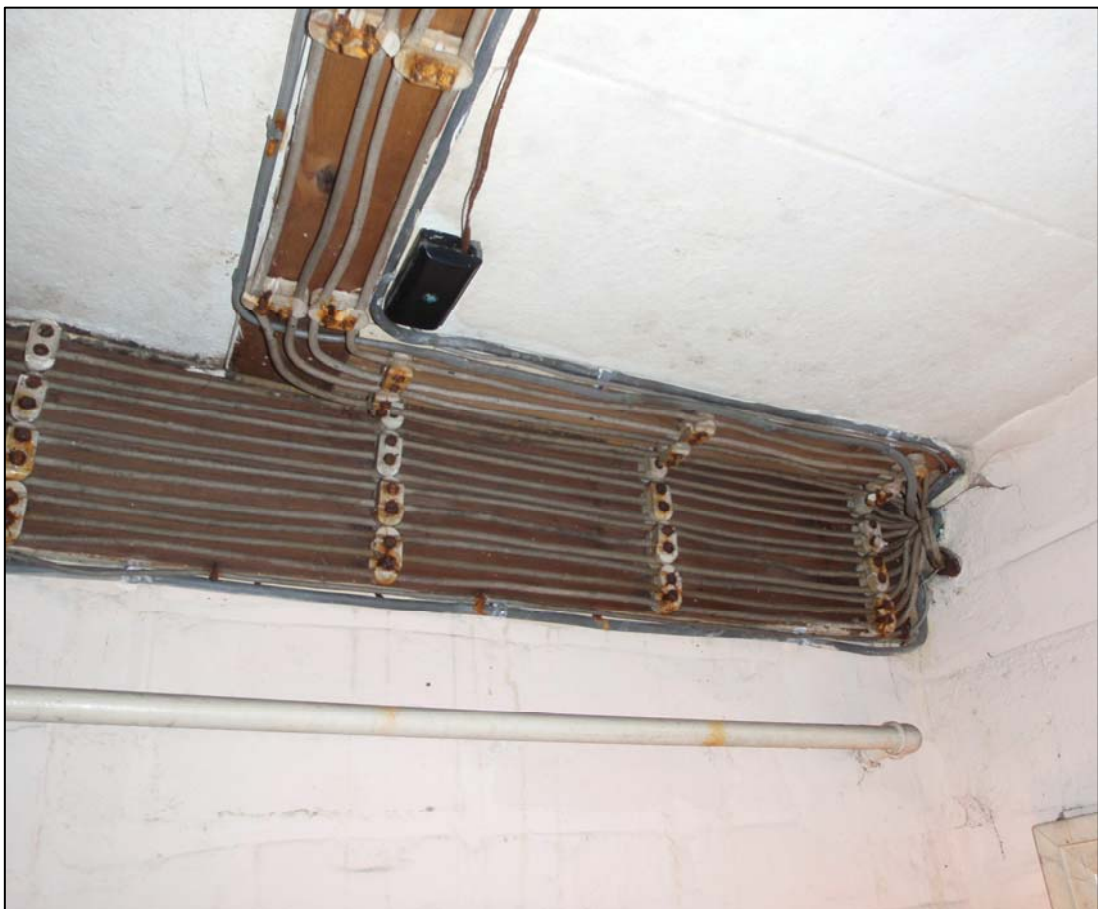
Plate 61. Room B1, electrical wiring (ref. HLY 56)
