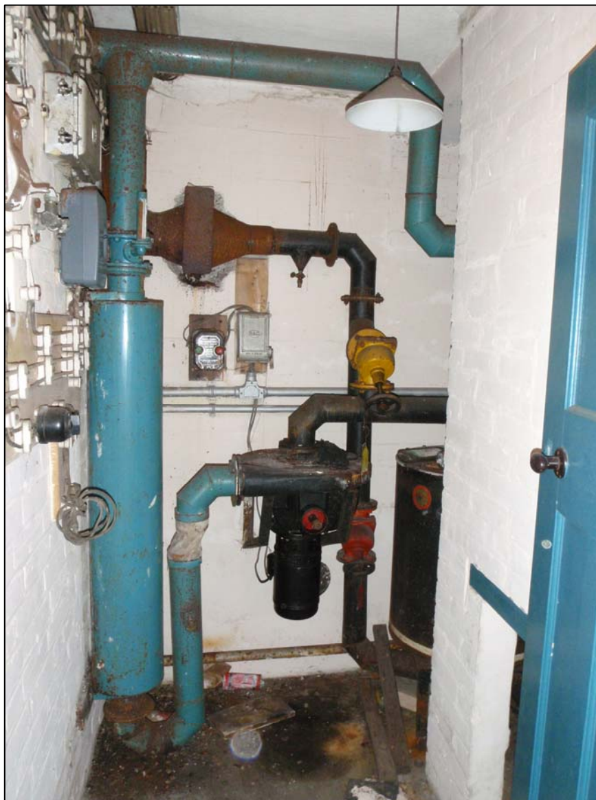
Plate 53. Room B6, air supply equipment, camera facing south-west (ref. HLY 14)
