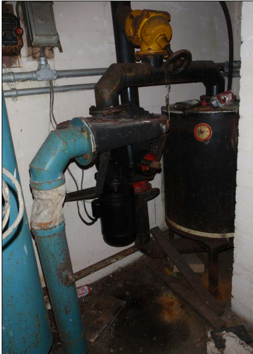
Plate 55. Room B6, air supply equipment - pump and gas filter (ref. HLY 39)
