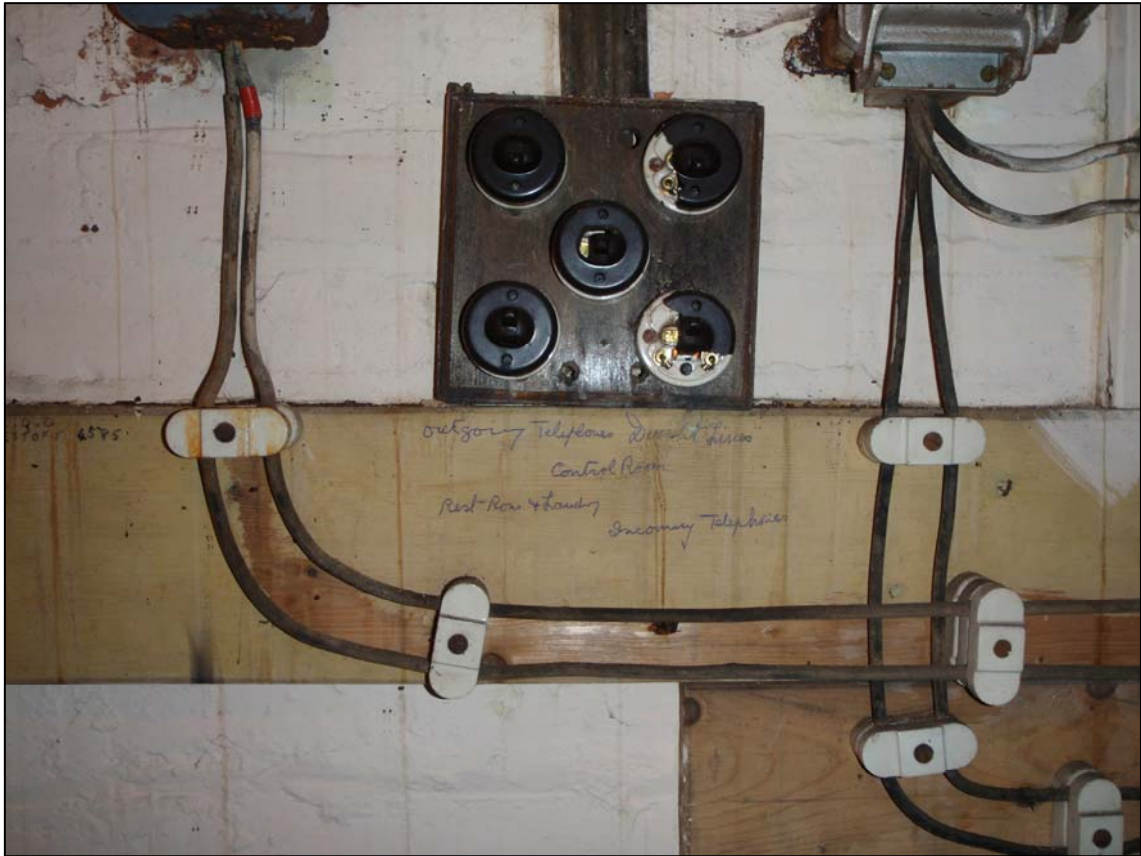
Plate 50. Room B6, switches, camera facing south-east (ref. HLY 15)
