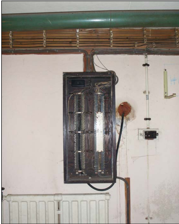
Plate 40. Room B3, telephone wiring box, camera facing south-west (ref. HLY 45)
