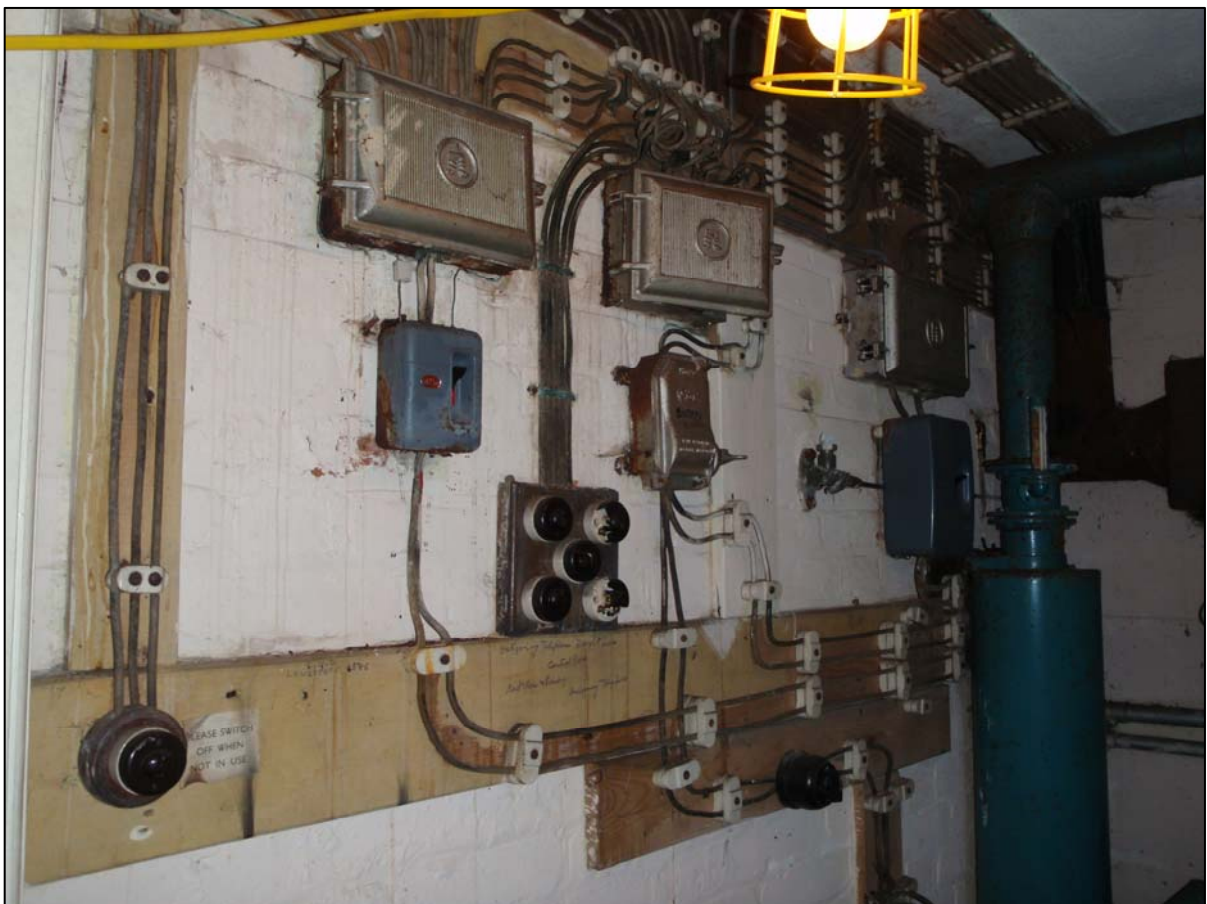
Plate 47. Room B6, fuse boards and switching, camera facing south (ref. HLY 29)
