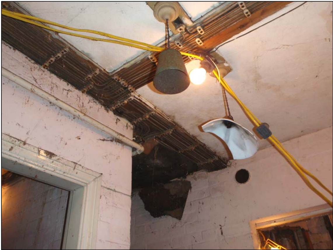
Plate 62. Room G6, electrical wiring (ref. HLX 35)
