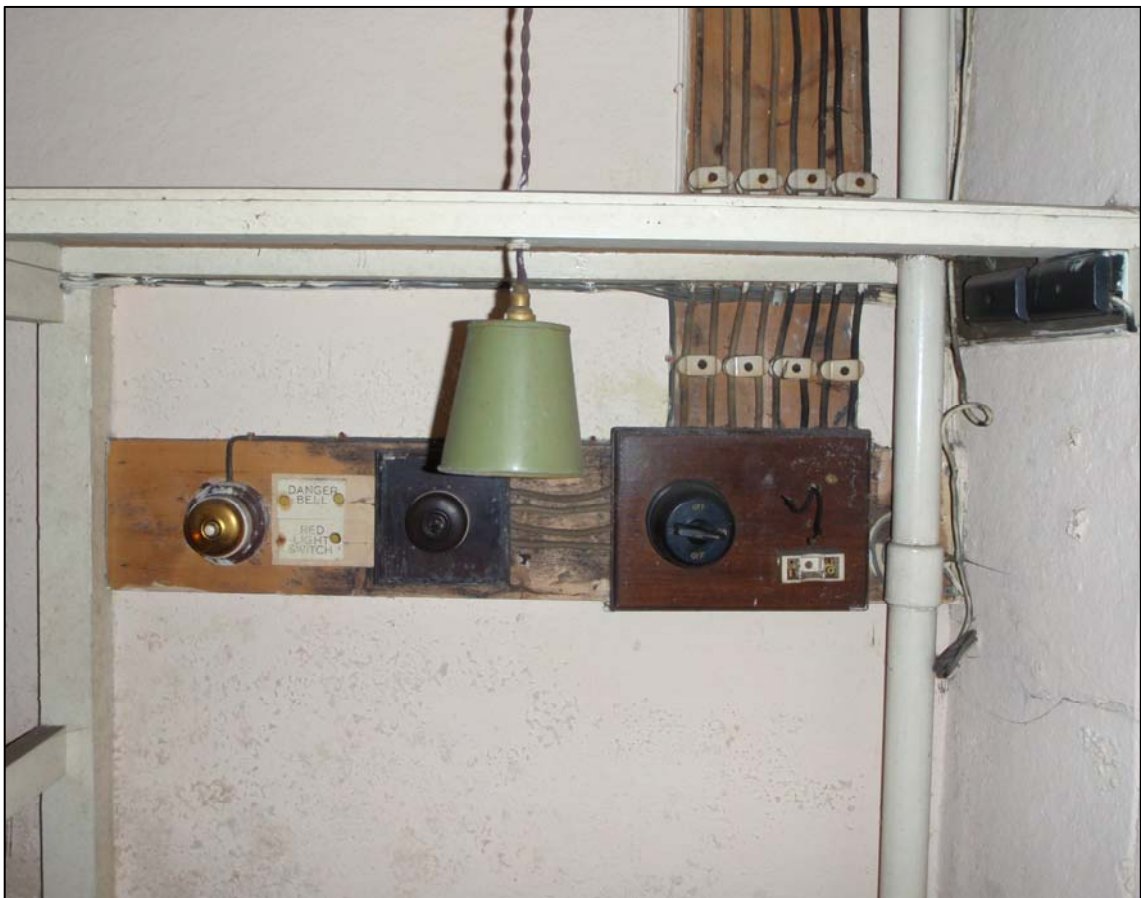
Plate 39. Room B3, switches in southern corner, camera facing south-east (ref. HLX 91)
