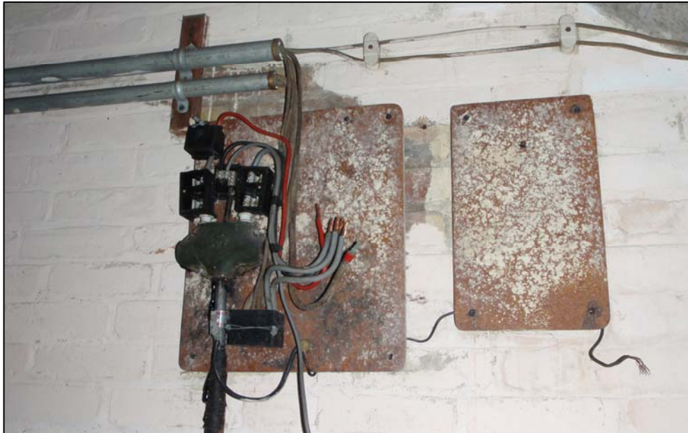
Plate 52. Room B6, power supply and site of ?meter, camera facing north-west (ref. HLY 25)
