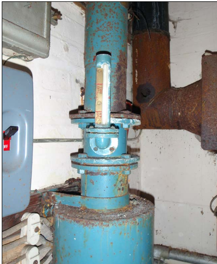
Plate 59. Room B6, air supply flow gauge (ref. HLY 20)
