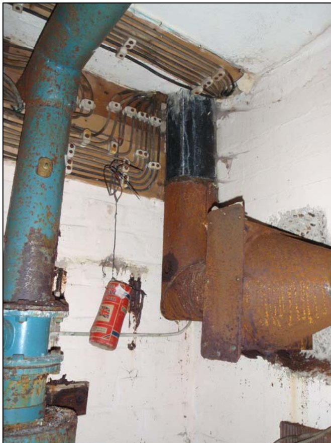
Plate 49. Room B6, battery and air supply filter, camera facing south-east (ref. HLY 28)
