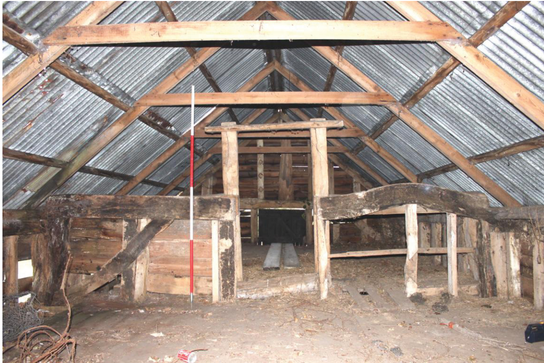
Illus. 5. Interior of eastern loft from east showing the upper part of the sooted medieval 'high-end' partition which divides the building into two halves. Note the original wall brace to the left and the bow in the tie-beam to right. This bow would have reflected an original doorway beneath, which explains the absence of a right-hand wall brace. The central door is an insertion of the 17 th century and the roof is modern.
