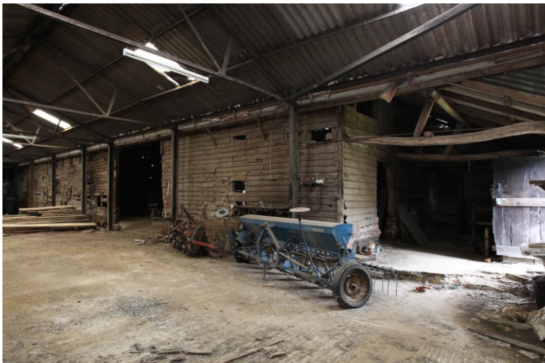
Illus. 10. The unpainted external weatherboarding of the barn (1) from the 20 th century store (4) to the west, showing the remains of the clay-lump lean-to shed (2d) adjoining the south-western gable to the right.
