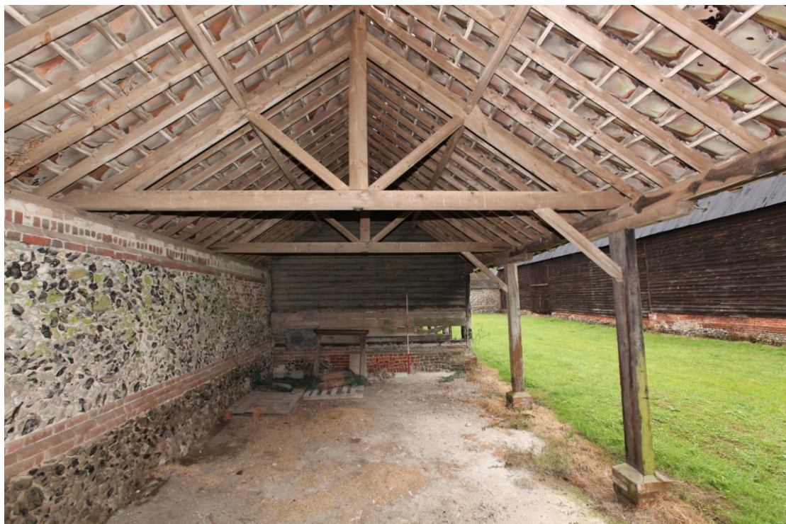
Illus. 6. The interior from the north-east of the shelter-shed (3c) showing its flint-rubble fabric and original king-post roof trusses of machine-sawn softwood. The barn (1) is shown to the right.
