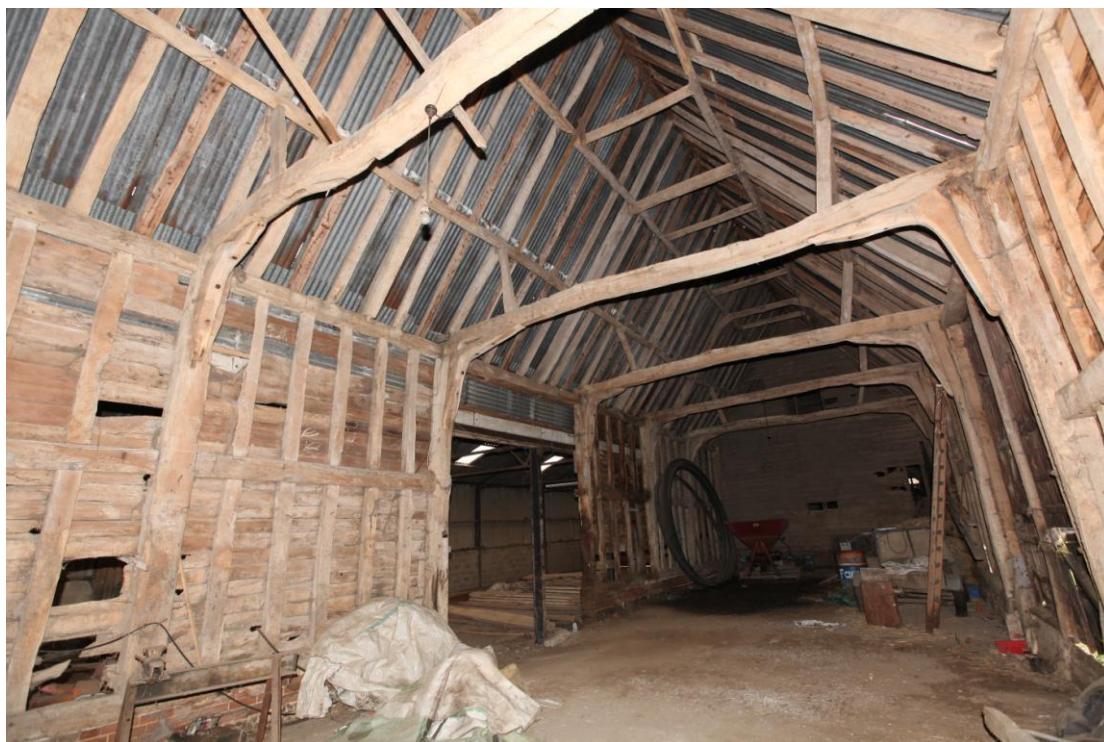
Illus. 14. The six-bay 16th century barn (1a) seen from the south-west. The original arch-braces to the tie-beams have been replaced by bolted knee-braces but the majority of its studs and mid-rails survive with evidence of internally trenched wall braces to all four corners.
