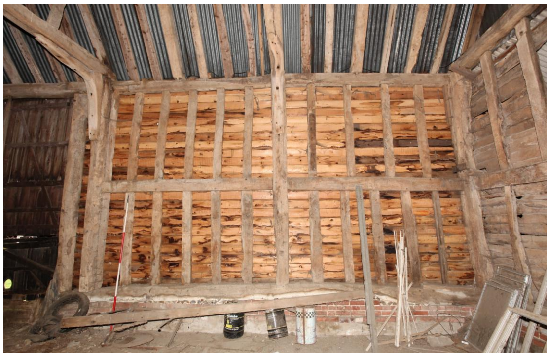
Illus. 16. The south-eastern interior of the western bays of the 16 th century barn (1a) showing the more widely spaced studs of the end-bay to the right. The studs contain mortises for the sill of a window or hatch above the mid-rail, but there is no evidence of mullions in the roof-plate.
