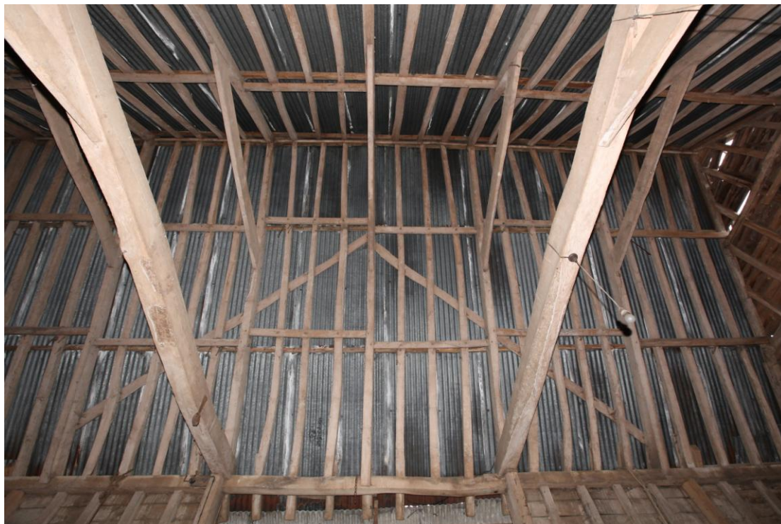
Illus. 13. The diagonal lap boards in the north-western roof of the 18th century barn (1b) reflecting the original gabled roof of the rear porch (1c). The staggered butt-purlin structure, with pegged collars and a ridge-board, is completely intact.
