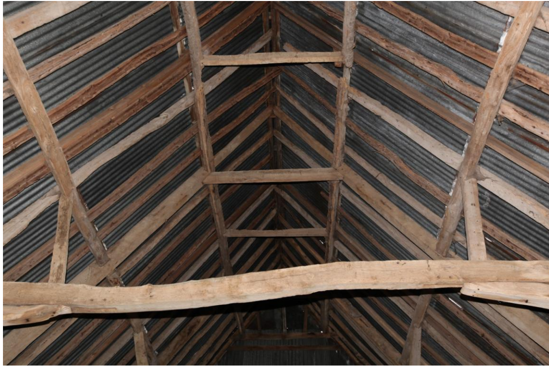
Illus. 17. The roof structure at the south-western end of the 16 th century structure (1a) showing the lower tier of linear butt-purlins and the original clasped-purlins (which have been replaced elsewhere). The principal rafters contain pegged mortises for wind-braces and an anomalous lower collar which suggest a major reconstruction.
