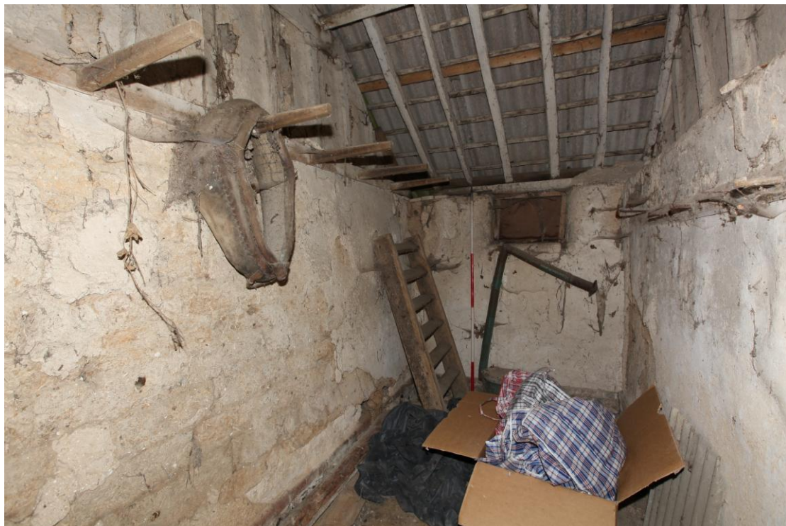
Illus. 8. The southern tack room (2a) from the north-east showing its clay-lump fabric with a leather horse collar hanging on a series of original wooden harness hooks to the left.
