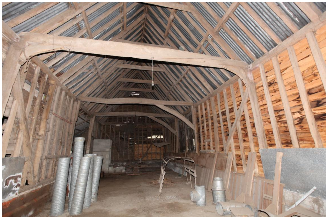
Illus. 12. The interior of the four-bay 18th century barn (1b) from the south-west. The timber frame remains largely intact, with two original arch-braces flanking the south-eastern entrance and bolted knee-braces to the outer tie-beam in the foreground.
