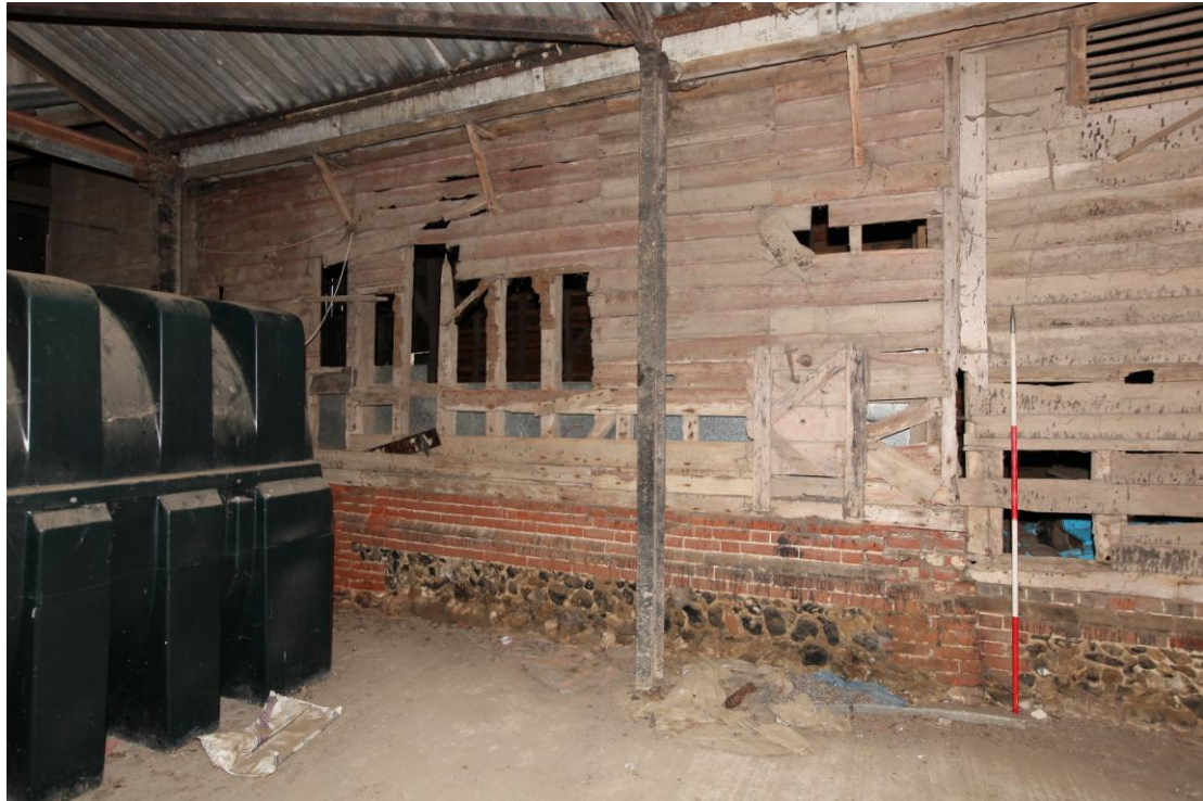
Illus. 11. The weatherboarded north-western exterior of the barn from the 20 th century store (4) showing the junction between its two phases. The boarding of the 18 th century structure (1b) to the left of the scale rod retains traces of original red-ochre pigment, but there is no evidence of colourwash to the 16 th century bays (1a) on the right.
