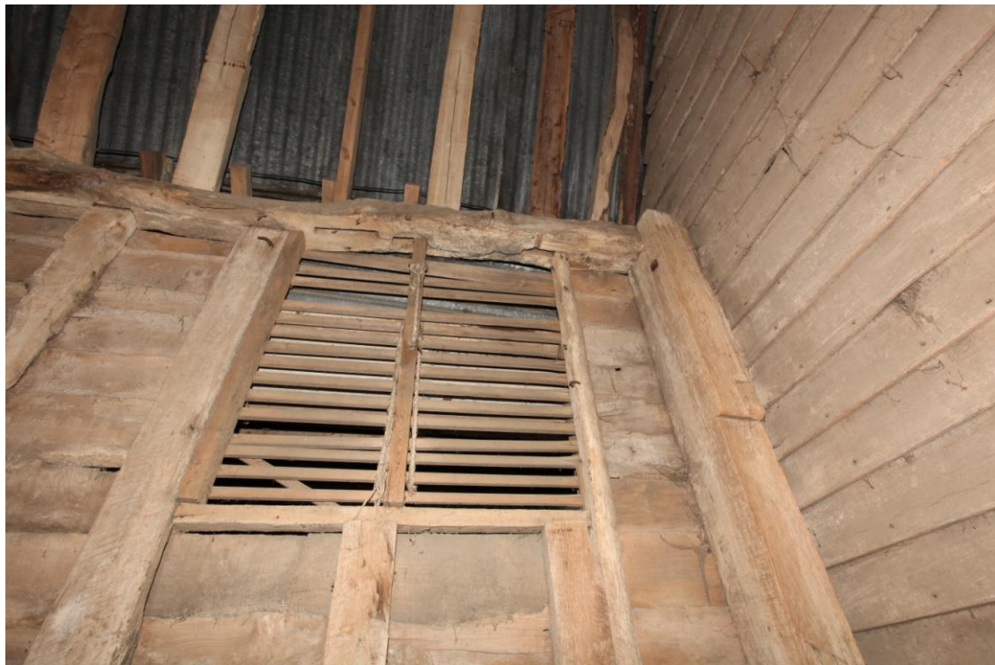
Illus. 18. The 19 th century louver at the north-eastern end of the 16 th century barn's north-western elevation. The roof-plate above contains empty mortises for two original studs and an internally trenced wall brace, but there are no corresponding mortises in the right-hand corner-post which is a later replacement.
