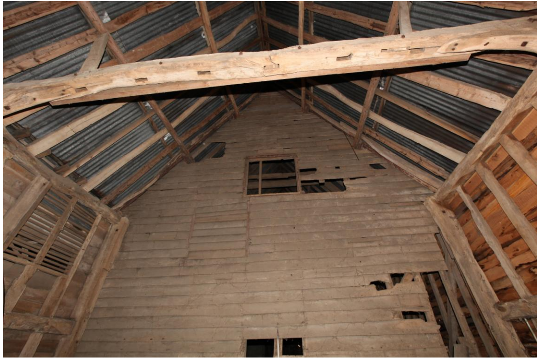
Illus. 15. The north-eastern end of the 16 th century structure (1a) showing the intact weatherboarding of the 18 th century structure's external gable complete with red ochre pigment to its projecting rafters and hatch rails. The framing of the 16 th century gable is lacking and the left-hand post is a replacement – suggesting that the earlier barn was moved to its present position only after the completion of the 18 th century barn. The tie-beam above contains empty mortises for an internal stable partition.
