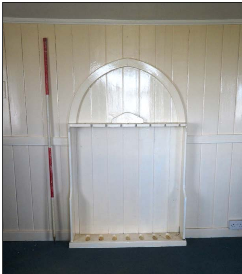
Plate 32. rack, first floor (ref. HQD 25)
