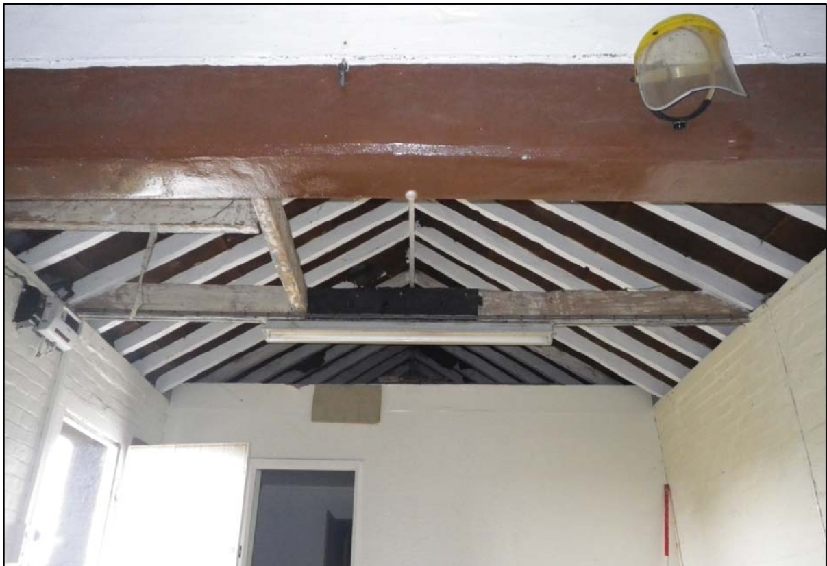
Plate 14. Structural beam and roof structure, some additional, non-structural, beams are also visible (ref. HQD 04)
