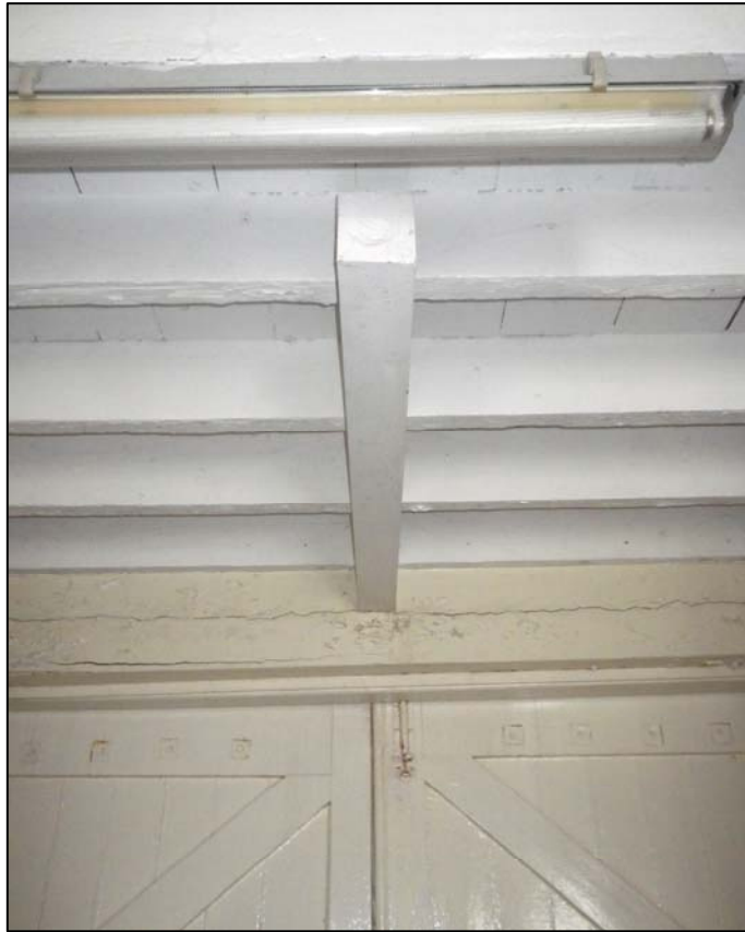
Plate 15. beam supporting the first floor bay window and underside of floor (ref. HQD 08)
