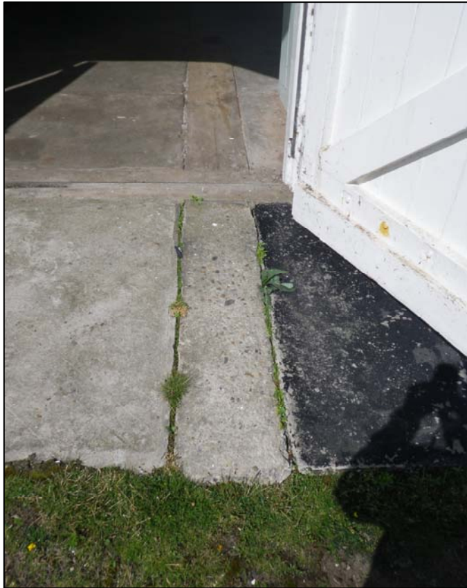
Plate 19. site of timber track in the concrete surface of exterior ramp (ref. HQC 73)
