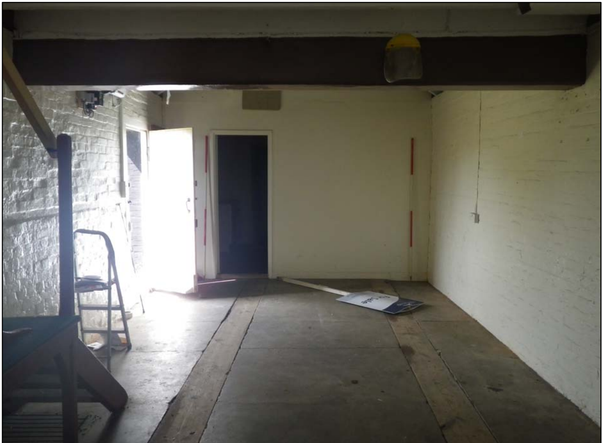
Plate 18. general view of the interior of the building, camera facing west (ref. HQC 92)
