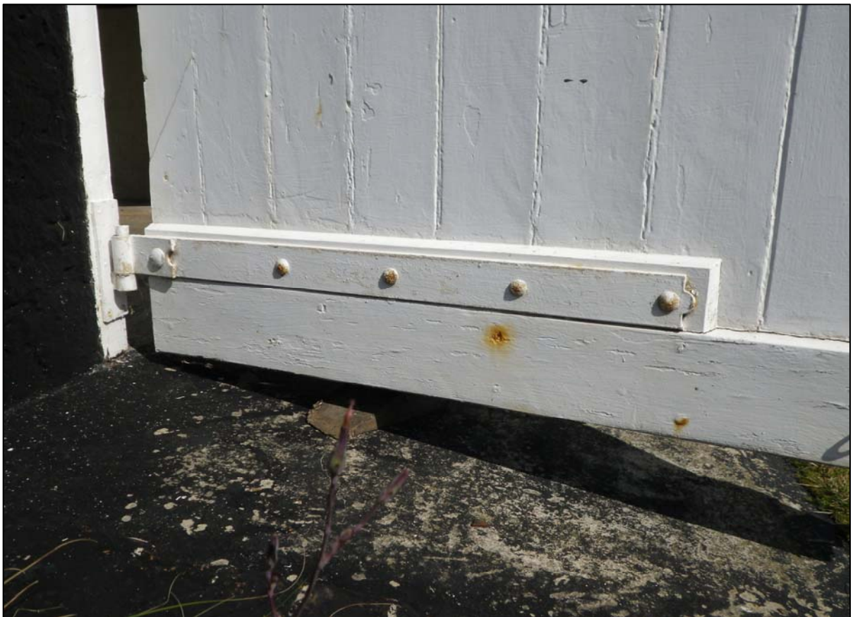
Plate 10. lower right hand hinge on the double doors in the eastern façade (ref. HQC 67)
