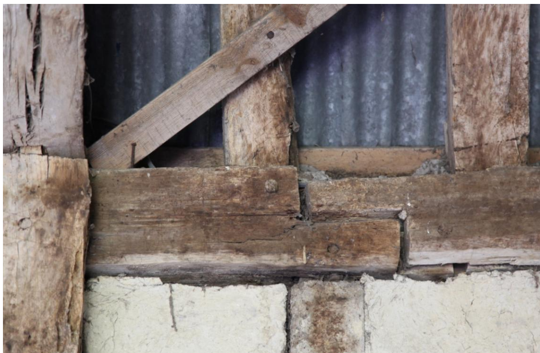
Illus. 10. A detail of the 16th century-type edge-halved and bridled scarf joint in the western roof-plate of bay C. Joints of this kind were quickly superseded during the first quarter of the 17 th century.
