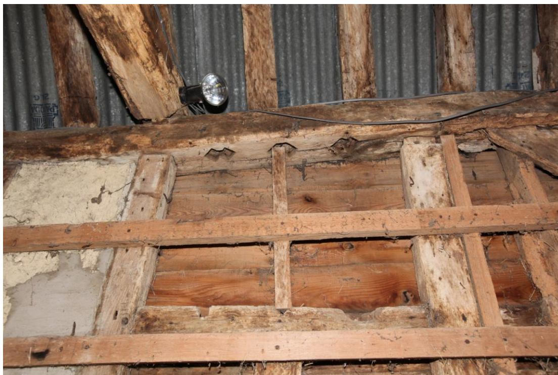
Illus. 11. A detail of the unusual ‘double’ diamond mullion mortises in the western roof-plate of bay D with the original window sill beneath. This window lit the missing loft, and its mortises relate to the correction of an error by the carpenter who seems to have intended four mullions before realising there was only room for three. The eastern window immediately opposite was 20 cm wider (8 ins) and was able to accommodate four mullions. The error was not repeated in the sill.
