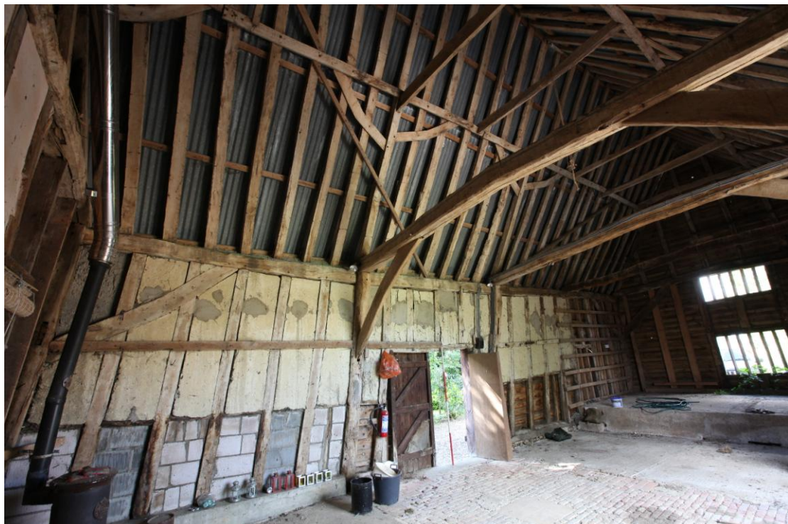
Illus. 8. The barn's internal western elevation showing the largely intact wall and roof framing with a 20th century concrete platform in the northern bay (D) to the right. The wattle-and-daub between the studs appears to be original (with recent patching in cement) but has been replaced by cement block-work where it adjoins the lower tier of external weatherboarding shown in illus.5 above.
