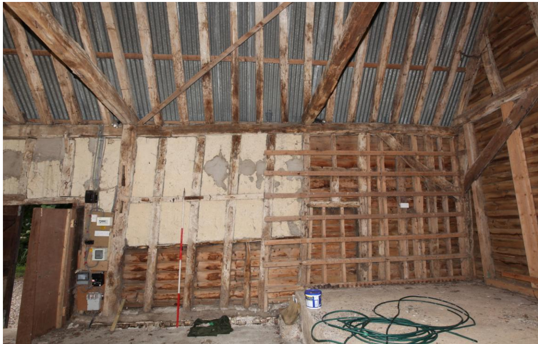
Illus. 9. The western interior of the two northern bays (C and D), divided by a tie-beam and principal roof truss but not a storey post. These bays were originally floored over at the height of the horizontal batten 2 m above the present ground level in bay C to the left, and there is evidence of original ground and first-floor windows to the right. The battens of bay D are modern and probably relate to the use of the raised concrete platform as a grain store.
