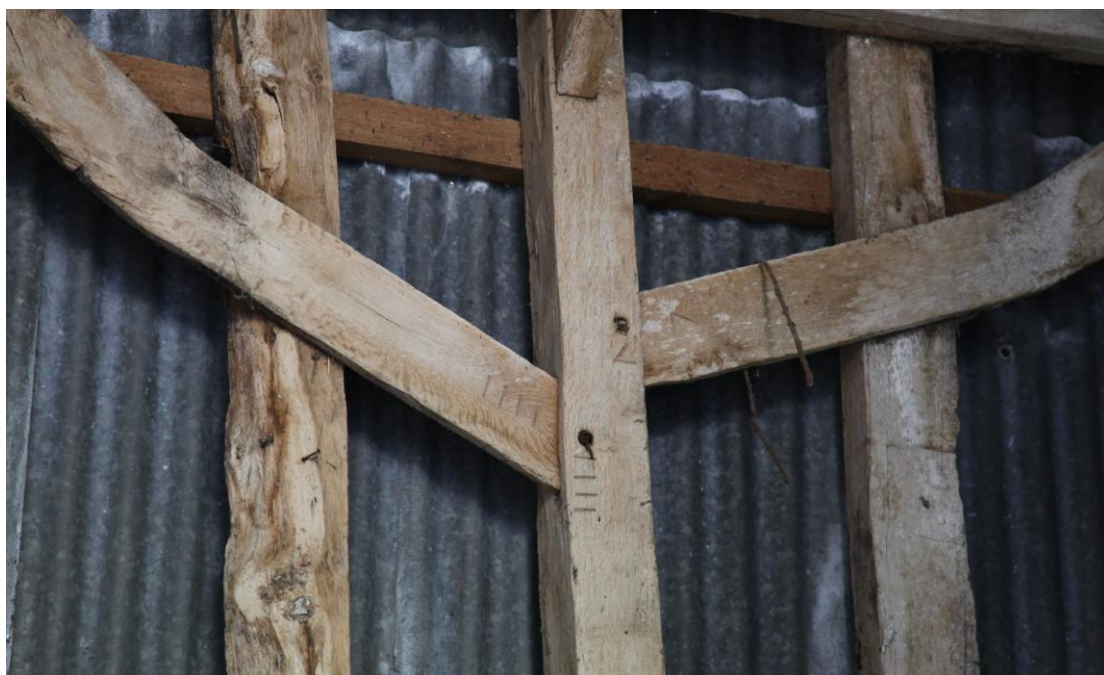
Illus. 12. Detail of the chiselled Roman carpenter's numerals III and V to the western reverse-cranked wind-braces between bays B and C. Chiselled marks of this type (as opposed to scored marks) are typical of the 17 th century and later, and are rarely found in conjunction with edge-halved scarf joints.
