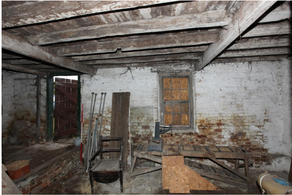
Illus. 9. The internal south-western facade of the early-19 th century shed (2) showing the entrance and stair platform at ground level to the left with the sunken floor and original 6 over 6 sash window to the right.
