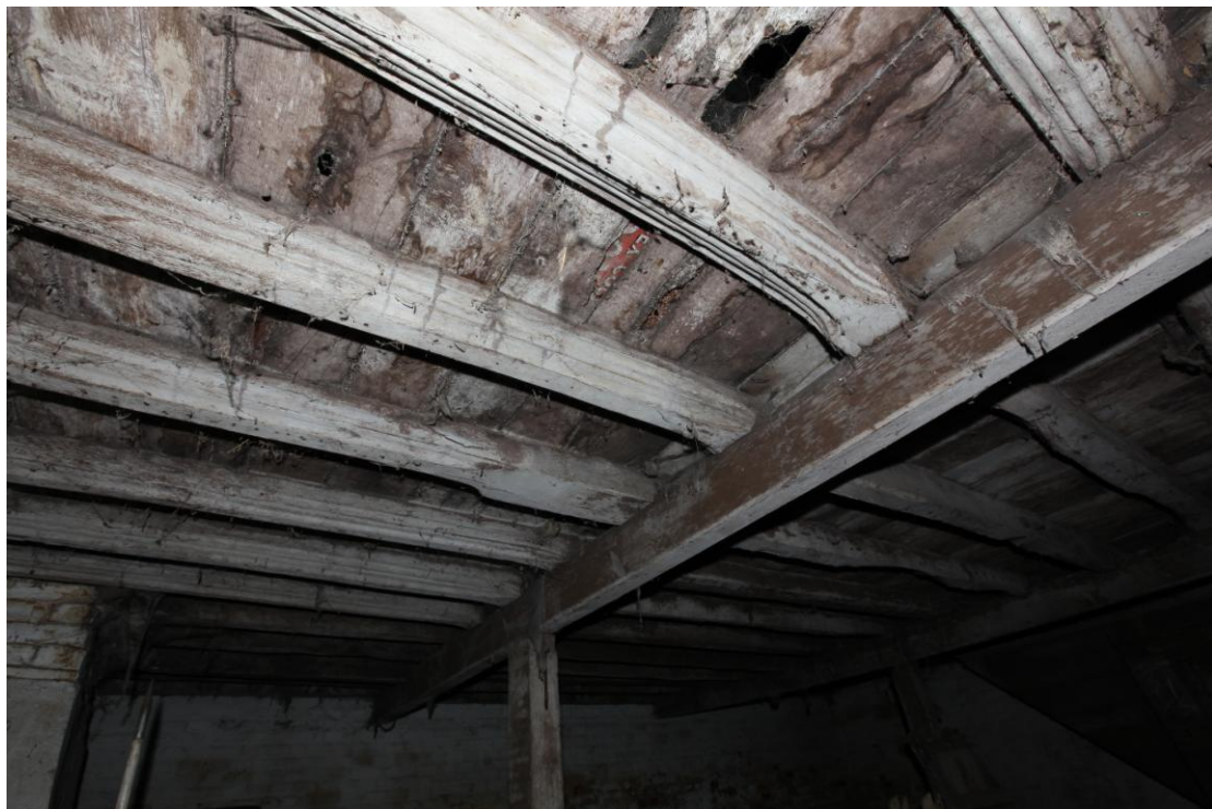
Illus. 8. The re-used late-15 th or early-16 th century ogee-moulded joists in the three-bay ceiling of the early-19th century shed (2), viewed from its southern corner. Several joists show evidence of a jetty, and were probably salvaged from the buildings in the rear courtyard of the nearby grade II-listed range (illus. 1) which were in the same ownership and demolished at or around the time of the shed's construction.
