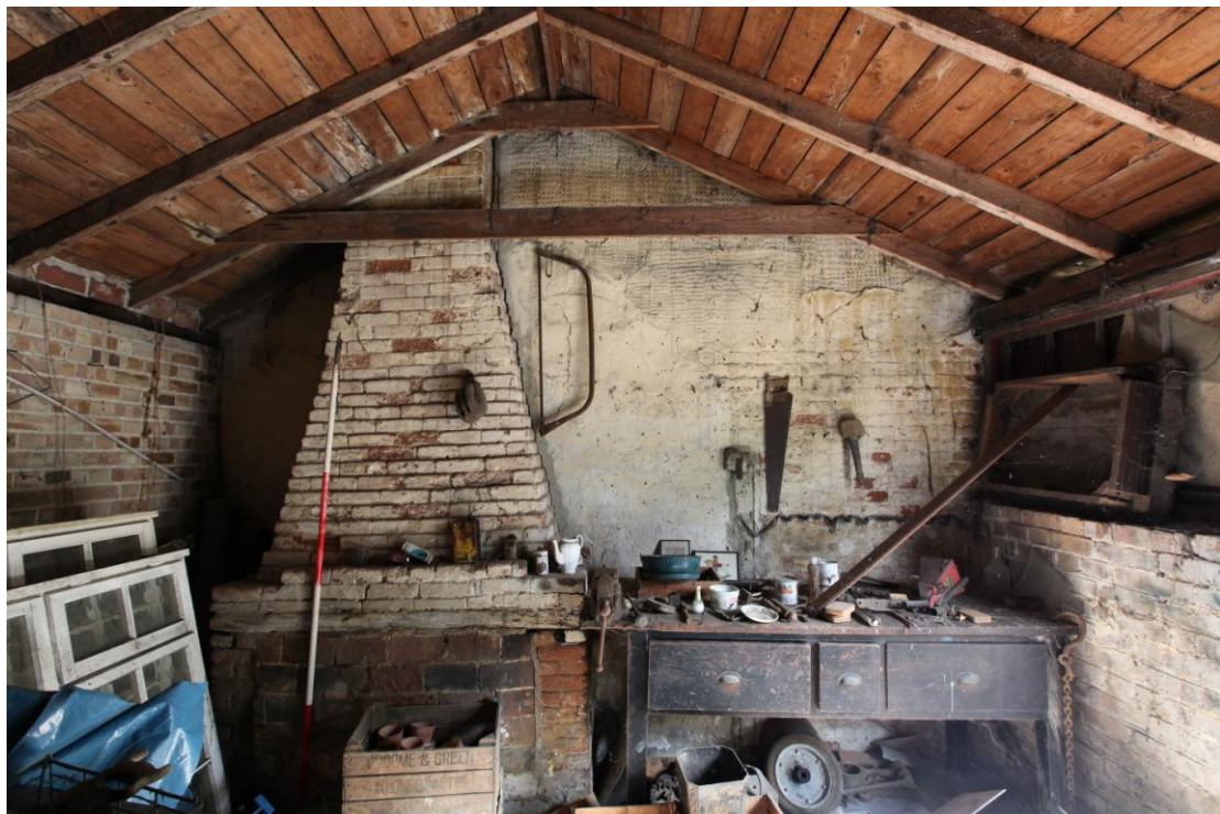
Illus. 4. The interior of the 20 th century vehicle shed (1) from the south-west showing the early-19 th century chimney and blocked fireplace with the truncated roof plate of an earlier, smaller shed to the right. The profile of this earlier shed is clearly visible in the plaster on the gable of the early-19 th century shed (2) which preserves original external pargeing above the whitewashed brickwork of its lower storey.
