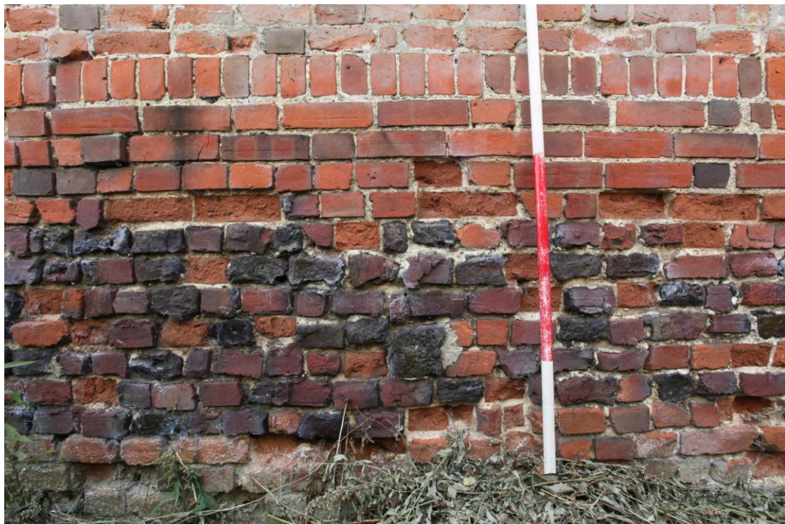
Illus. 14. A detail of the re-used over-fired brick-kiln wasters in the low 19 th century boundary wall (capped by a soldier course – i.e. a row of headers set on edge) incorporated into the north-western rear elevation of the mono-pitch shed (4) and part of the late-19 th century shed (3). These wasters probably stem from the Garrad brickworks beside the railway at the foot of Lamarsh Hill in Bures Hamlet.
