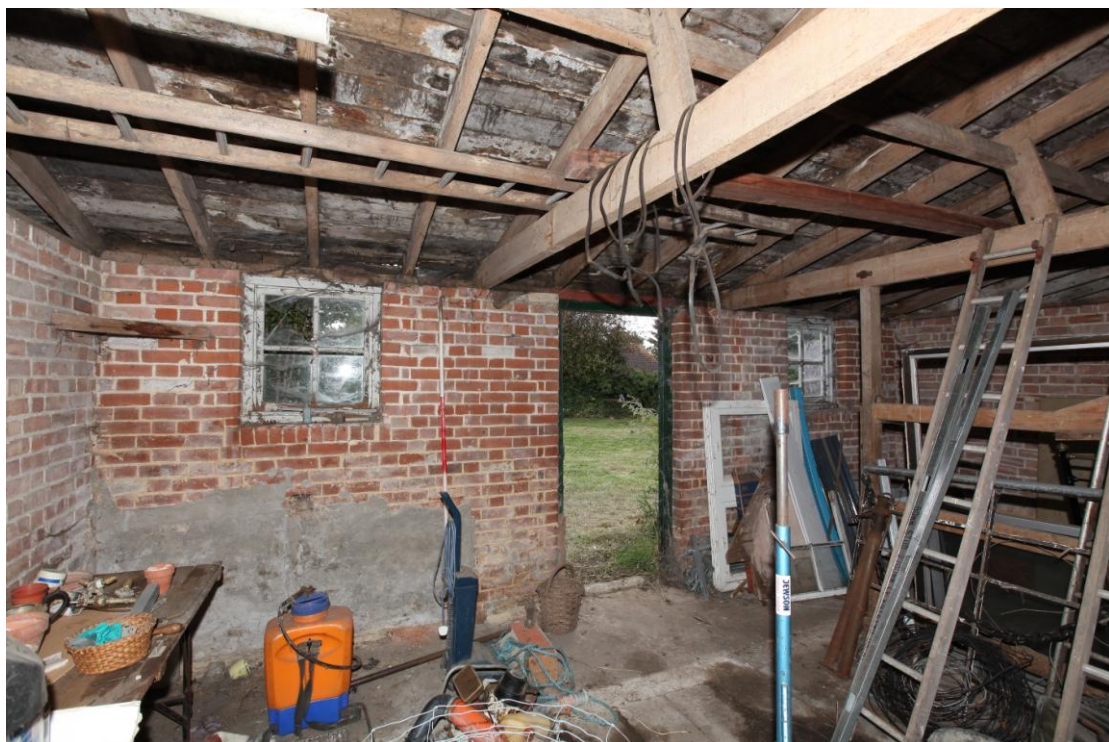
Illus. 16. The south-eastern facade of the central compartment (4b) of the mono-pitch shed showing its boarded roof and central door flanked by original windows. The remains of two original boarded stall divisions are visible to the right and this compartment was designed as a stable.
