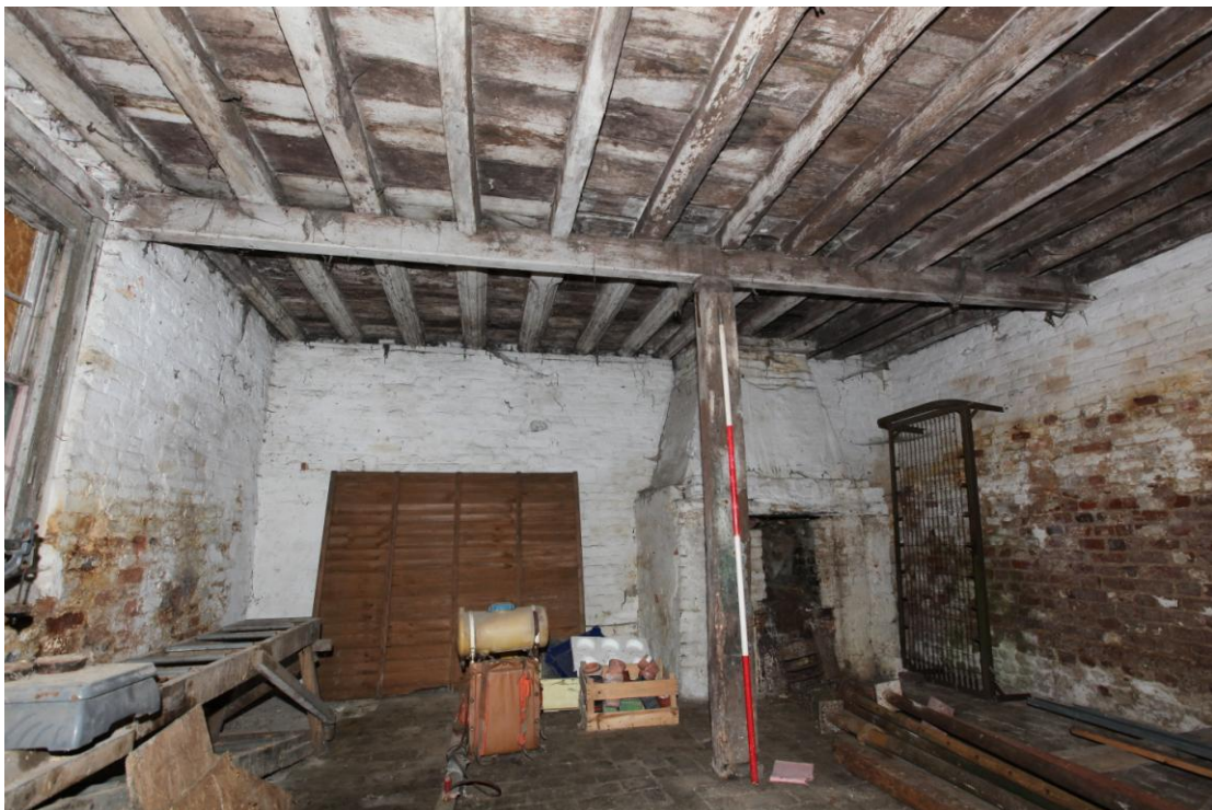
Illus. 6. The interior of the early-19 th century shed (2) from the north-east showing its intact sunken brick floor, original fireplace and re-used late-medieval ceiling joists.
