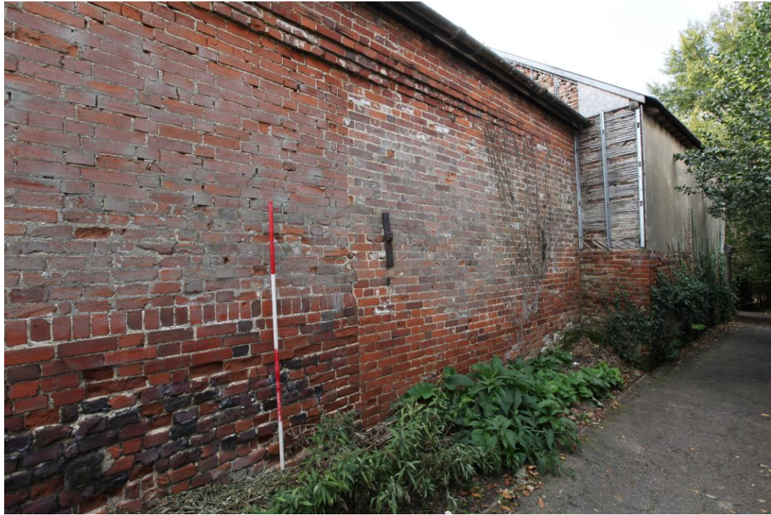
Illus. 13. The ‘blind’ north-western exterior of the late-19th century shed (3), viewed from the tarmac of the adjoining footpath and showing three phases of brickwork with the former low boundary wall at bottom left. The wider early-19 th century shed (2) is visible in the rear to the right.
