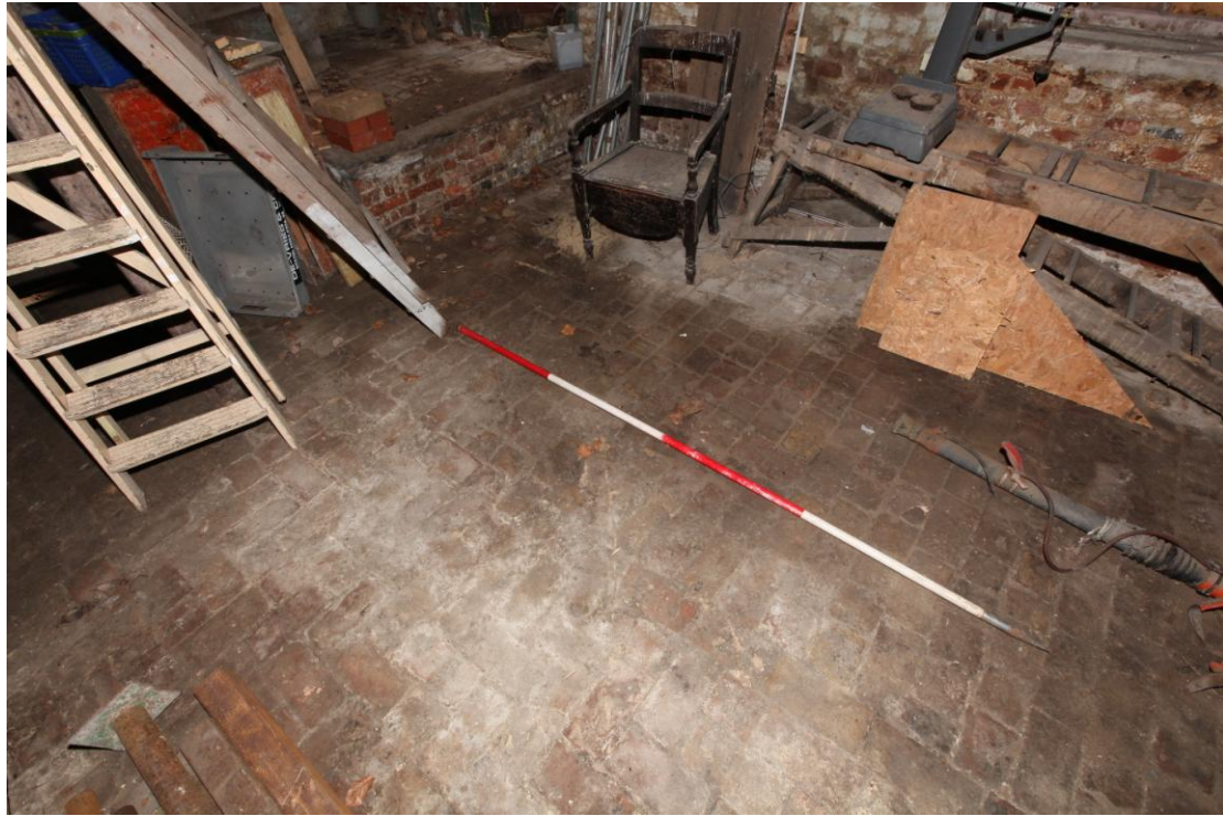
Illus. 11. A detail from the west of the well preserved original sunken brick floor of the early-19th century shed (2) with the entrance platform to the left.
