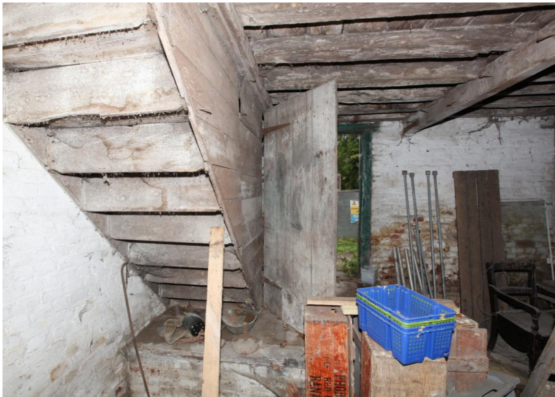
Illus. 10. The underside of the boarded stair in the eastern corner of the early-19 th century shed (2). This rests on a brick platform at ground level with the rest of the floor 0.5 m lower.
