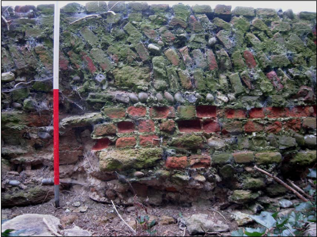
Plate 45. E. precinct wall: external, representative example of brick patching
