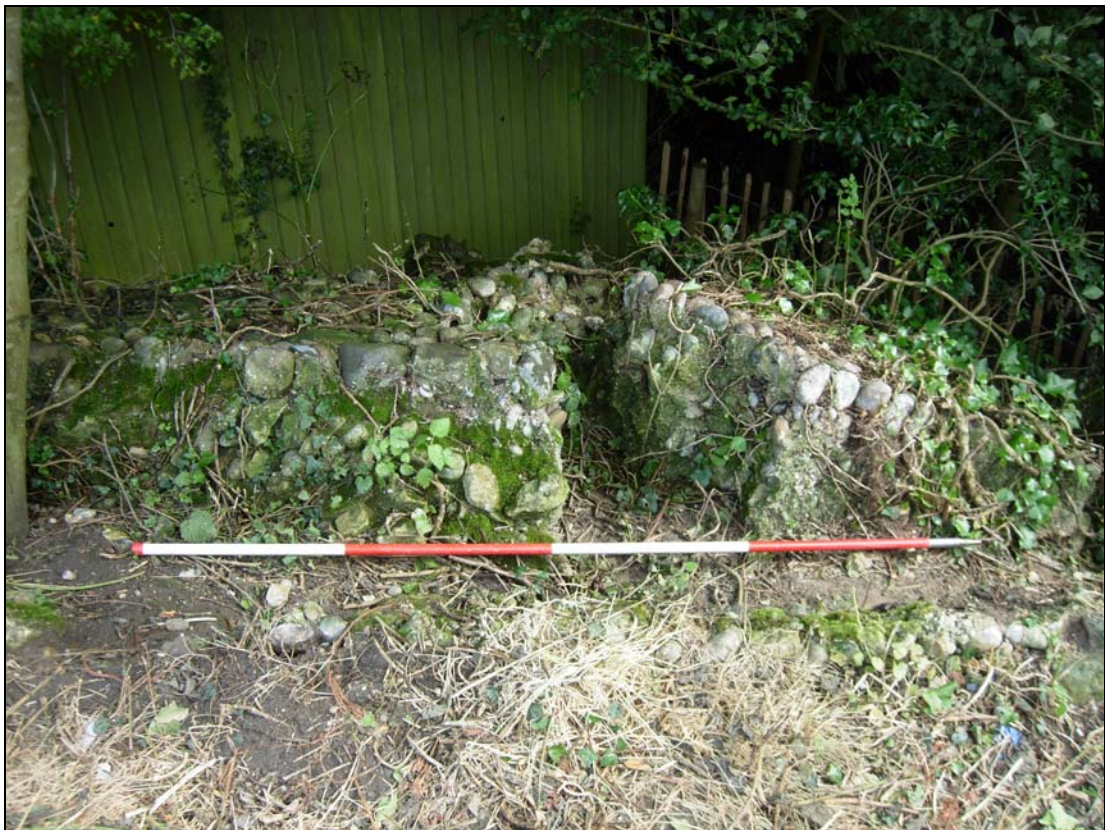
Plate 2. N. precinct wall: detached blocks on external slope
