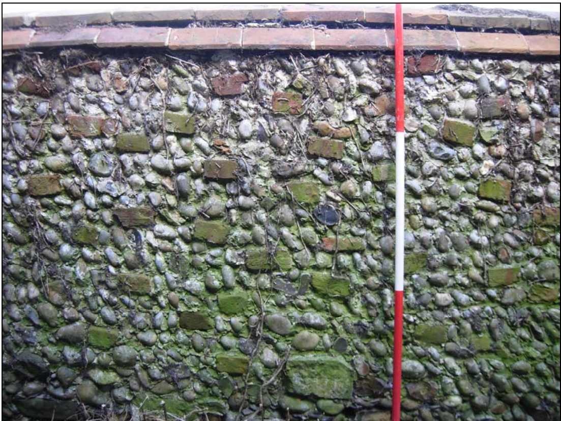
Plate 70. S. precinct wall: external, example of intact face
