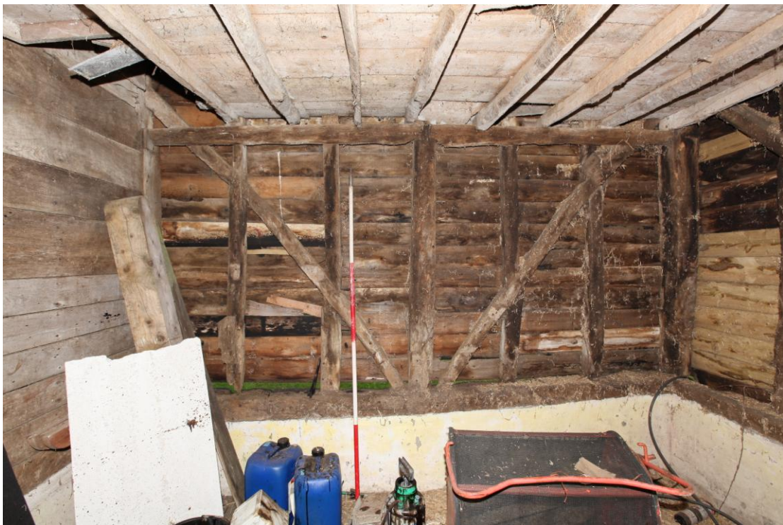
Illus. 10. The northern interior of the stable (1b) showing its original framing and the clamp (rail) which supports the ends of the original ceiling joists with the hay drop (aperture in ceiling) to the left.
