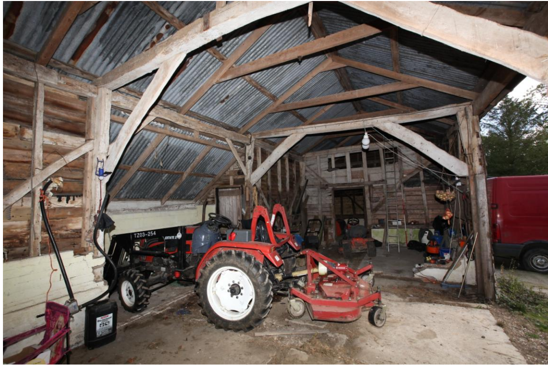
Illus. 5. A general view of the three-bay threshing barn (1a) from the west showing its intact tie-beam braces and mid-20 th century softwood roof structure. The lean-to rear porch (1c) adjoins the central bay to the left but the threshing floor has been replaced or covered by concrete. The roof-plate above the original southern entrance to the right was replaced in the 20 th century.
