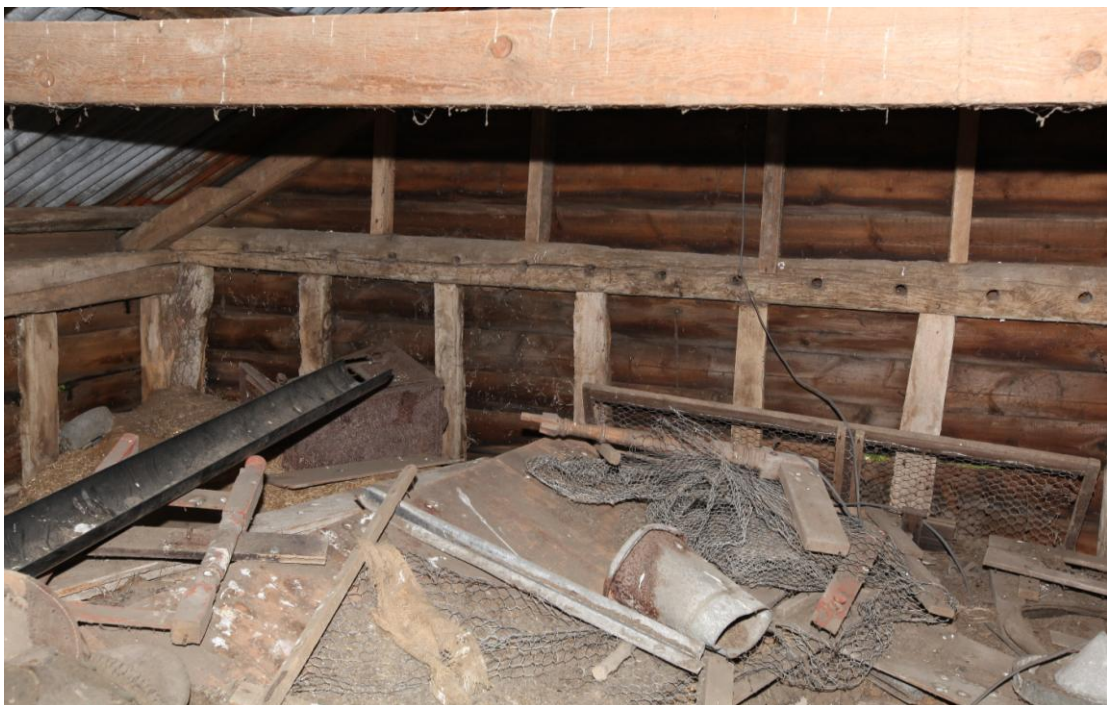
Illus. 12. The internal north-eastern corner of the hay loft above the stable (1b) showing the unusual series of dowel holes in the tie-beam of the eastern gable to the right. These penetrate the timber and may have been intended to secure an external pentice board or canopy above the stable's entrance. There is nothing to suggest the timber is re-used.
