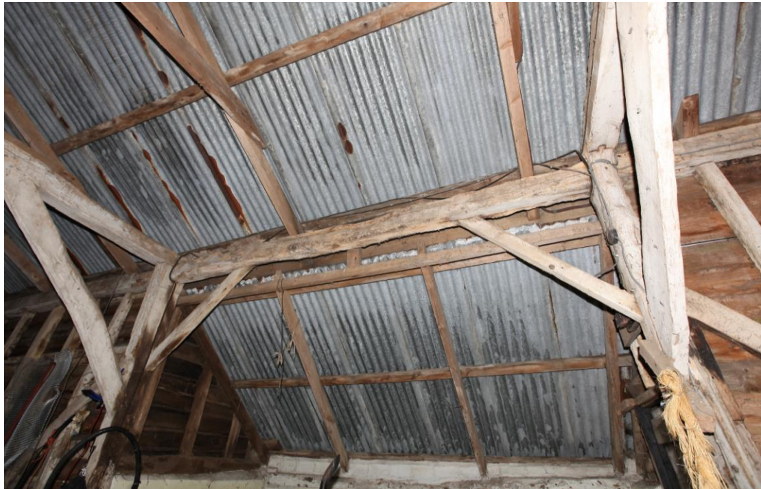
Illus. 8. A detail of the northern roof-plate of the threshing barn (1a) adjoining its central lean-to porch (1c), showing the original tenoned & pegged braces from the storey posts. These braces demonstrate that a porch must have existed here from the outset, although the present structure has been rebuilt in cement block-work and its roof-plate (which may be a re-used timber) contains no evidence of a central door.
