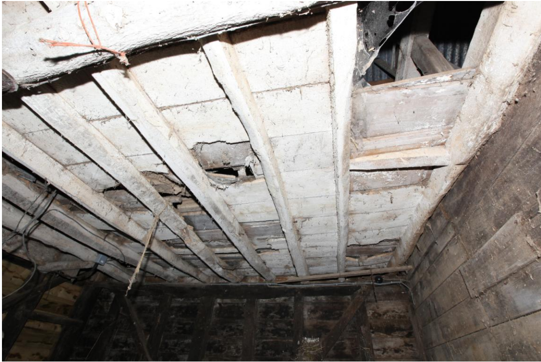
Illus. 11. The original ceiling joists of the stable (1b) from the north, showing the partly blocked hay drop above the missing hay rack against the internal partition to the right. The whitewashed floorboards adjoining the southern elevation appear to be original, and the hay drop did not span the entire width of the building. The original tapered strut to the right is one of two that survive.
