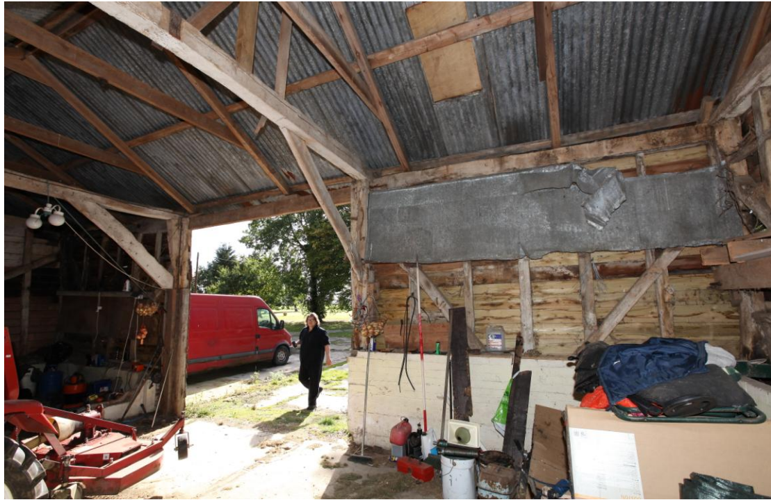
Illus. 7. The southern interior of the threshing barn (1a) showing the original entrance in the central bay (lacking its doors and roof-plate) with the brick internal walls of a 20 th century grain bin in the western bay to the right. The wall framing survives largely intact with primary braces that are tenoned and pegged to the jowled storey posts and ground sills.
