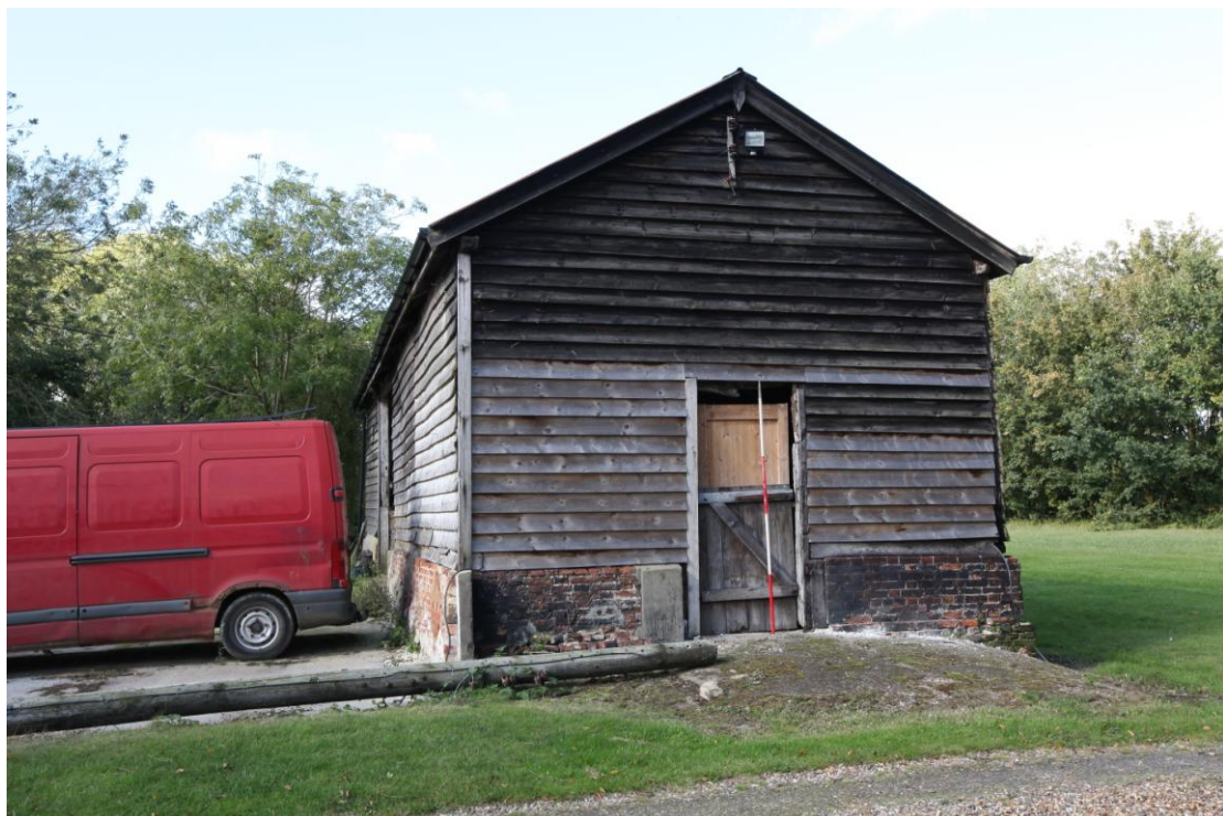
Illus. 4. The eastern external gable showing the original entrance to the stable (1b) which is respected by the rebuilt brick plinth to the right. The original plinth to the left is cement-rendered and consists largely of re-used 16 th and 17 th century bricks.
