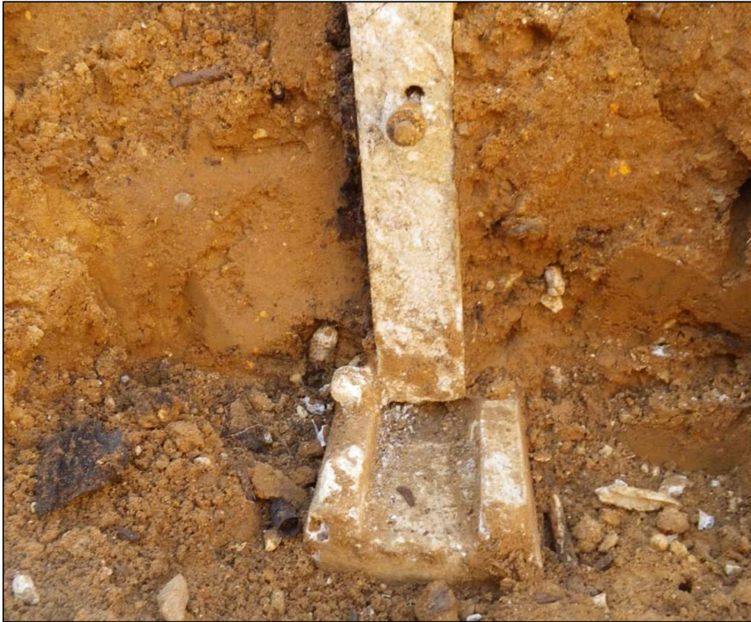
Plate 3. Shallow trough at base of panel. One of the tie bolts is also visible. South-east wall, camera facing south-west (ref. HQK 88)
