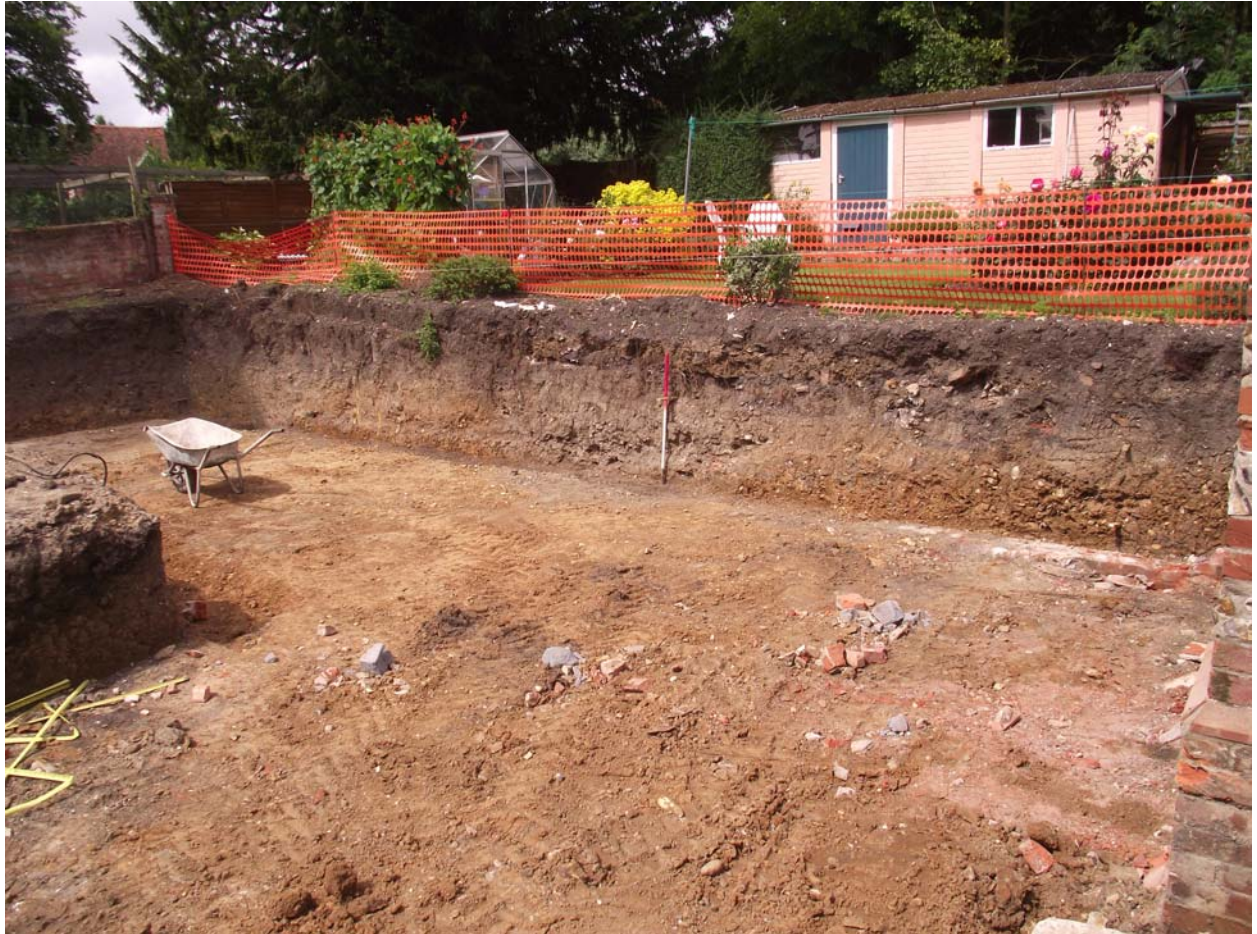
Plate 1. View of the excavated area looking north-west. The large pit 0005 can be seen in section behind the 1m ranging rod. Pit 0008 is in the north-west corner of the area (behind the wheelbarrow)
