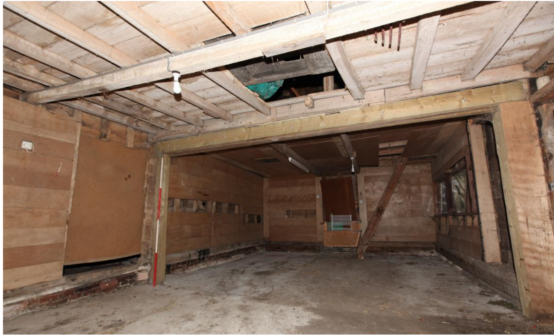
Illus. 11. The undivided ground-floor of the southern range from the south, showing the wall framing largely hidden by late-20 th century boarding. The ceiling of the former stable (3) in the foreground was renewed in the 20 th century, although one binding joist may be original. The door to the left opens onto the lean-to shed (4) which may have served as a tack room. The partition between the stable and the southern bay of the barn (2) has been removed and its position is indicated by the scale rod and corresponding new softwood in the ceiling.
