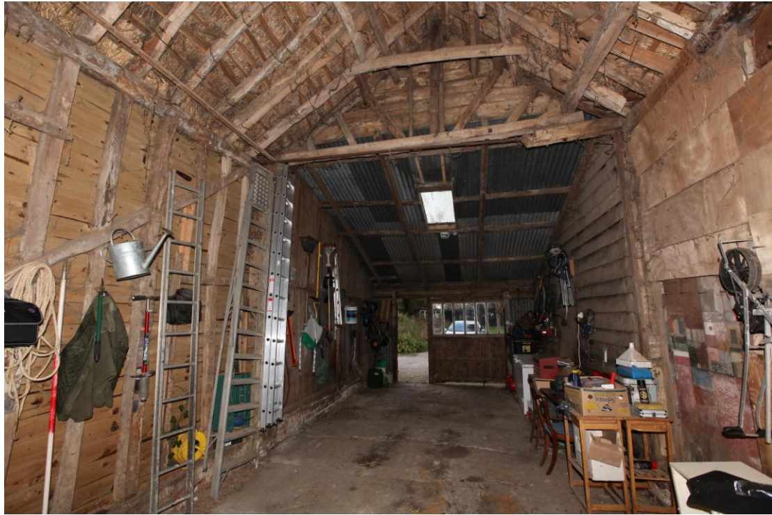
Illus. 9. The porch (1) from the west showing its junction with the 20th century lean-to shed (5) which replaced the threshing barn into which the porch initially opened. A short surviving section of the demolished barn's roof-plate is visible at top right (it continues into the remaining southern bay from which the lean-to is divided by a later boarded partition).
