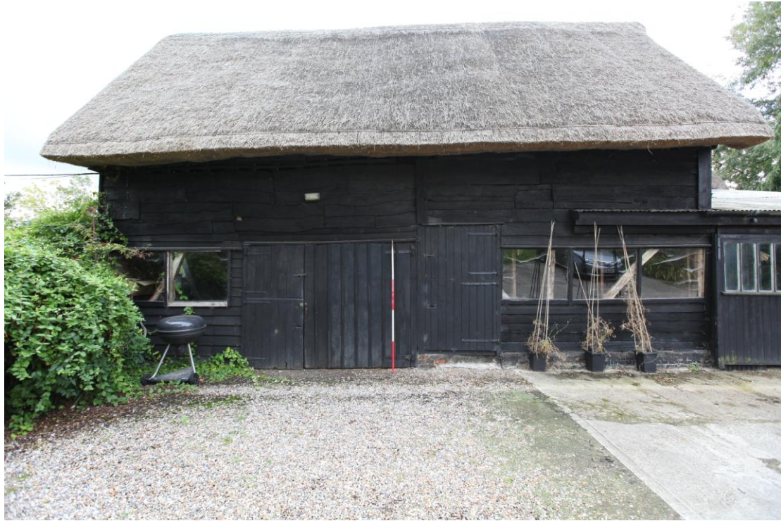
Illus. 5. The eastern exterior of the southern range, which consists of the southern bay of a late-18 th or early-19 th century threshing barn to the right of the scale rod (2) and an early-19 th century former stable (3) to its left. The various ground-floor doors and windows were inserted during the 20 th century but good, heavily tarred and waney-edged weatherboarding survives above.
