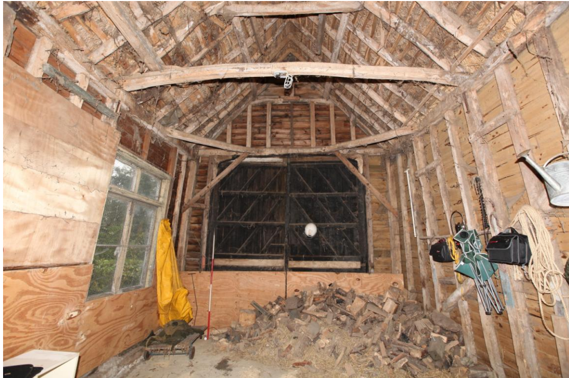
Illus. 7. The interior from the east of the 19th century porch (1). The wall framing is largely original, although cut by modern windows to the left and partly hidden by boarding. The barn doors are good late-19 th century half-hung examples with original bolted knee-braces framing the doorway.
