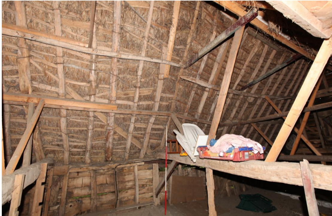
Illus. 13. The eastern roof structure of the southern bay of the original threshing barn (2) showing the tie-beam containing the empty pegged mortises of its original southern gable to the right – with the roof of the later stable (3) beyond. The studs of the barn are pegged to the roof plate while those of the stable are not. The clasped-purlin roof is partly original but its collars have been removed and the various struts are modern.
