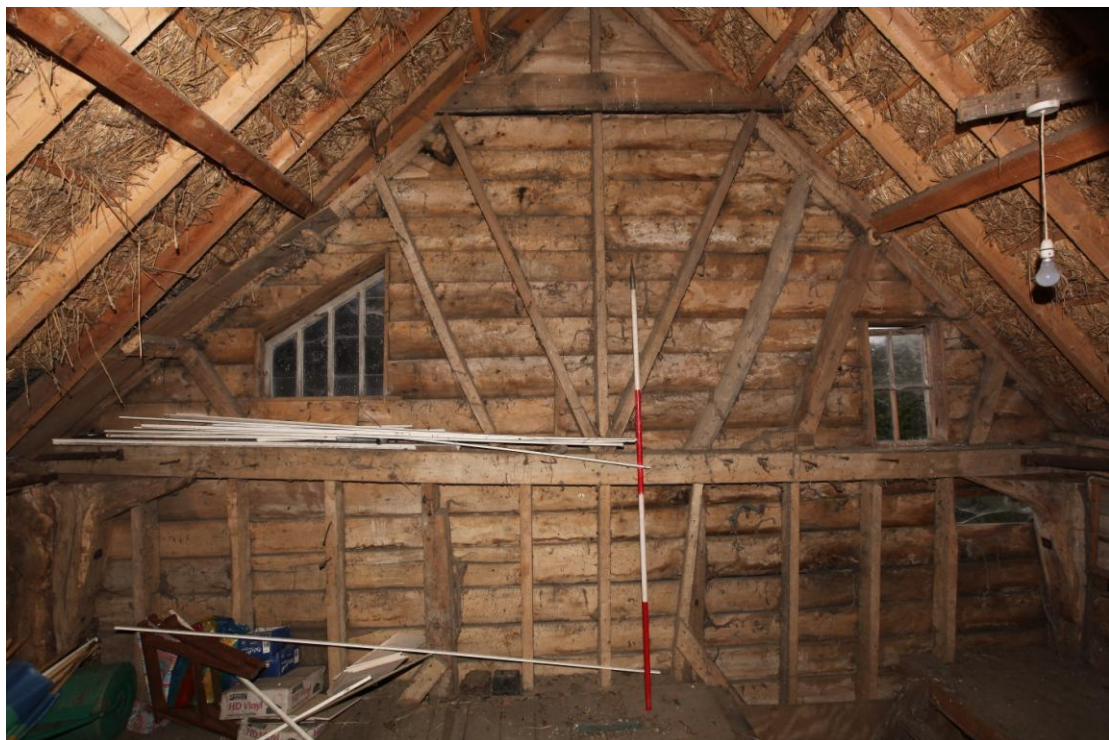
Illus. 12. The internal northern gable of the southern bay of the original barn (2) showing the later partition dividing it from the site of the demolished threshing floor. The tie-beam has been renewed but the bolted knee-braces of the formerly open truss (to right and left) appear to remain in situ . The floor is a 20 th century insertion.
