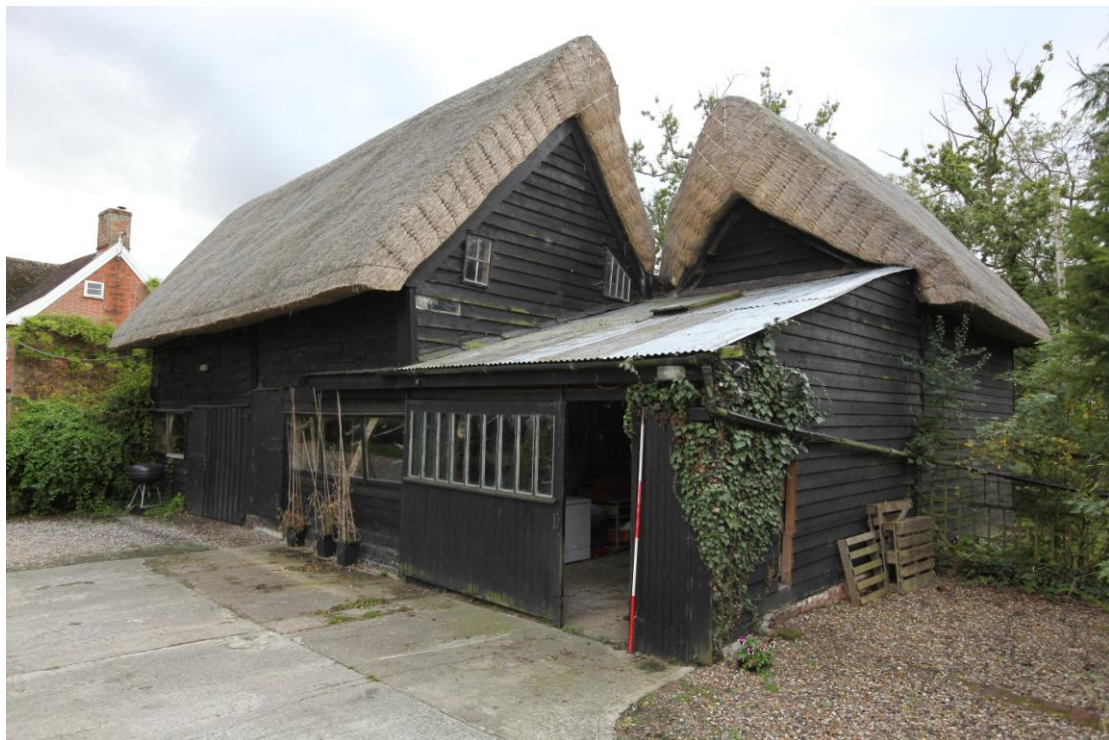
Illus. 6. The unusual appearance of the building from the north-east. A mid-20 th century lean-to shed with a corrugated iron roof (5) occupies the site of the demolished threshing bay of the original barn, with the surviving early-19 th century porch (1) to the right and the barn's southern end-bay (2) and the former stable (3) to the left.
