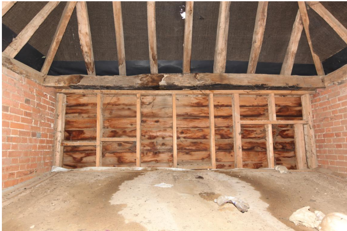
Illus. 13. The tie-beam of the hipped porch gable (above the modern fibre-board ceiling) showing a central mortise for a door bar with double-pegged mortises at both ends for the missing jambs of full-height original doors. The softwood studwork and weatherboarding are insertions of the late-20 th century. The barn evidently contained full-height doors at both ends of its threshing floor: a rare feature in an 18 th century barn.
