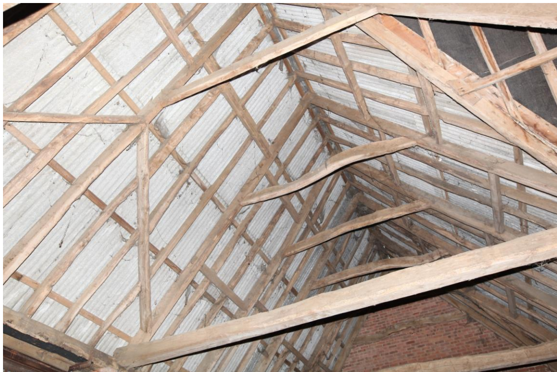
Illus. 8. The completely intact original roof structure containing two tiers of staggered butt-purlins with pegged through-tenons, pegged collars, and asymmetrical primary rafter braces (seen from the north). The rafter braces above the eastern entrance to the left reflect the lap boards of the western porch to the right but are lower in pitch and do not indicate the former presence of an eastern porch.
