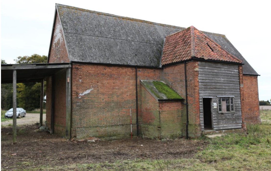
Illus. 2. The barn from the north-west showing the original hipped porch, now pantiled, with an integral lean-to shed in the return angle. The weatherboarded studwork is a late-20 th century insertion which replaced original doors (the barn possessed opposing full height doors from the outset). A blocked pitching hole is visible in the northern roof gable, and the roof scar of a demolished single-storied shed shown on 19 th century maps can be seen to the left.
