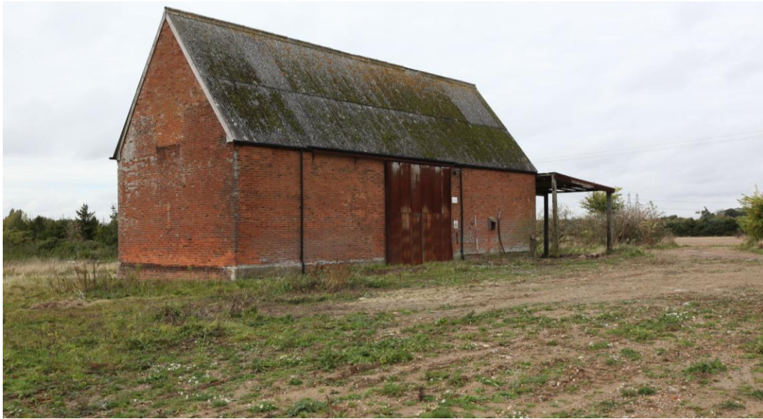
Illus. 1. The barn from the south-east showing its isolated location in open countryside. The steep pitch of the roof suggests the present corrugated asbestos replaced thatch. The apex of the southern gable was rebuilt in the 20 th century but the outline of a large pitching hole is still visible in the roof gable with a blocked ventilation loop beneath. 20 th century sliding doors of corrugated iron occupy the position of the original central entrance.
