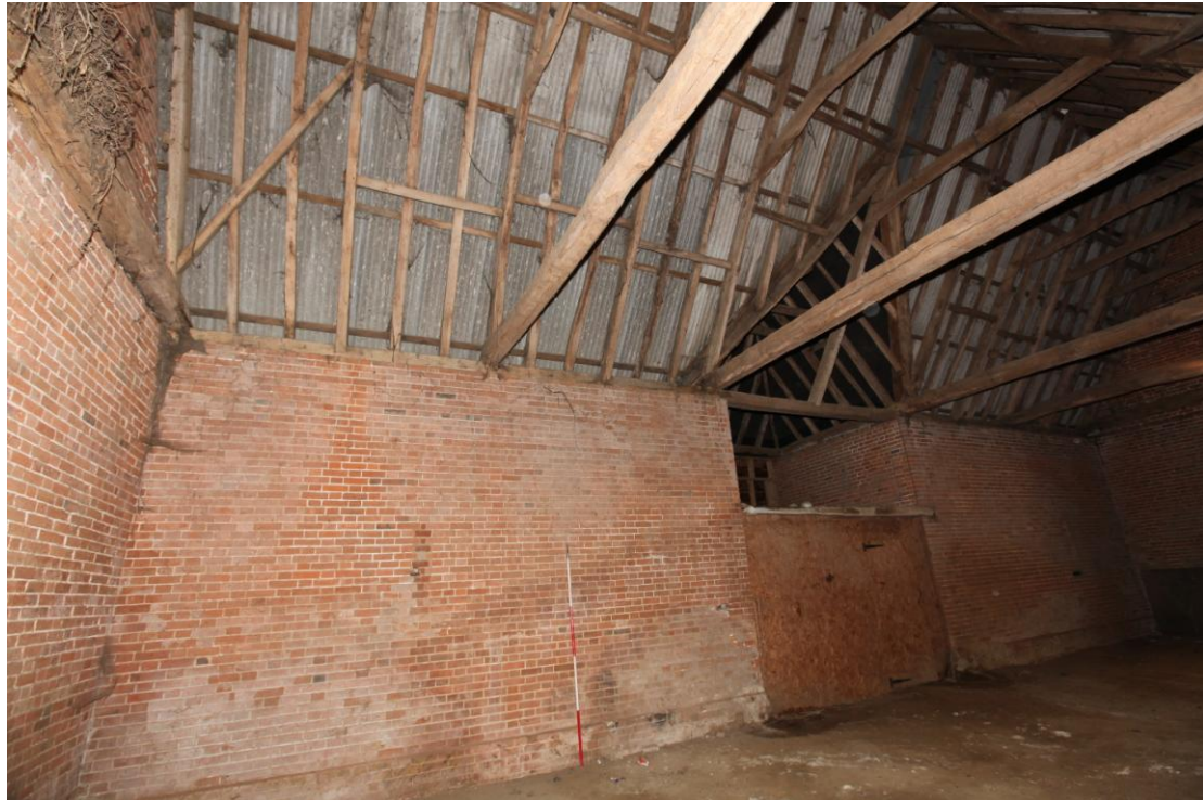
Illus. 9. The western internal elevation showing the central porch with a primary rafter brace to the southern gable to the left but not to the northern gable. The situation is reversed to the east. Two short ‘purlins’ were tenoned to the external face of each gable rafter to penetrate the brickwork and secure barge-boards. The blocked ventilation loops of the outer bays are not central (unlike those to the east) as they accommodated the lean-to sheds flanking the porch.
