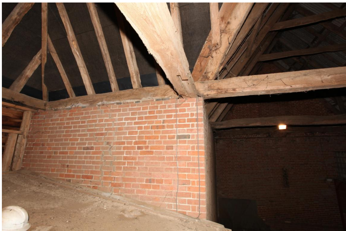
Illus. 14. The northern side-elevation of the porch showing the tie-beam of the main barn continuing to form its roof plate; this oak timber is an impressive 9.9 m (32.5 ft) in length, as is its counterpart to the south.
