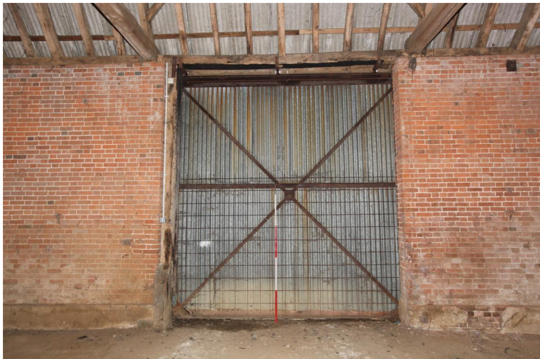
Illus. 12. The central entrance of the eastern elevation showing an ostensibly original door jamb to the left. The roof-plate contains a pegged mortise for a second jamb to the right with a central mortise to hold the door bar of the original full-height barn doors. The remaining jamb bears an incised date '1762' at a height of 1.75 m but this appears to be a relatively modern misreading of the original 1767 date on the opposite wall.
