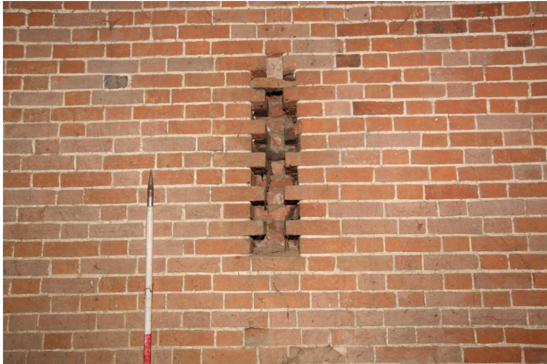
Illus. 11. The blocked ventilation loop to the internal northern gable showing its original indented brickwork. The barn contains six identical loops (in both gables and to both sides of the eastern entrance and western porch).
