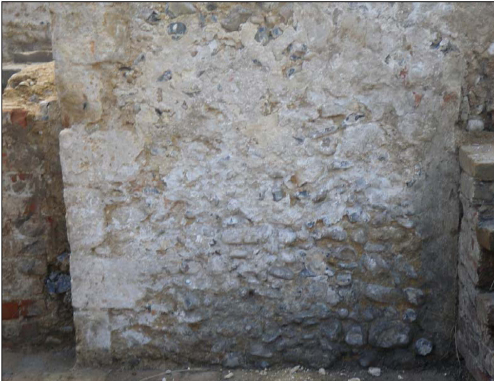
Plate 4. West wall 0116 detail. Looking west, the flint work is not in courses, unlike the eastern wall, and the block-work on the left of the picture is misaligned with the right angled corridor wall behind suggesting that they were not built at the same time. The chamfered finish to the wall on the right of the picture is a repair to the scar left when the returning cross wall 0115 of the cellar was removed.
