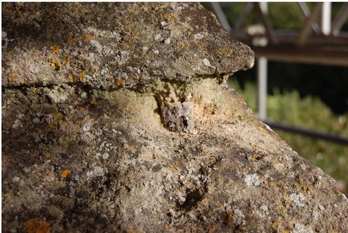
Plate 11. An example of the iron staples/dogs set into the limestone tying the buttress capping stones together.
