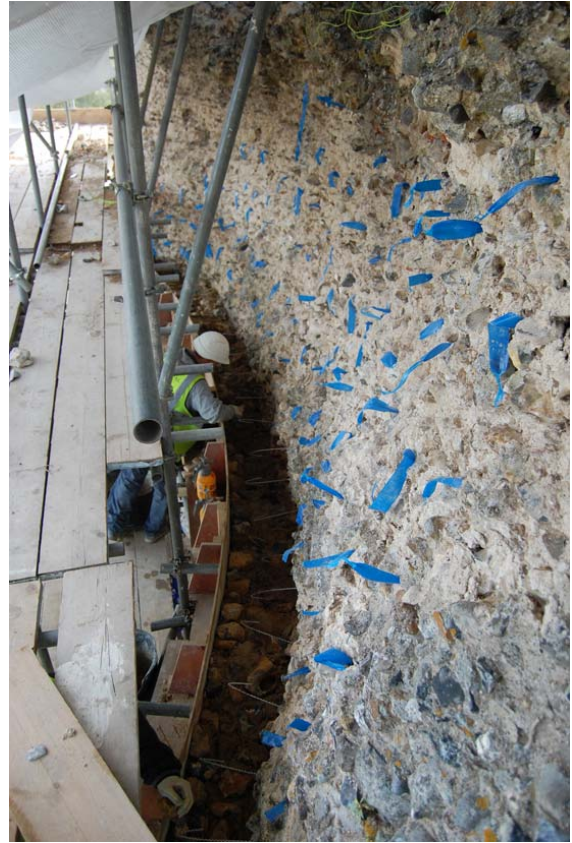
Plate 4. Building up the inner face of the wall behind curving timber formwork. The blue tags mark the stainless steel pins that help tie the flint face to the core
