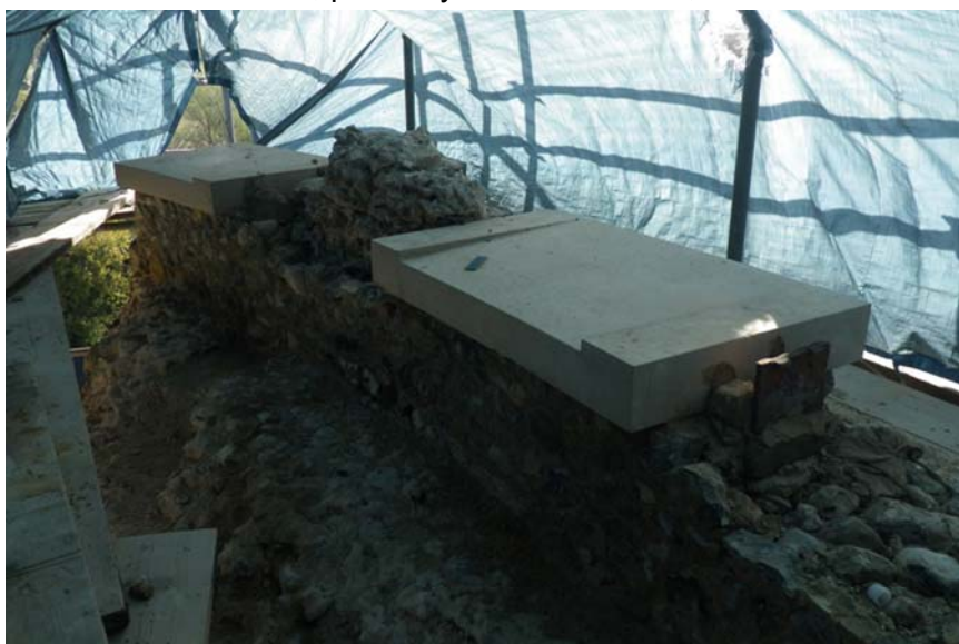
Plate 8. Limestone sills placed between the merlins as part of the reconstruction of the crenulations
