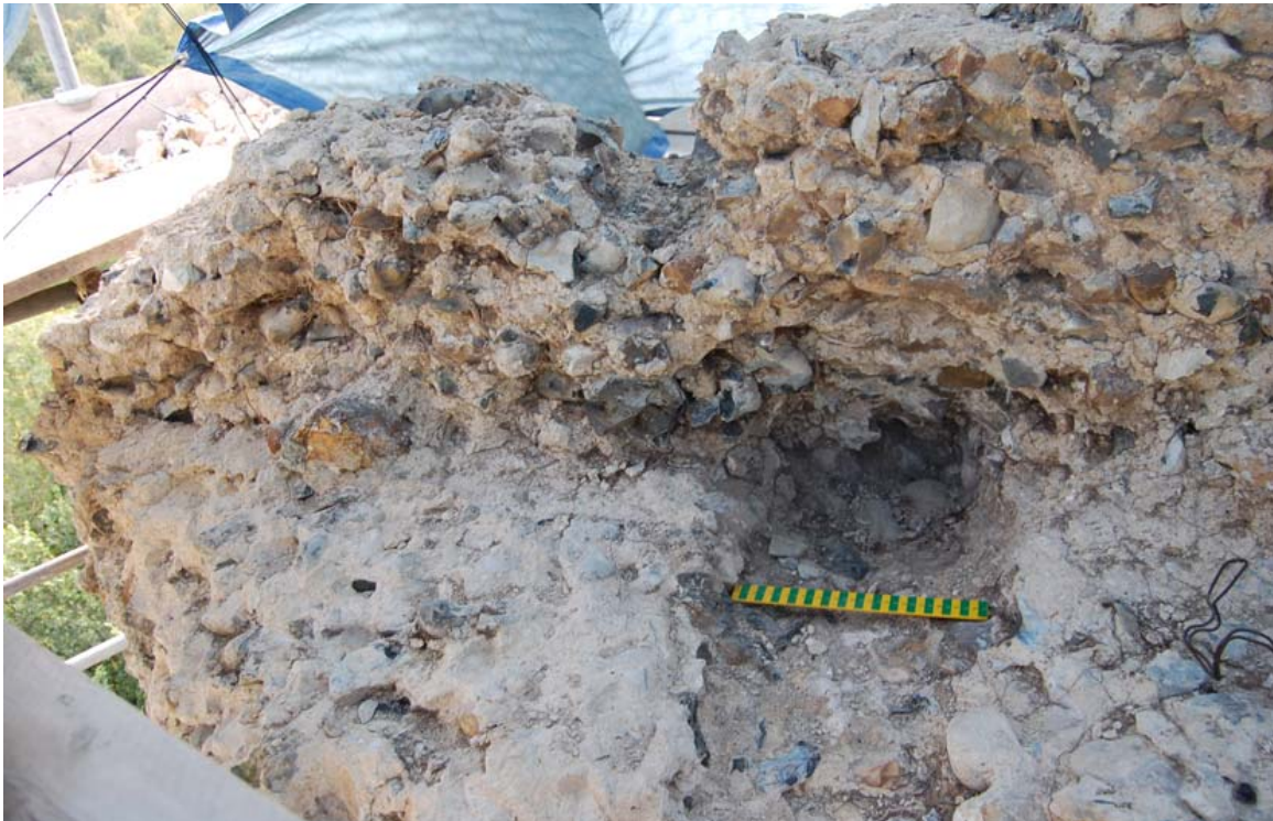
Plate 5. The scale lies within one of the beam slots set into the top of the wall to support the roof timbers of the keep buildings. The remains of the smaller hole which can be seen above it to the left, is thought to be for a water spout to discharge rain water through the parapet and outside the keep.
