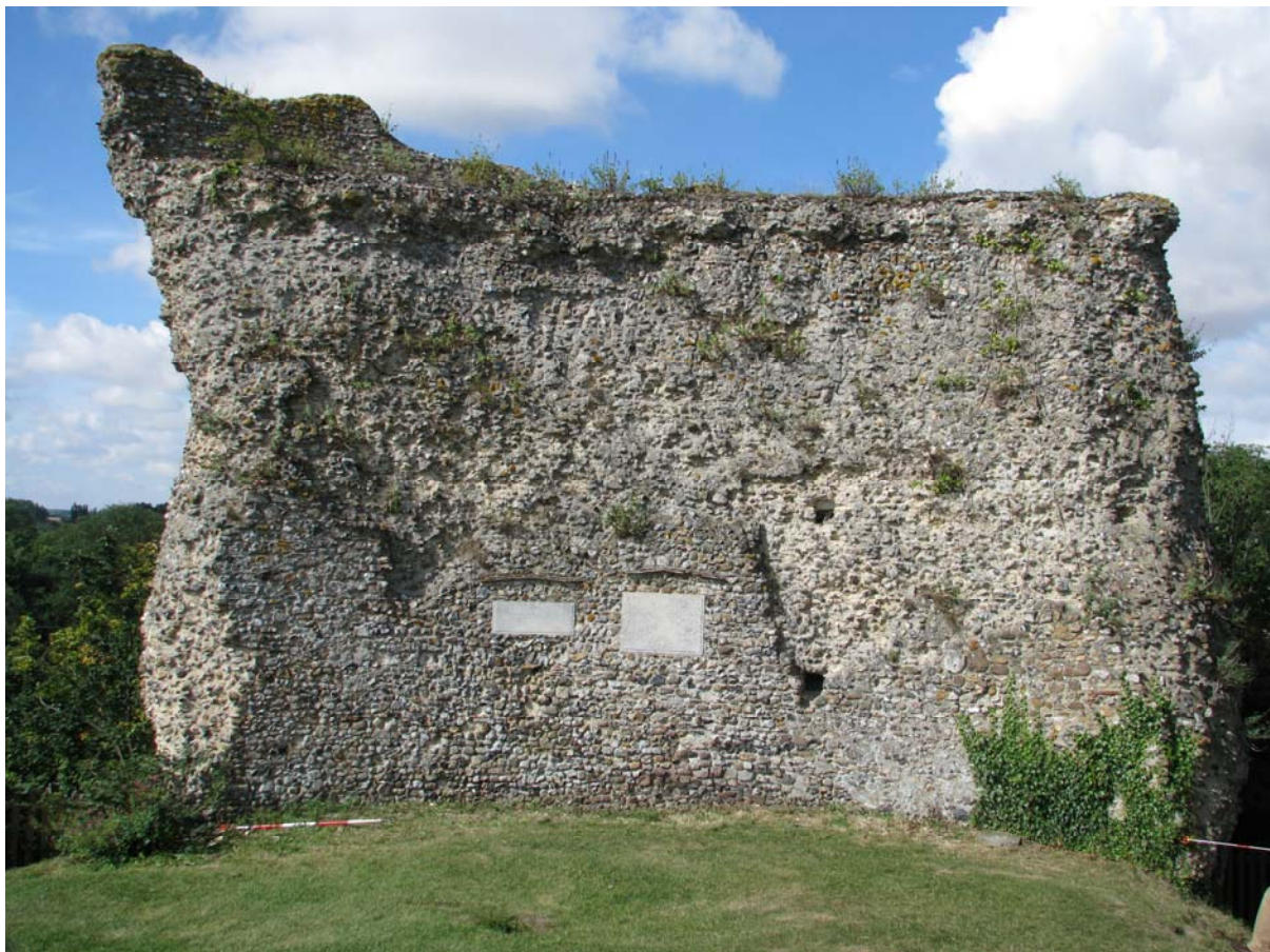
Plate 2. General view of the interior of the keep showing the condition of the monument prior to consolidation. The wall face has fallen away from a large section of the upper part of the wall exposing the wall's core. The remains of the parapet can be seen at the top of the wall to the left.
