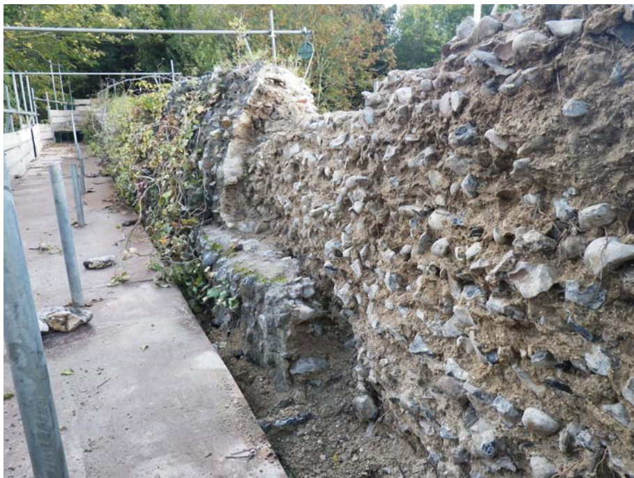
Plate 14. Top of the bailey wall with concrete capping partially removed revealing the original wall core fabric beneath. North face of the wall looking east.
