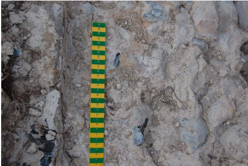
Plate 6. Looking down on the top of the keep wall showing the mortared screed finish and the face of the parapet wall to the left of the scale.
