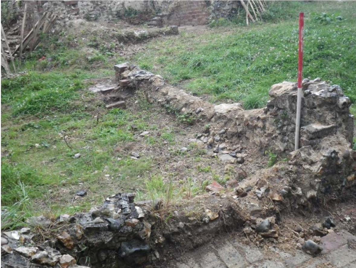
Plate 17. An example of the condition of the 19th century walls inside Kerrison's Folly prior to repairs
