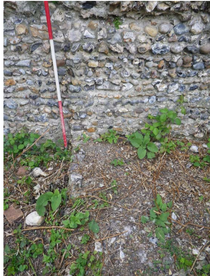
Plate 10. Interior of the north wall of chambers 1 and 2. The scale is positioned against the west face of the central sub wall. The unbroken flint work to the right of the scale demonstrates that the stub wall did not rise above floor level.
