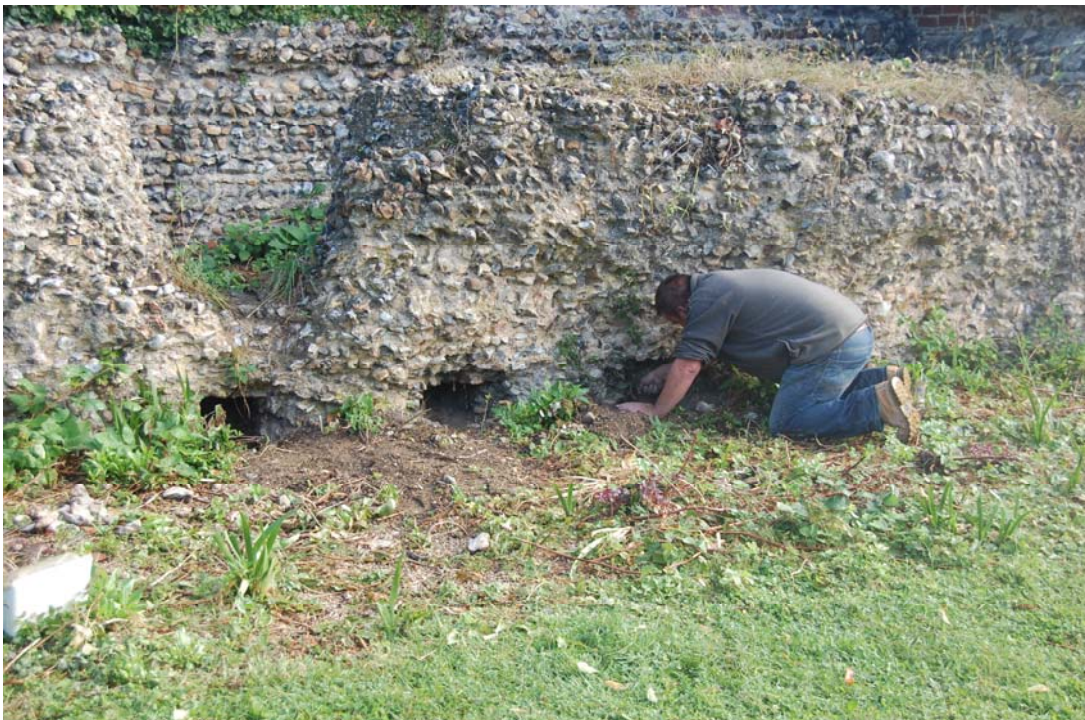
Plate 2. Excavating the channel entrances (Nos 7, 8 and 9) at the base south wall of chambers 1 and 2, showing the arrangement of channels in groups of three
