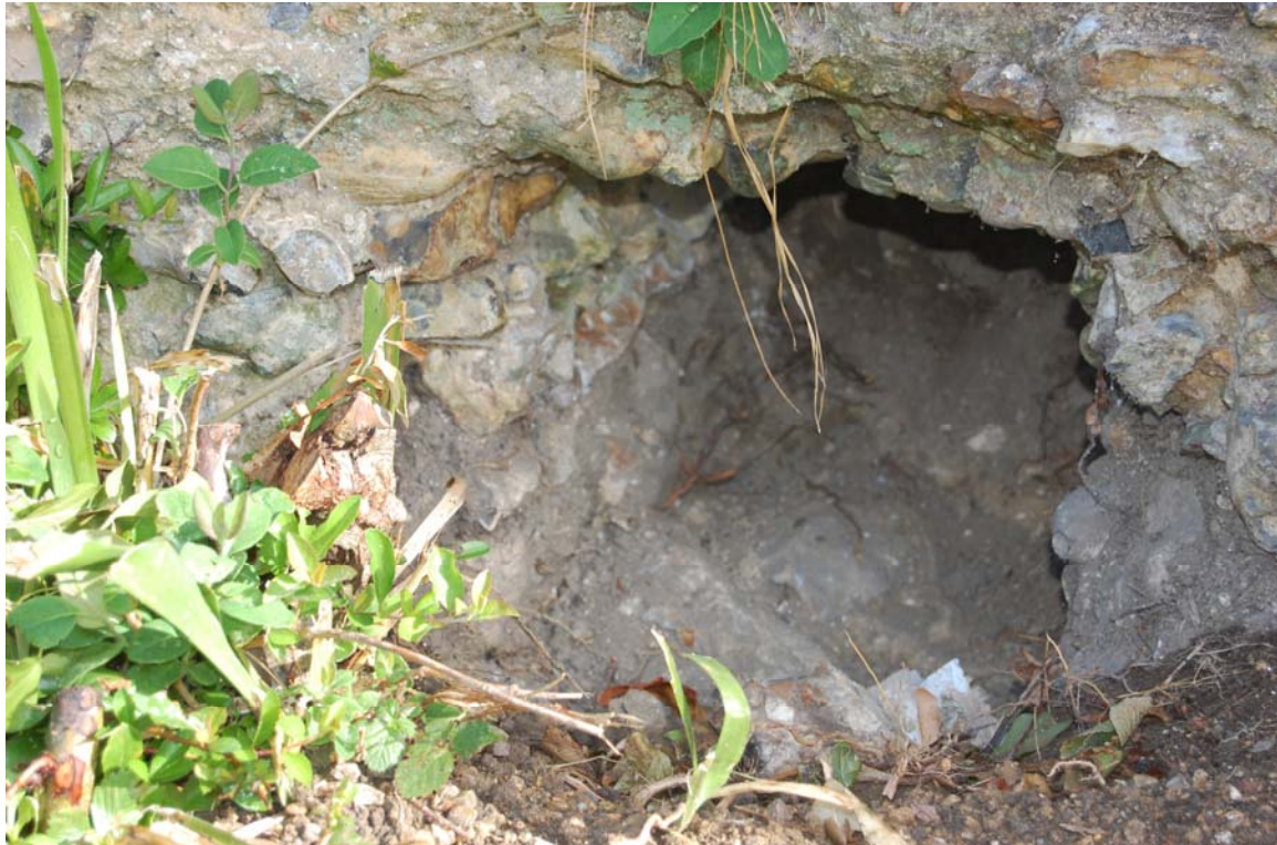
Plate 3. Entrance to one of the channels which are square-section and measured 300mm across. The internal faces were neatly finished suggesting that they had been constructed around timber beams. The floor of the channels was mortared flint and the voids had become blocked with soil which was partially excavated prior to blocking with 'masonry'.
