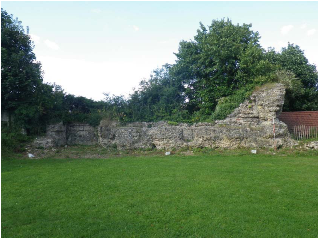
Plate 1. The bailey curtain wall from within the bailey looking south. The open structure on the left is the remains of the west tower, the south wall of which has been truncated at ground level. The tall section on the right is a partition wall between chambers 2 and 3. The entrances to the series of channels below floor level can be seen at the base of the south (nearest) wall.
