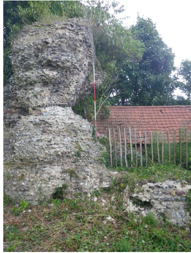
Plate 6. The partition wall between chambers 2 and 3 looking N. The ranging pole is on the line of the original wall face, as demonstrated by fragments of surviving Norman facework at the top and bottom of the wall, and illustrates the degree of fabric loss in the middle of the wall.
