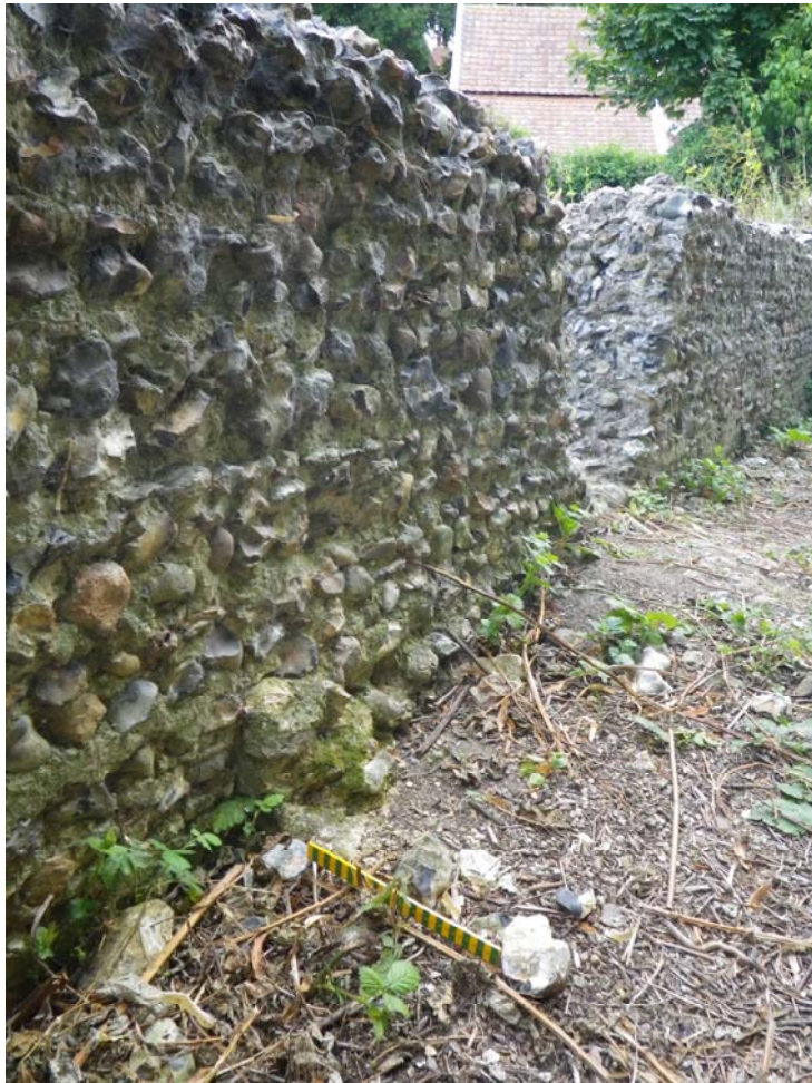
Plate 9. Interior of the south wall of chambers 1 and 2. The two chambers are separated by a central stub wall, which is buried below existing ground level there is no scarring on the vertical wall faces to indicate that the stub wall extended above its extant height which suggests that was not a partition but a support for a suspended floor and chambers 1 and 2 were not divided above floor level.
