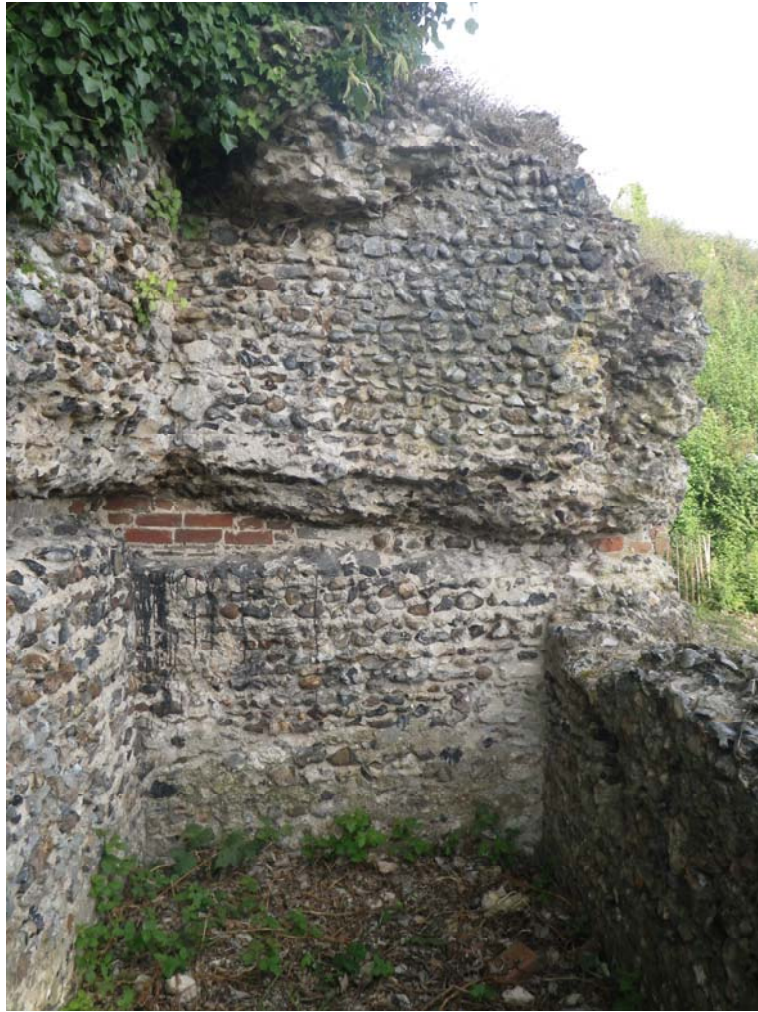
Plate 5. West face of the N-S partition wall between chambers 2 and 3. A horizontal channel, repaired previously with brick, divides the wall at mid-height and can be seen returning on the north wall at the left of the picture. Horizontal flint coursing characteristic of Norman masons can be seen on the lower wall and appears angled on the upper suggesting that the upper block has slumped and was once detached. The N-S channel is directly over channel No.10 below the ground floor level.
