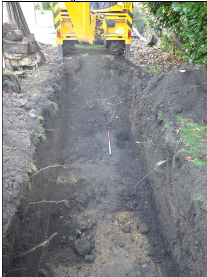
Plate 2. Facing north, ditch 0001 is visible to the right of the trench. Scale is 1m.
