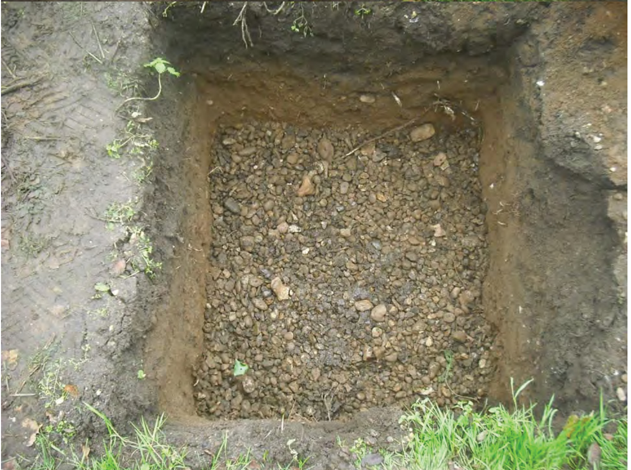
Plate 25. A barrowful of stones from the sieving is backfilled into the base of TP 5
