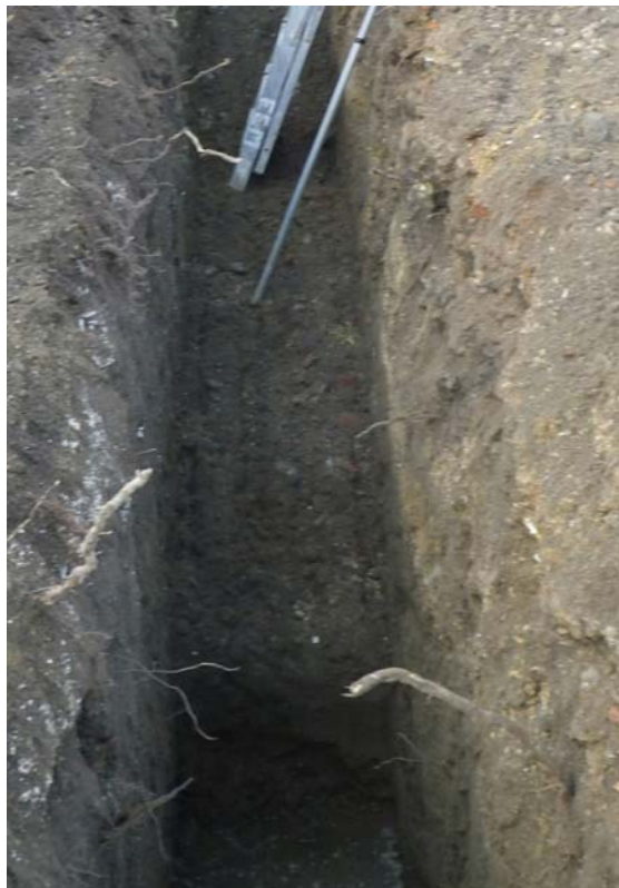
Plate 6. South wall footing trench at 1.6m with a possible medieval quarry pit 0014 at 2.2m and partially under water in the foreground facing north.
