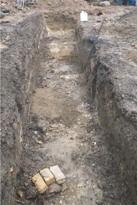
Plate 1. Evaluation trench to the top of the clay, 0004. Intercutting later post medieval features and a modern drain in the foreground facing south
