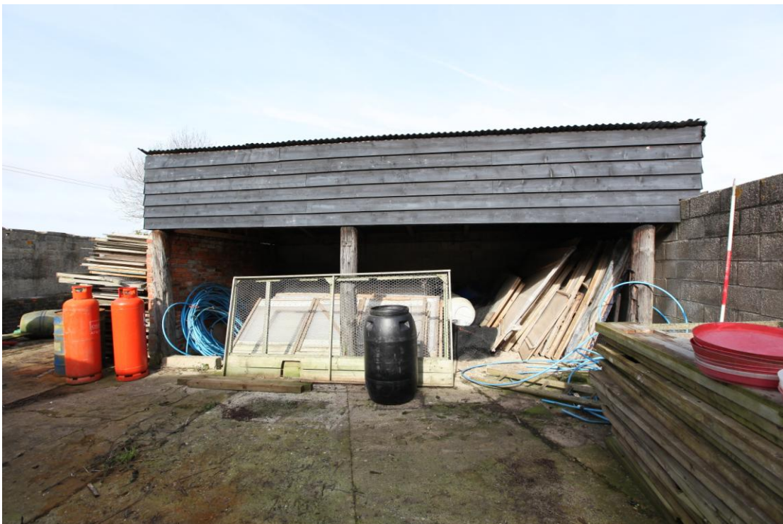
Illus. 4. The southern exterior of the open-sided shelter-shed (3) to the rear (north) of the barn (1). This is shown on the historic Ordnance Surveys but with the exception of its western brick wall (left) was entirely rebuilt in the mid-20th century with re-used telegraph poles and cement block-work.
