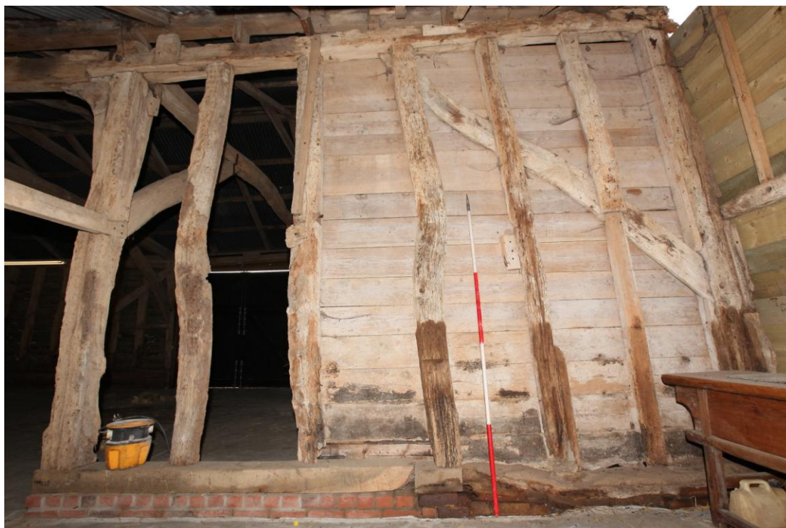
Illus. 14. The northern exterior of the western bay from the later lean-to, showing the intact original studs with an ogee-curved internal wall brace reflecting that of illus 11. The internal boarding is a 19 th century addition, and the studs were formerly infilled with wattle-and-daub and rendered externally.
