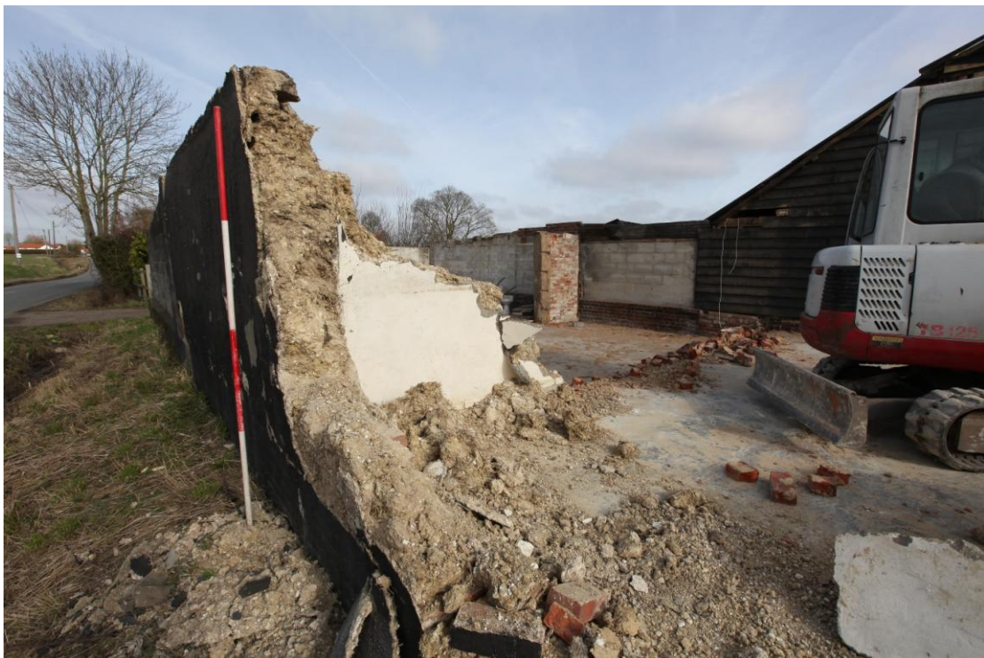
Illus. 2. A detail from the south of the partly demolished tarred western wall of the shuttered clay shed (2a) adjoining the barn's western gable. There is no trace of clay lump blocks within the fabric.
