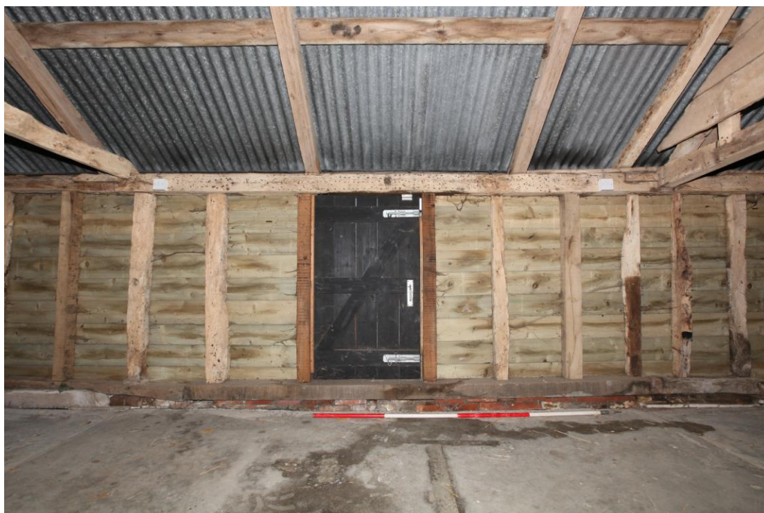
Illus. 13. The central bay of the rear (northern) lean-to with a modern door slightly to the left of the original. The roof-plate appears to belong to a 16 th century structure, with edge-halved and bridled scarf joints beneath the tie-beams to left and right, but all but one or two studs have been replaced and the original lean-to was probably widened in the 19 th century.
