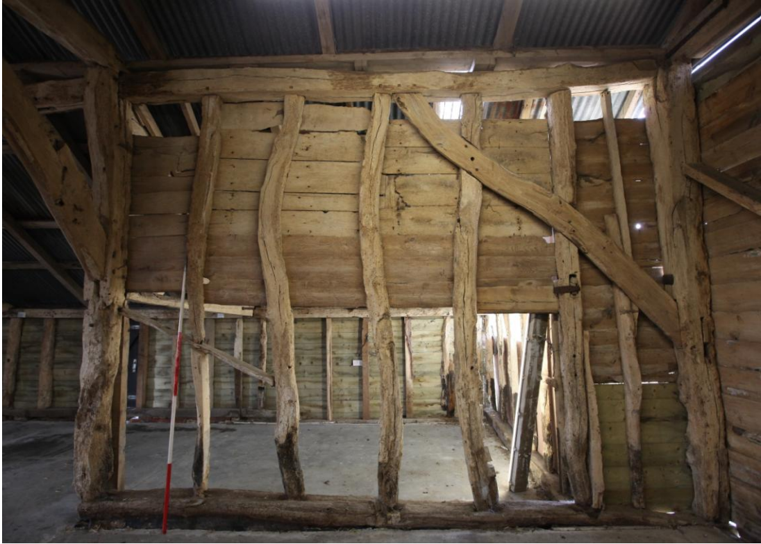
Illus. 11. The northern interior of the eastern bay showing an original ogee-curved internal brace with a mortise in the corner post for a matching brace in the rebuilt gable. Note the unusually distorted nature of the oak studs.
