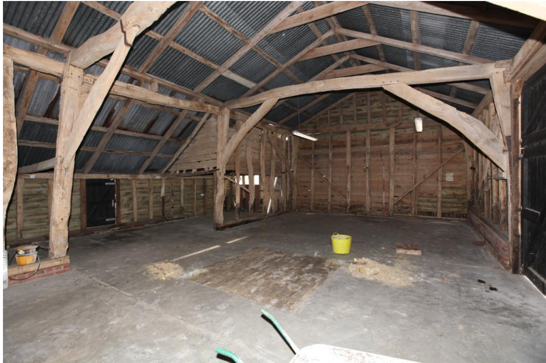
Illus. 9. The interior from the south-west showing the later rear lean-to on the left and the modern concrete floor with a central panel made from gault bricks that are understood to have been salvaged from the remains of a threshing floor.
