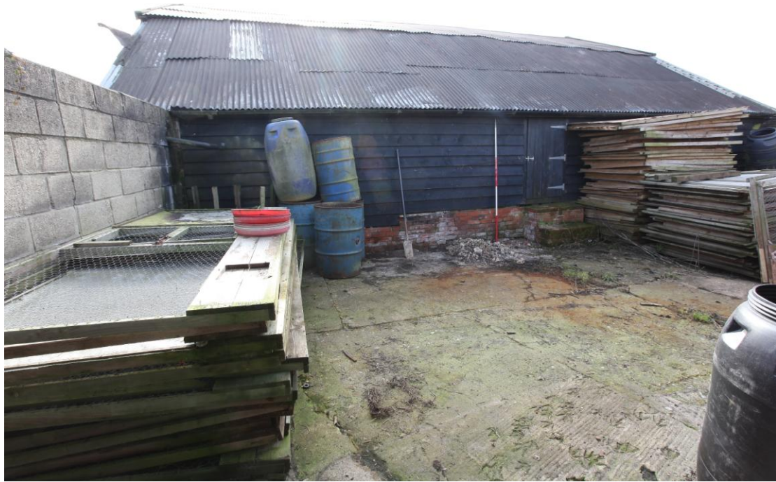
Illus. 5. The rear (northern) exterior of the barn (1) from the enclosed yard (4) showing the corrugated iron roof and recent weatherboarding of the later rear lean-to.
