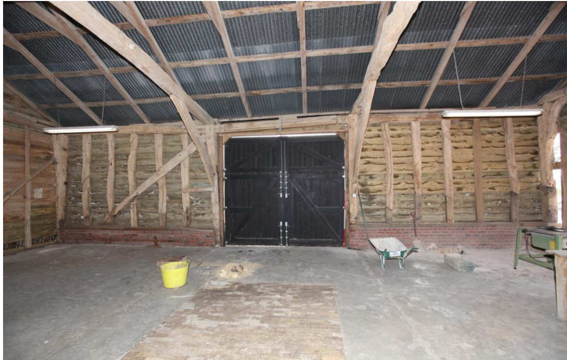
Illus. 7. The southern interior of the three-bay threshing barn (1) showing its central entrance doors flanked by original arch-braced tie-beams. The roof-plate contains mortises for the jambs of a slightly narrower original entrance. The studs of the outer bays have been truncated at their bases but with the exception of the penultimate stud on the right all are original and are trenched for missing internally trenched braces that reflected those of the northern wall. The diagonal brace on the left is secondary.
