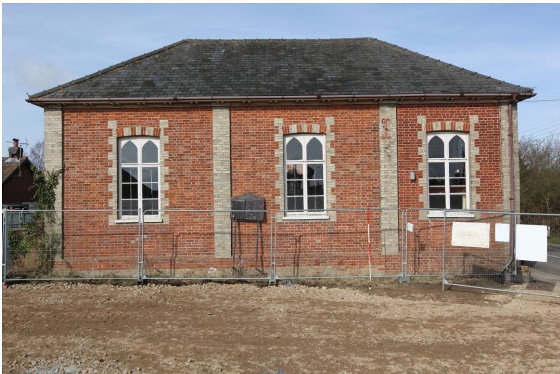
Illus. 2. The southern exterior showing the gault brick pilasters which separate the elevation into three bays. The right-hand bay is narrower and was added as an extension to the original two-bay chapel in the late-19 th century. Every attempt was made to match the earlier fabric, but the later brickwork is markedly darker and more uniform in colour.
