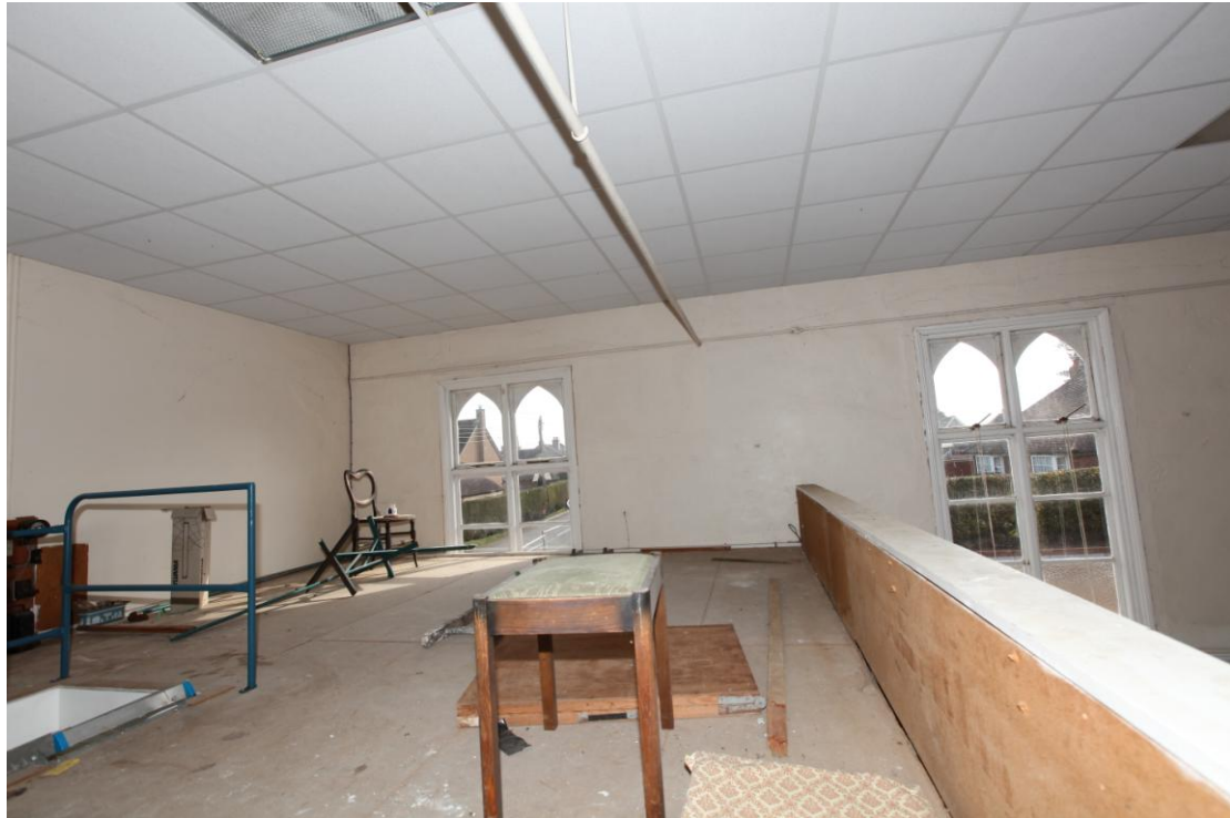
Illus. 11. The balcony above the modern partitions at the eastern end of the hall (1), viewed from the north. This area was reached by a retractable steel loft ladder from the entrance passage (as shown to the left). Note the iron tie-rod that replaced the original eastern gable when the building was extended.
