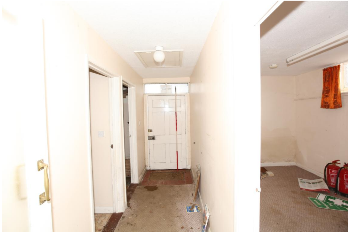
Illus. 13. The entrance passage (5) from the west, showing the external door with the loft hatch to the balcony in the ceiling above, the ‘committee room’ (6) on the right and doors to the kitchen, WC and cloakroom (2, 3 & 4) on the left.
