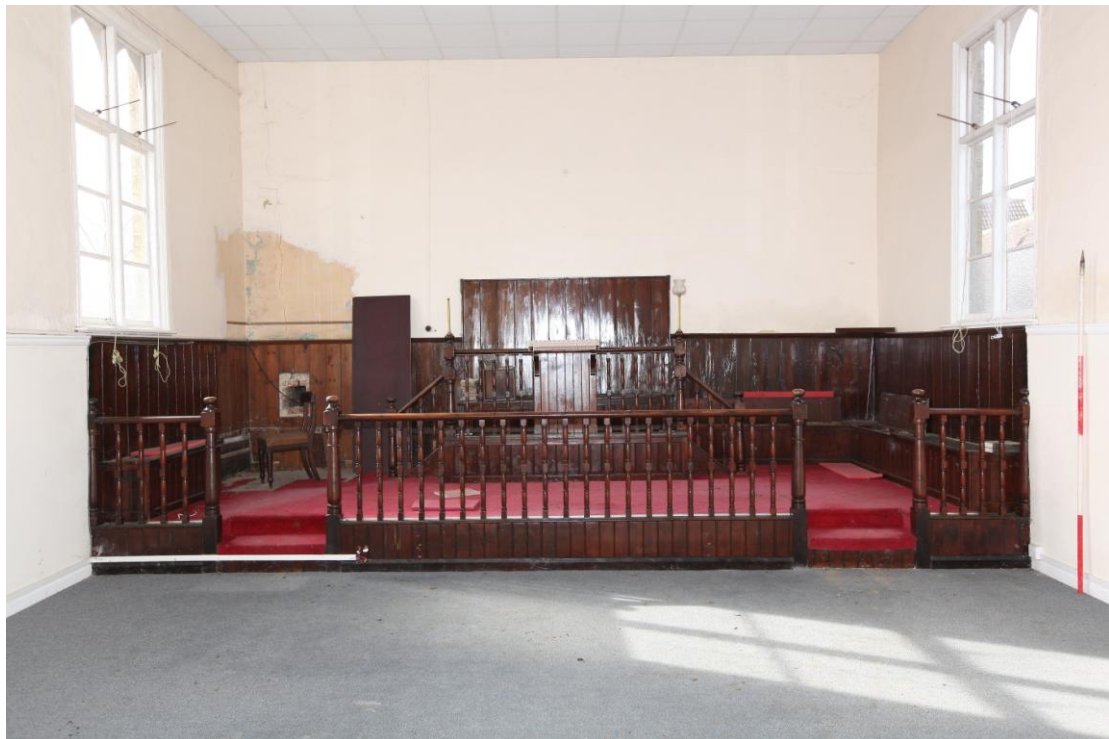
Illus. 6. The stained pine dais (1a) at the western end of the main hall (1). This is probably contemporary with the extension of the chapel at the end of the 19 th century.
