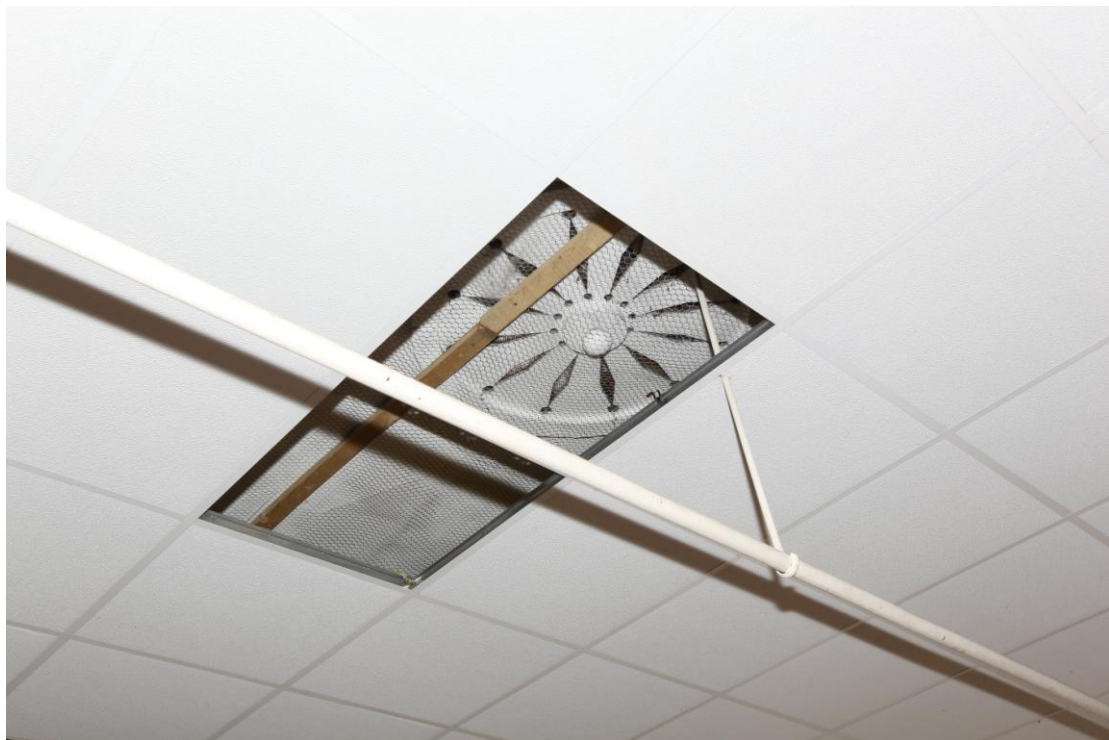
Illus. 12. A detail of the ventilation rose or chandelier support visible beneath the 20th century ceiling tiles above the eastern balcony, with the tie-rod shown in illus. 11. Other Victorian decorative features may be hidden behind modern cladding elsewhere.
