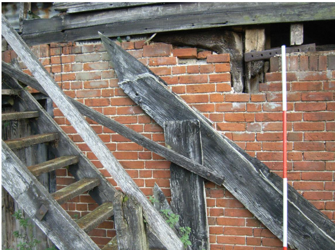
Illus. 14. The western gable of the granary (5) showing the timber post and knee-brace of an earlier timber granary and cart shed embedded in the later brickwork.
