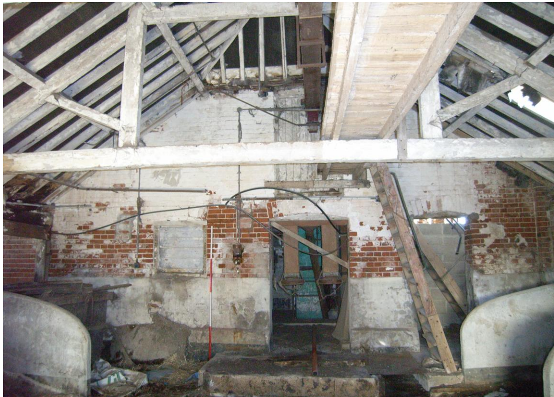
Illus. 10. The southern exterior of the eastern former stable (1c) from the later milking parlour (2a) showing its original central door flanked by windows and a later loading door to the hay loft above.
