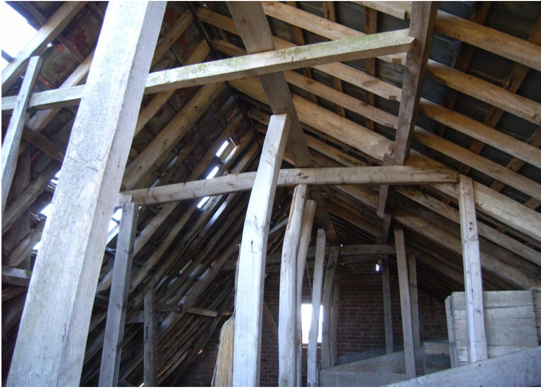
Illus. 15. The grain floor of the granary (5) from the western gable entrance showing the remains of 19 th century grain bins and the difference between the northern side of the roof (left) which contains butt-purlins and appears to survive from an early-19 th century predecessor, and the shallow-pitched southern half which spans the lean-to sheds and relates to its mid-19 th century remodelling in brick.
