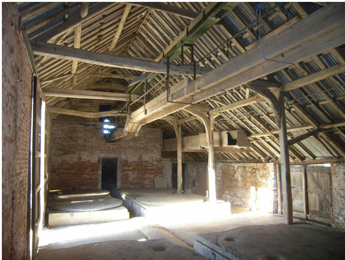
Illus. 4. The interior of the central threshing barn (1a) from the east showing its intact roof and rear aisle with the concrete bases of the 20 th century grain silos that were reached by the surviving axial platform. The doors to the western stable (1b) and its rear lean-to shed (1d) are secondary insertions. The relatively shallow pitch of the roof suggests it was initially pantiled to match the house.
