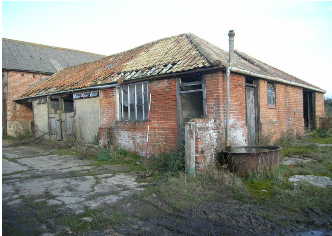
Illus. 11. The ‘double-pile’ mid-19 th century cattle shed complex (2) to the east of the yard (seen from the south-west). The wide entrance to the right-hand milking parlour (2a) is original and there is evidence of a similar wide doorway in the left-hand gable. An open-sided shelter-shed (2b & 2c) to the left has been enclosed to form loose boxes.
