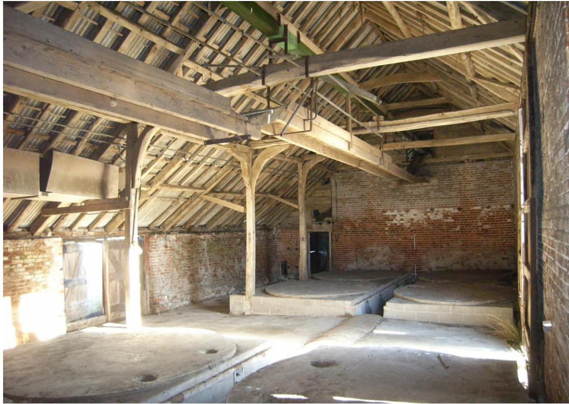
Illus. 5. The interior of the threshing barn (1a) from the west the showing intact roof and arcade posts with the rear doors of the (missing) threshing floor to the left.
