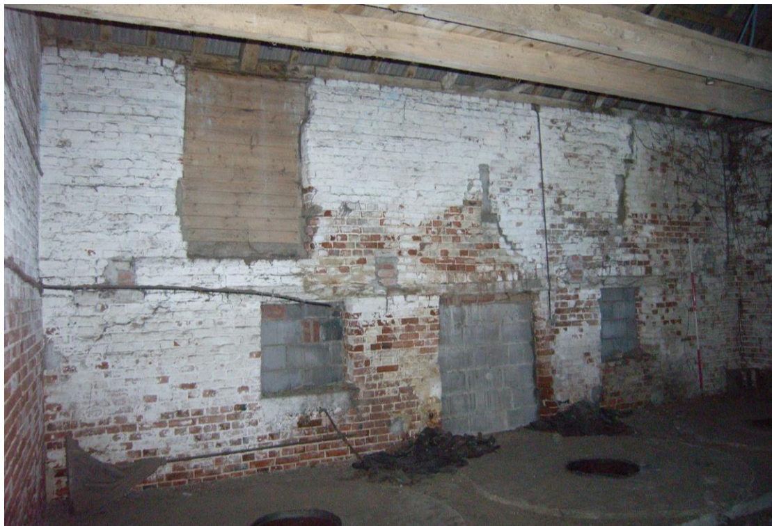
Illus. 8. The southern interior of the former stable (1b) to the west of the threshing barn (1a), showing its blocked central door flanked by windows, three ventilation loops to the missing hay loft (the easternmost enlarged to form an external door) and the scars of the removed principal ceiling joists.
