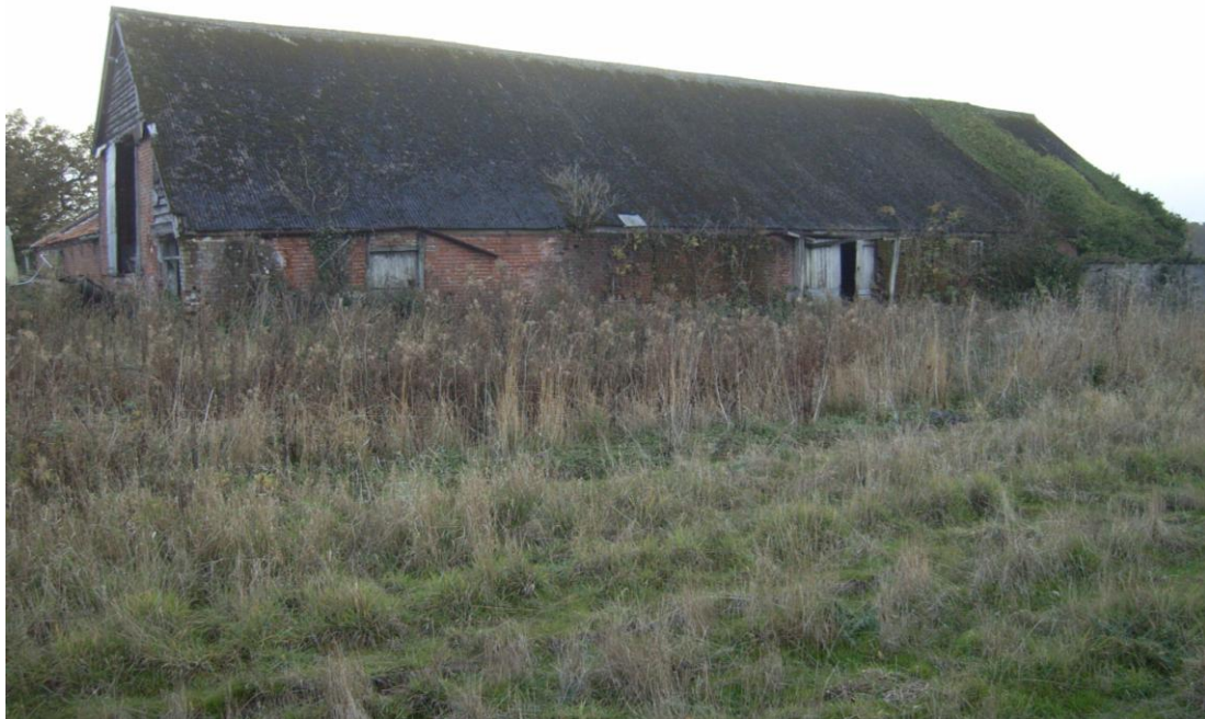
Illus. 3. The intact original rear aisle of the brick barn with 20 th century doors in its eastern gable, the original door to the lean-to shed adjoining the eastern stable (1e) to the left, and the rear doors of the threshing barn (1a) to the right.
