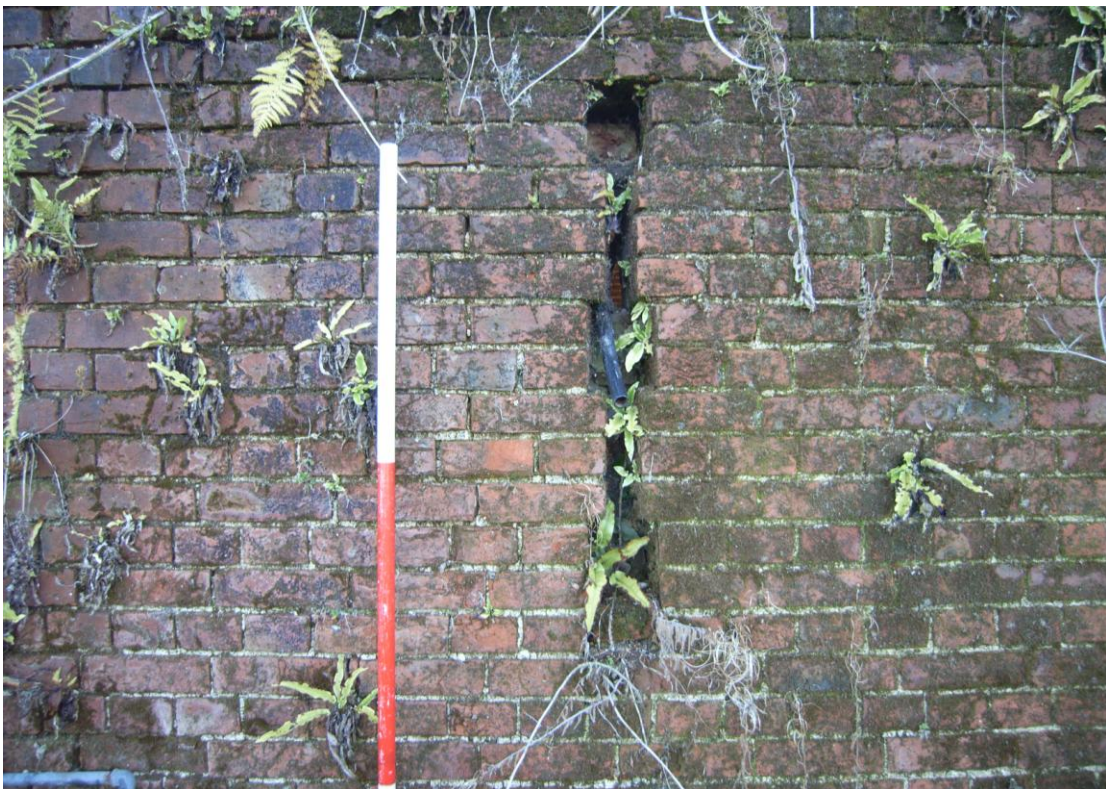
Illus. 16. Detail of a ventilation loop in the northern exterior of the threshing barn (1a).
