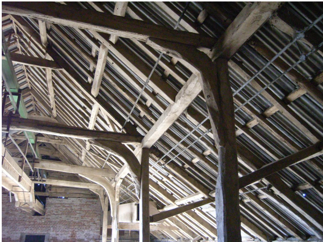
Illus. 6. The original roof structure from the east showing its impressive bolted knee-braces, raking aisle struts (tenoned to the arcade posts and the principal aisle rafters), staggered butt-purlins, pegged collars and ridge-piece.
