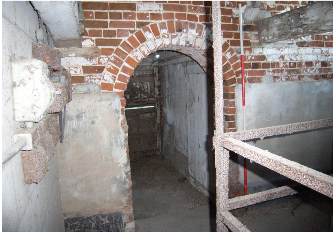
Illus. 9. The original arched doorway in the northern interior of the former stable (1c) to the east of the threshing barn (1a) with an original ceiling joist to the right. This door opens into the rear lean-to shed (1e) immediately opposite a central external door.
