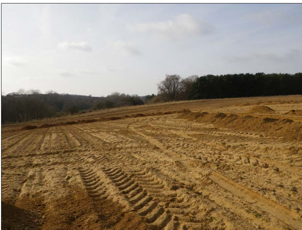
Plate 6. Looking west to show the southward slope into the river valley. Taken from the northern end of Trench 13
