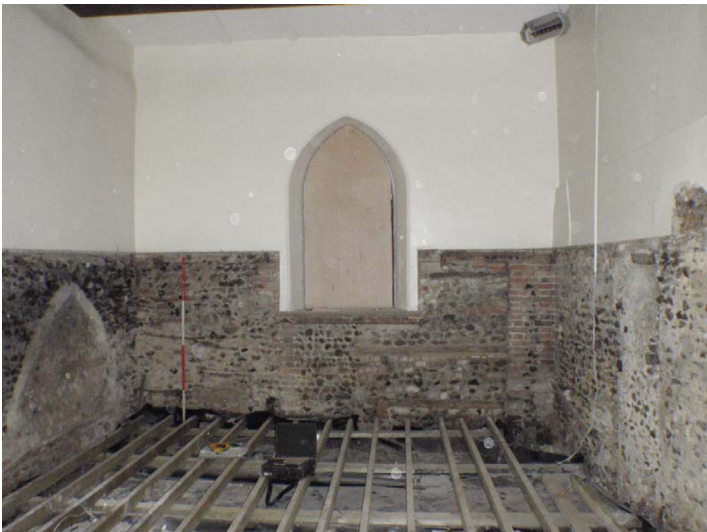
Plate 13. The exposed fabric of the north end of the cross-wing. The flints are mixed with reused bricks and timber over the entire area of the wall suggesting that it has been largely rebuilt.
