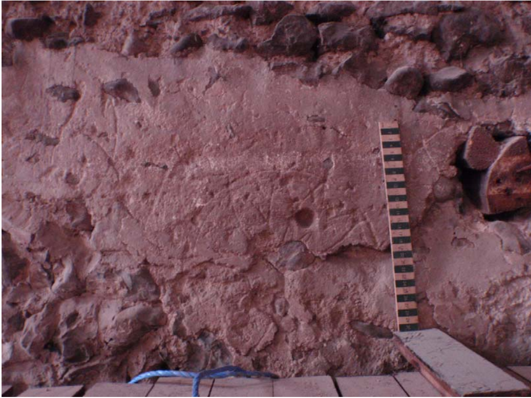
Plate 10. Apotropaic marks. Daisy wheel patterns were inscribed into the surface of the plaster on the north wall; these were numerous and occurred wherever the fragments of plaster survived (the remains of three wheels are shown here).
