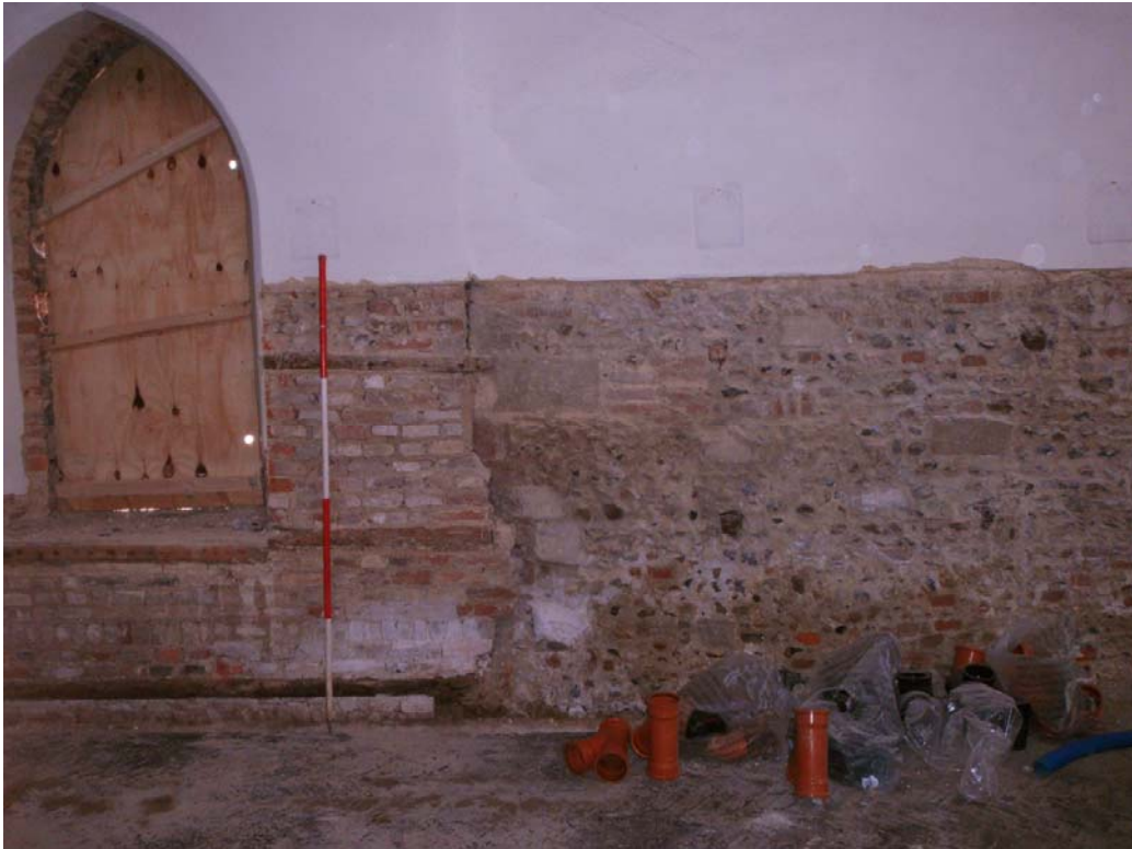
Plate 8. The inside of the church south wall after the removal of the wainscot. To the left the wall is made up of a jumble of reused brick roughly laid in a mix of stretcher/herringbone bonds as part of the C19th rebuild. Horizontal timbers contemporary with the brick and were built into the fabric to attach the wainscot. The 'rubble' wall to the right dates to the c.17th century and is part of the remedial work following the removal of the buttress and putative chimney from the outer face.
