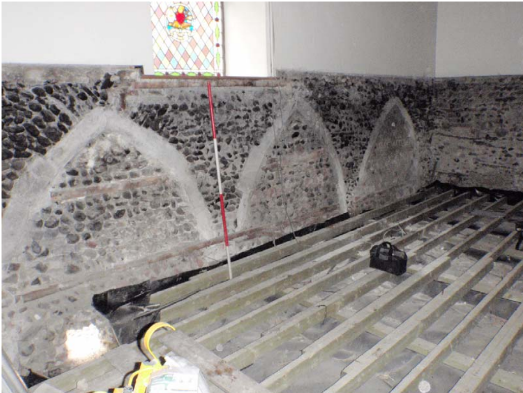
Plate 12. The interior of east wall of the cross-wing after the removal of the wainscot which revealed the arches of the reredorter. The reredorter was flushed through by water from the Stour brought to the building in a channel shown on the tithe map (Fig. 2 and Pl. 14). The arches came together at the current ground level but there was no opportunity to examine how the arches were supported below this. The presence of the horizontal timbers built into the arch infill suggests that they were not blocked in until the C19th.
