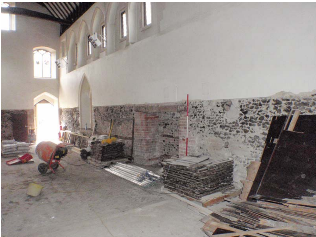
Plate 9. Interior of the north wall with the exposed remains of the brick-built jambs of the central door which was inserted in the 18th century; graffiti scratched into the bricks dated 1811. To the right of the door is the vestiges of wall plaster which carry apotropaic (evil averting) marks inscribed its surface. In-built horizontal timbers for the wainscot identify where the wall surface was re-built in the C19th; where the earlier wall face survives the wainscot was held on with inserted small wooden plugs. The blackened face of the flints is caused by sooting from the C19th heaters.
