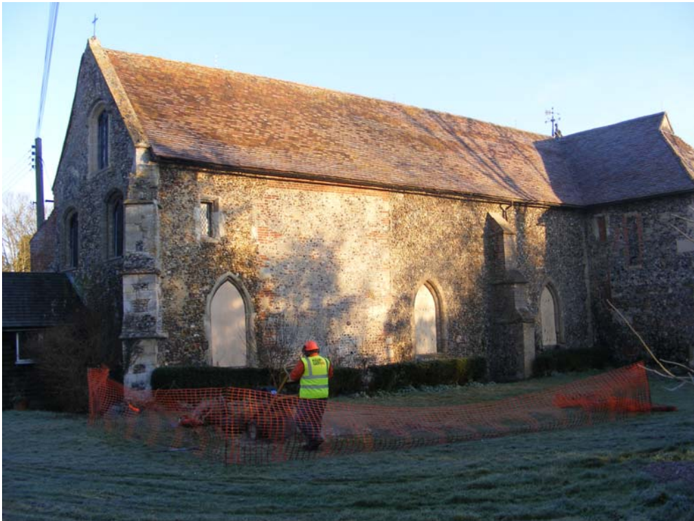
Plate 1. General view of the south side of the church prior to the start of work. The right half of the wall, including the two ground floor windows and the buttress between them, was constructed in the second half of the C19th infilling what had been an opening for full-height barn doors. The large area of paler fabric to the left of the central window is a C17th repair panel and the first and ground floor windows on the left are part of the original 14th century fabric.
