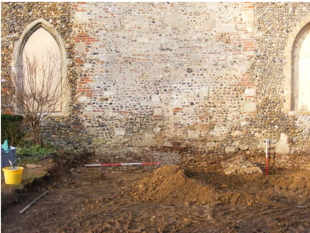
Plate 2. The below ground remains (highlighted by the scales) of a buttress (right) and chimney (left) which once projected from the face of the wall. The outer edges of the remains aligned with the limits of the repair section which was re-built after the wall containing these features was demolished. The scales are graduated in 0.5m.
