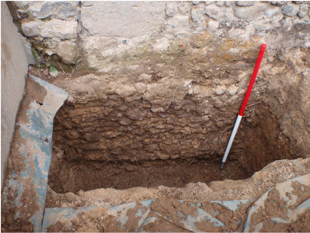
Plate 6. The medieval footing, well-constructed in bonded flint, beneath the south wall. The footing was not full length but stopped 4.5m short of the cross-wing (see below) it was built in a narrow trench, 1m deep and cut through redeposited or imported soil brought to site to raise the ground level before the infirmary was built. The top of the medieval work is at about the level of the blue plastic, the scale is 1m.
