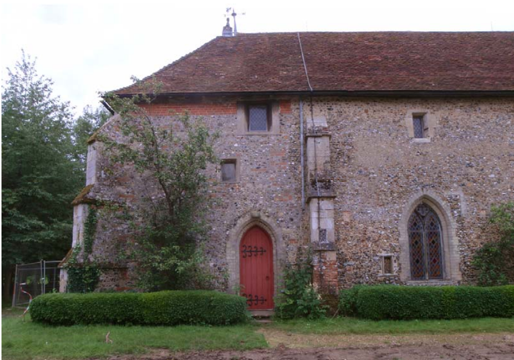
Plate 15. The east end of the church north side appears to have been re-built from a point just to the left of the buttress in the middle of the picture. Only the small first floor window on the right is the only original opening with all of the others being later inserts. The end of the footing on the opposing north face aligns with the right side of the large ground floor (C19th) window but there is no indication the building stopped here and the medieval fabric continues to the east (left) beyond this point
