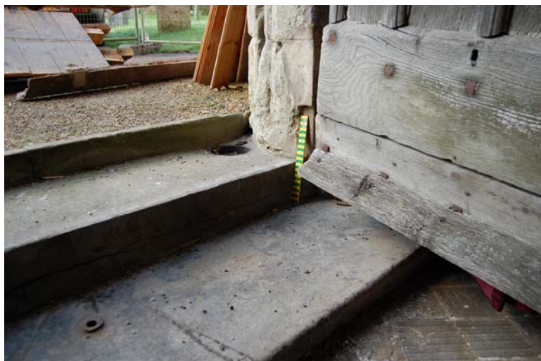
Plate 3. Steps down into the church showing the change in internal and external ground levels. The steps are later additions constructed to overcome the rising external levels.
