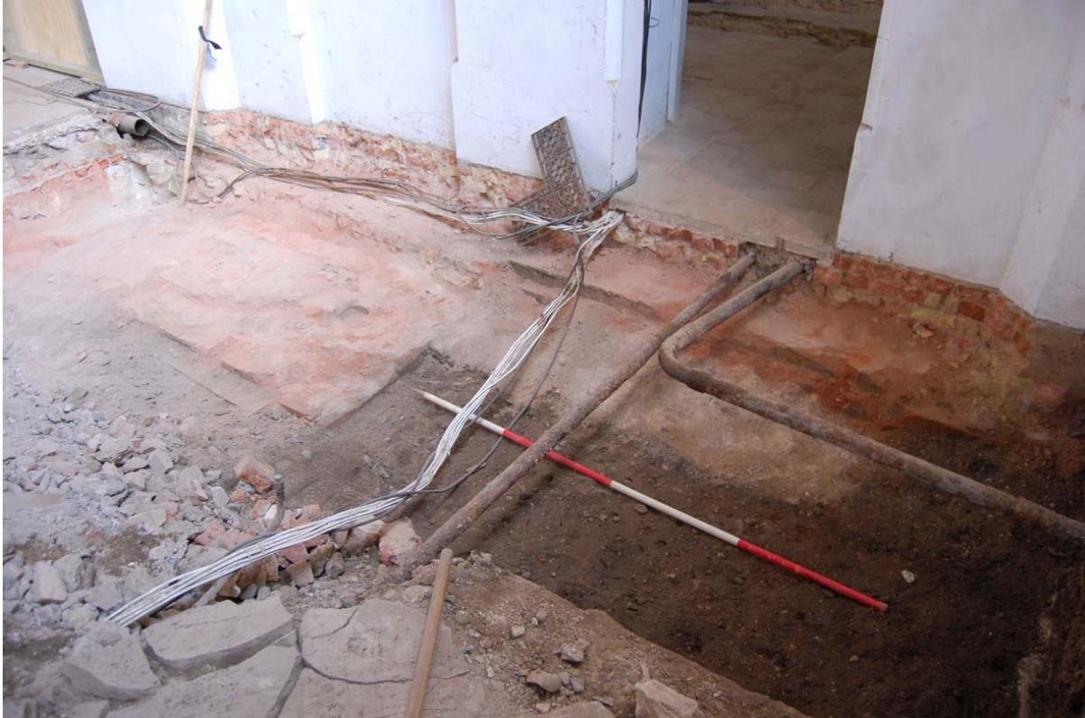
Plate 8. Brickwork (0014) underpinning the north wall of the tower. Alongside the scale is a flint footing, probably the original medieval foundation for the tower.
