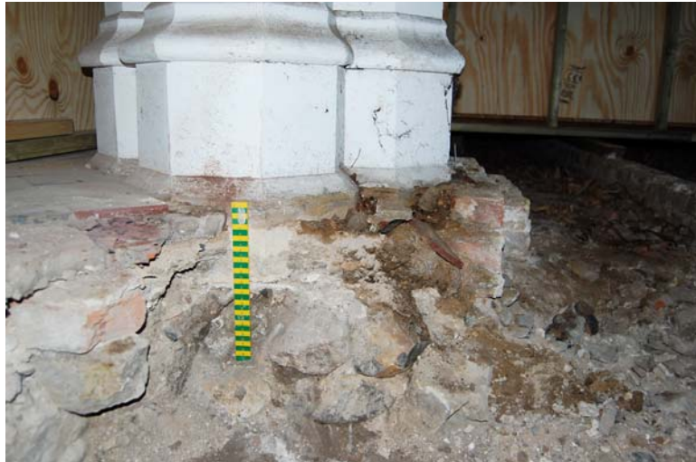
Plate 2. Flint foundation beneath the NW pier showing the absence of worked stone beneath the existing floor. The columns were built from floor level at the beginning of the C15th since when the floor levels have remain unaltered.
