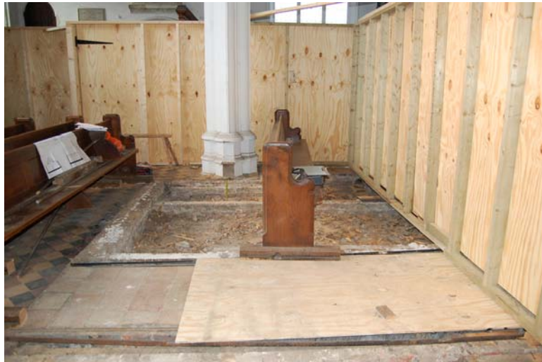
Plate 1. Area of excavation showing the dwarf walls that support the suspended floors exposed.
